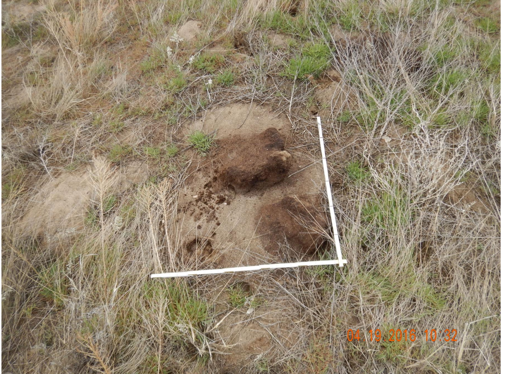
Figure 11: Photo taken from the southern end of the location (east end of the former pit location), photo shows stained soil. 3.5'x2.5' measuring stick for reference.
