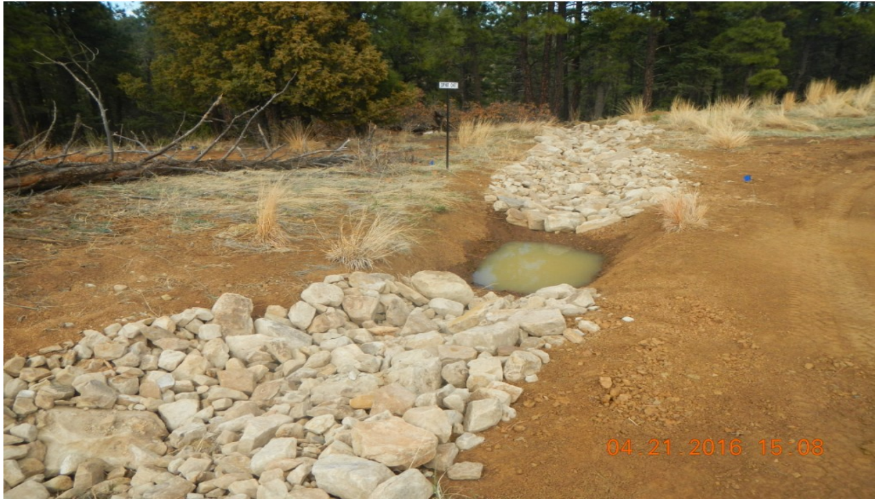
photo 3: Rip/rap rock and sediment trap has been installed at the northwest corner of the location.
