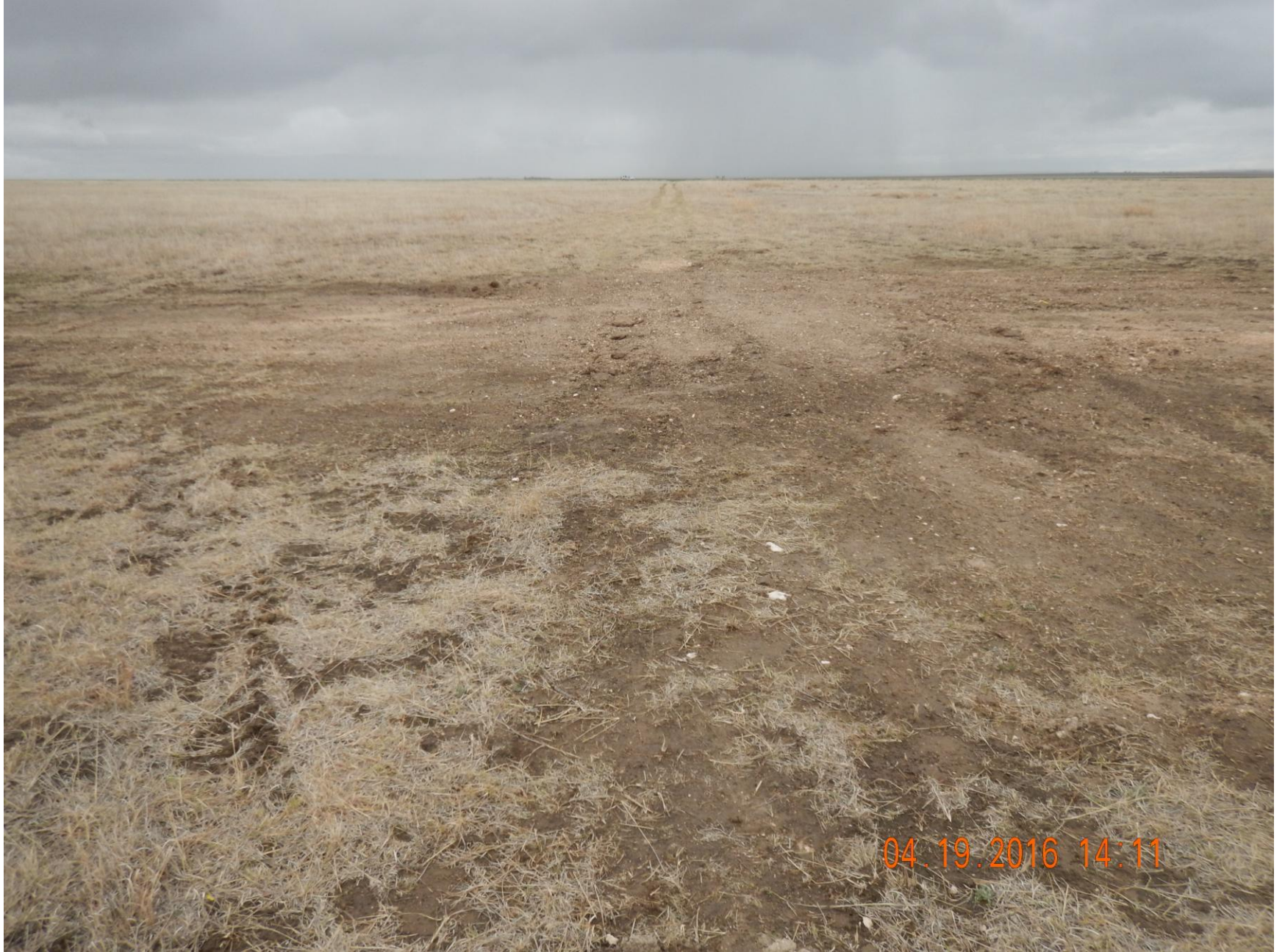
Figure 4: Photo taken from the north end of the location, facing south. Area appears to have had work done recently. Straw appears to have been spread over areas of the pit, not properly crimped. Unable to find evidence location has been seeded.
