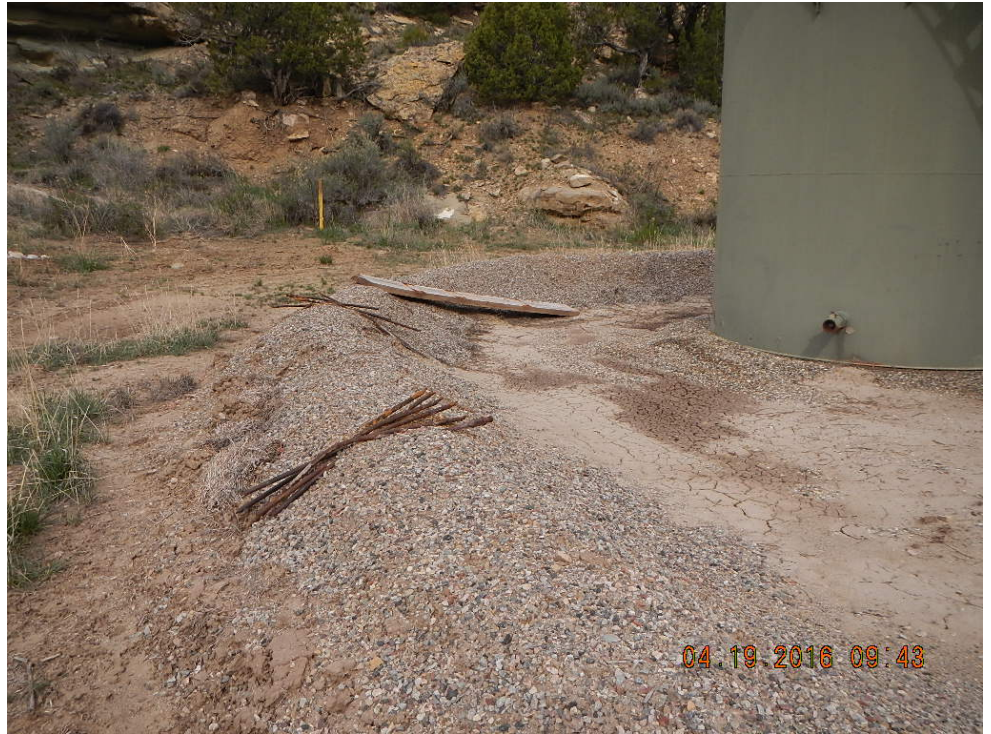
Debris on containment berm
