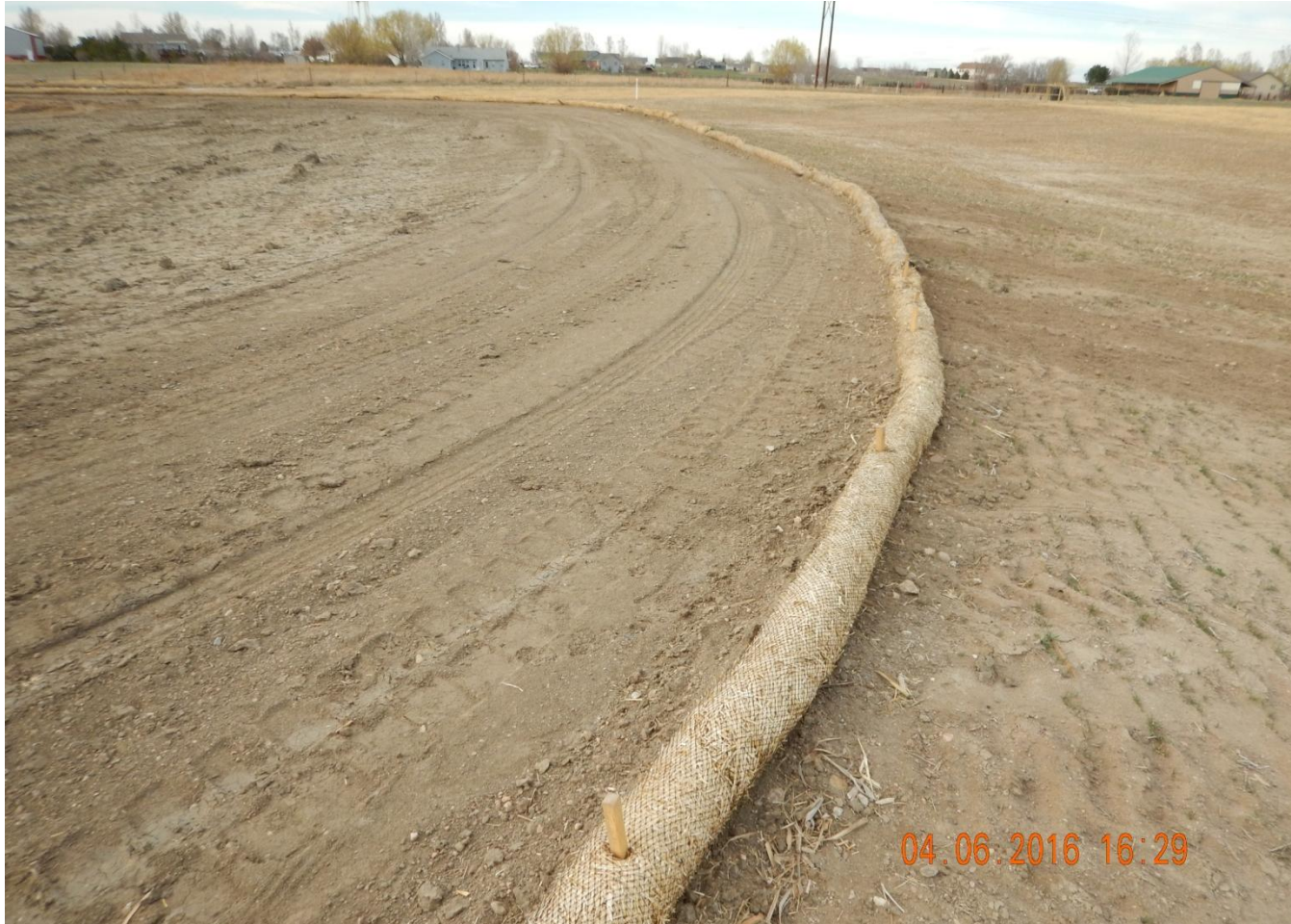
Photo 2. Photo taken from eastern location, facing North. Stormwater controls have been installed along southern, eastern and northern location areas.
