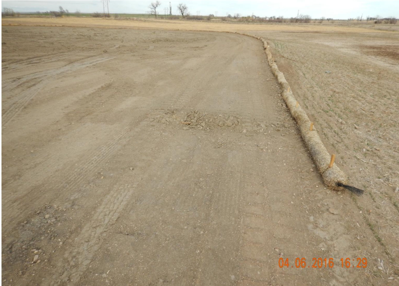
Photo 1. Photo taken from southern location, facing East. Stormwater controls have been installed along southern, eastern and northern location areas.
