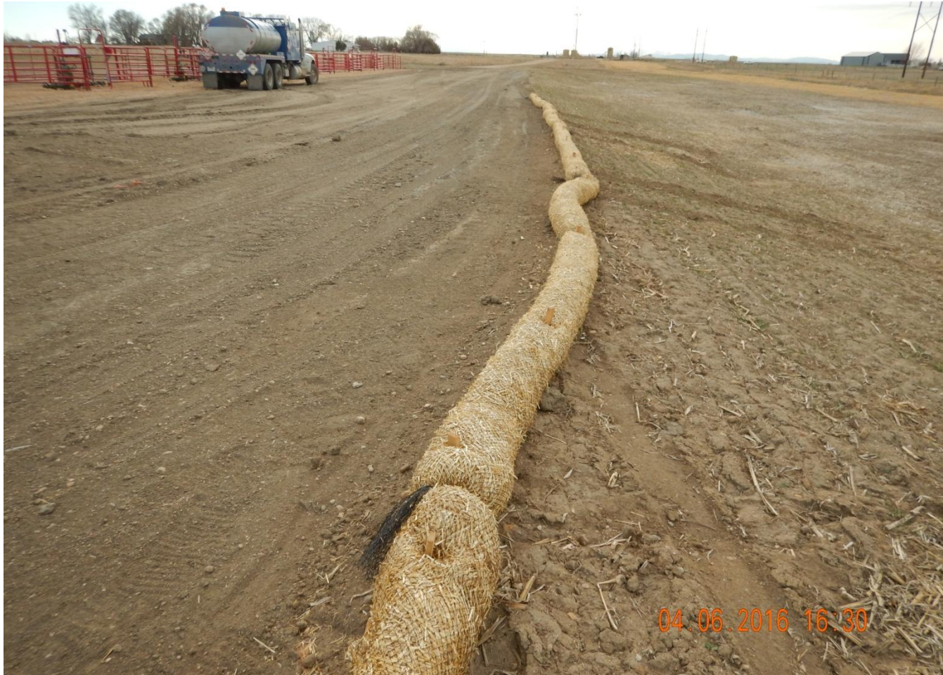
Photo 3. Photo taken from northern location, facing West. Stormwater controls have been installed along southern, eastern and northern location areas.
