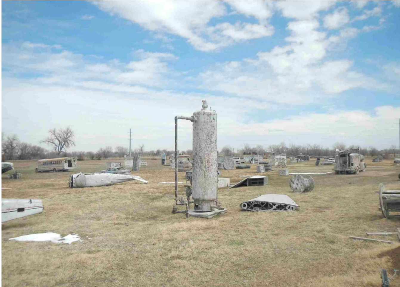
Photo 5. Photo taken of 2-phase separator, north of the 300 bbl tank. Need to remove all surface equipment within three months of plugging a well per Rule 1004.
