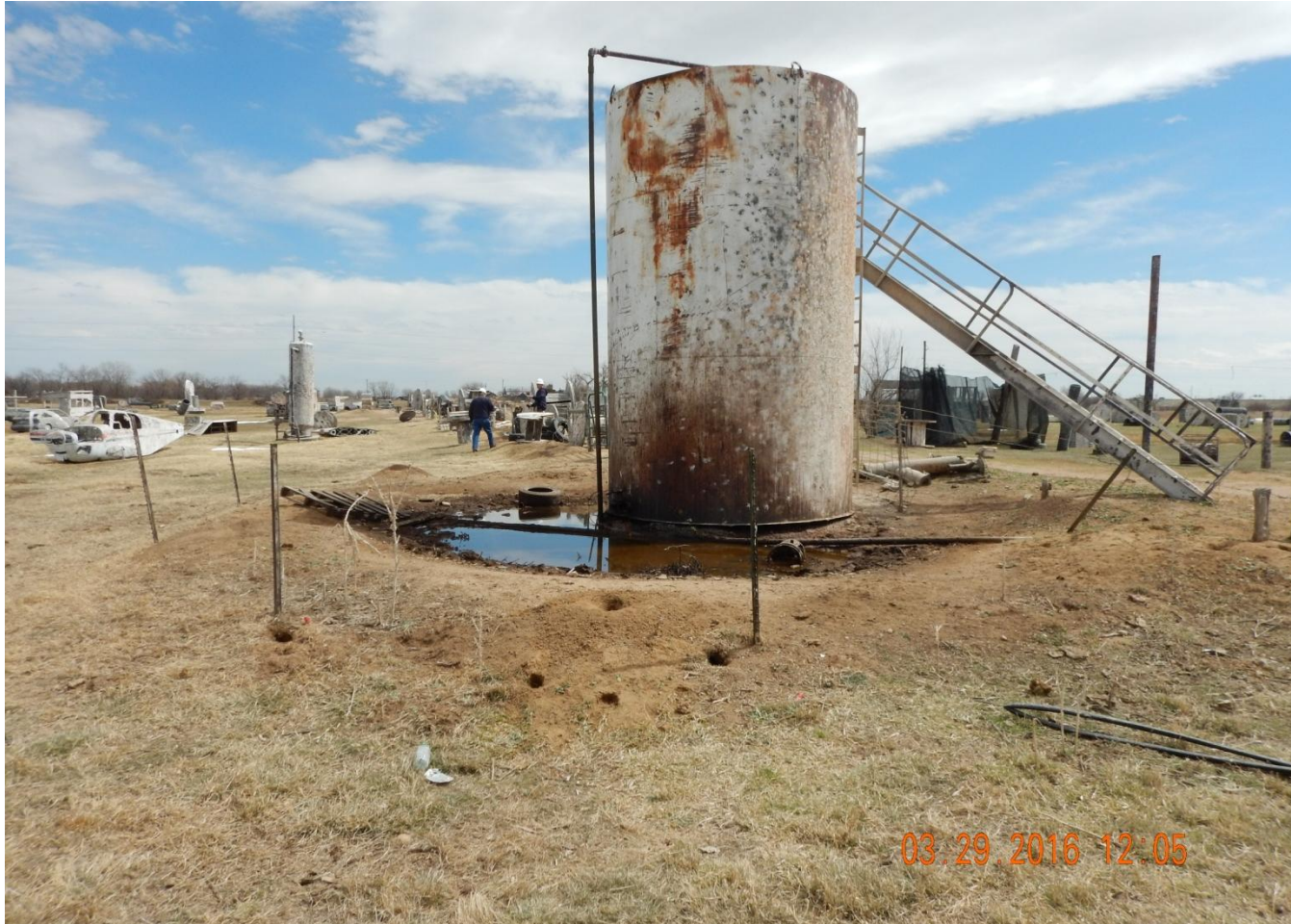
Photo 3. Photo taken of 300 bbl tank with pooled water and hydrocarbon odors. Need to remove all surface equipment within three months of plugging a well, backfill and reclaim area per Rule 1004.
