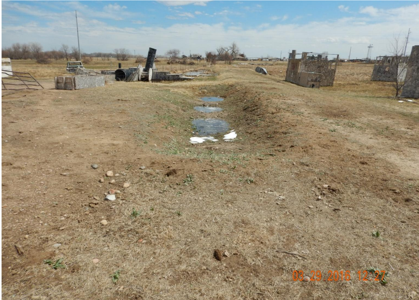
Photo 4. Photo taken east of 300 bbl tank of possible workover/plugging pit. Need to backfill and reclaim per Rule 1004.
