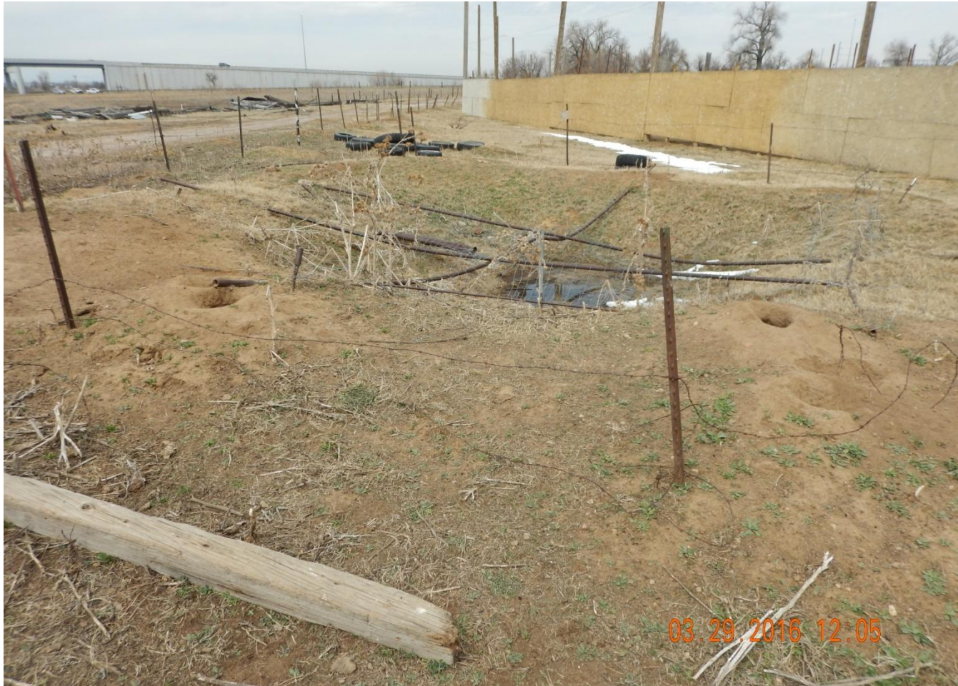
Photo 1. Photo taken of produced water pit west of 300 bbl tank. Pit needs to be backfilled and reclaimed per Rule 1004. Spread and infestation of a Colorado List B noxious weed (Bull thistle- Cirsium vulgare ) exists throughout the location, along the lease road, and spreading onto adjacent lands needs to be controlled per Rule 1004.
