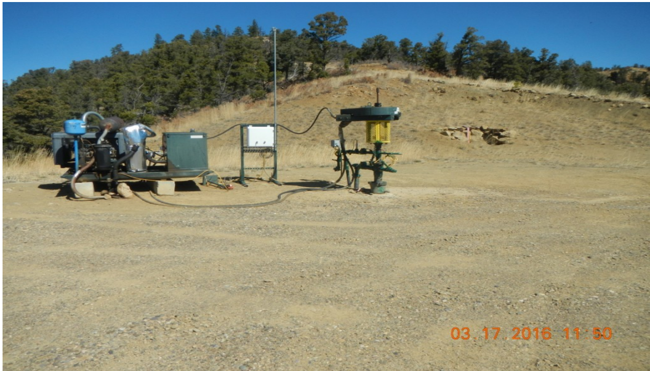
photo 1: Facing north toward the wellhead and equipment at the location.
