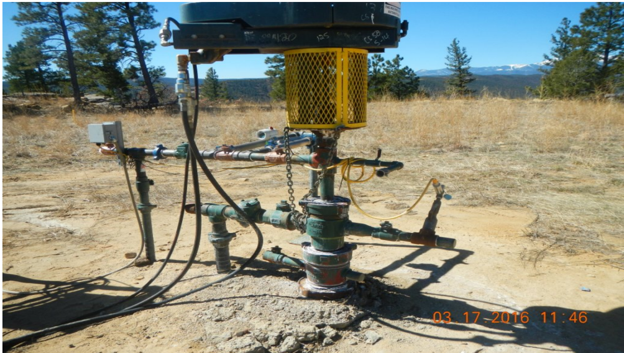
photo 3: Wellhead at the south side of the location. Water leak has been repaired.
