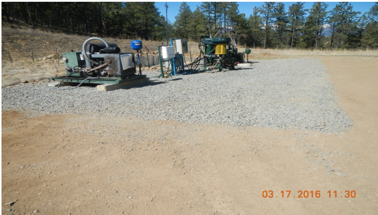
photo 2: Facing toward production equipment. New gravel has been placed around the equipment.
