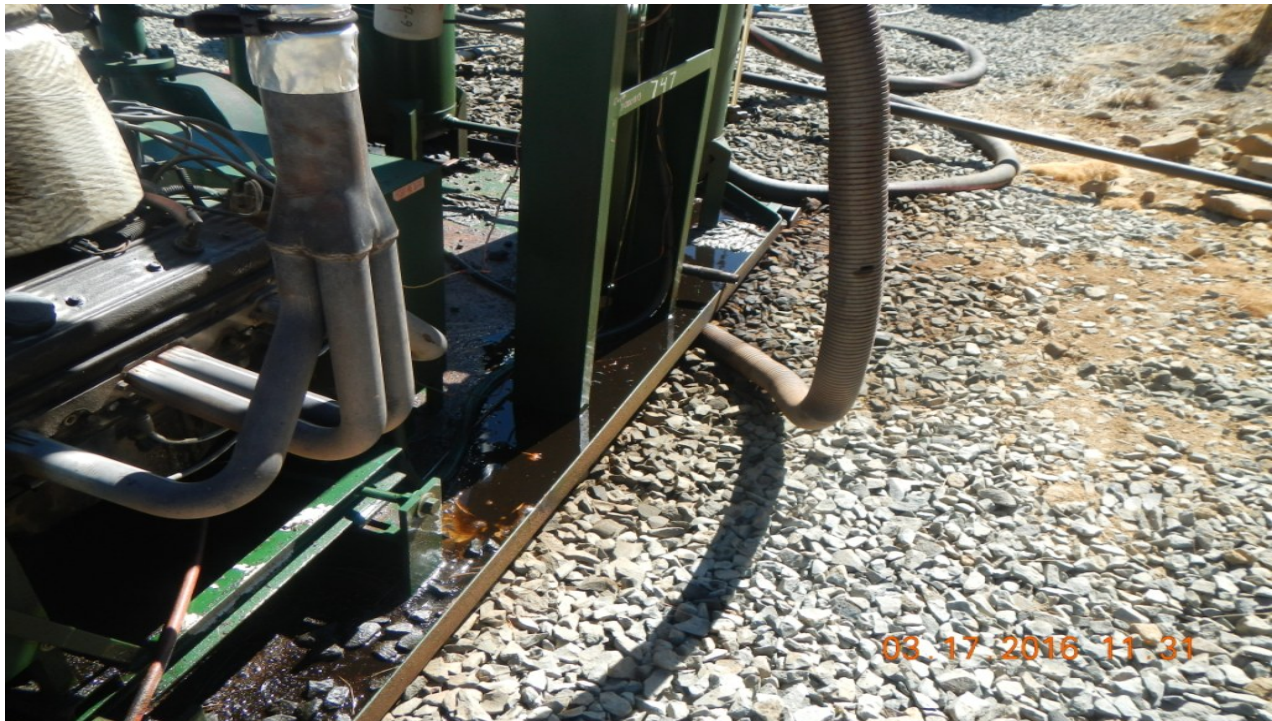
photo 3: Noticed oil on the skid of the separator. Pioneer employee nearby was notified.
