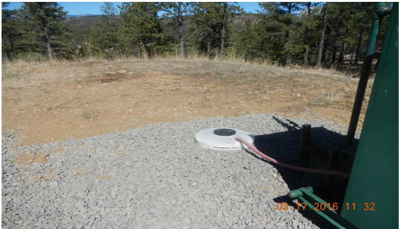
photo 6: Facing toward the northwest corner. Oil fluid noticed in the previous inspection appears to have been cleaned up.
