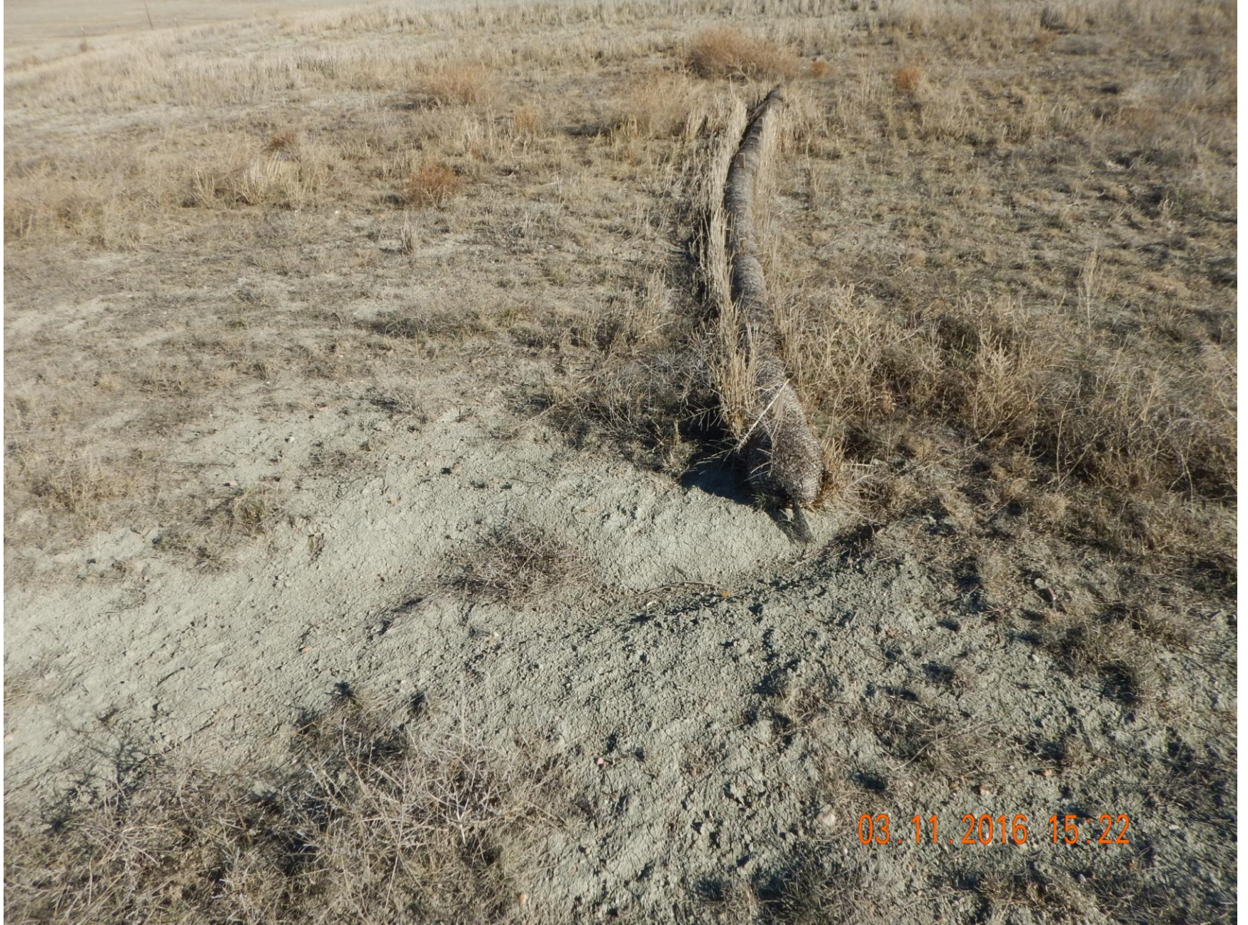
Figure 8: Photo taken from the west end of the location, facing east. Photo shows straw wattle BMP improperly maintained. Wattle is accelerating stormwater around, rather than pooling, causing erosion.
