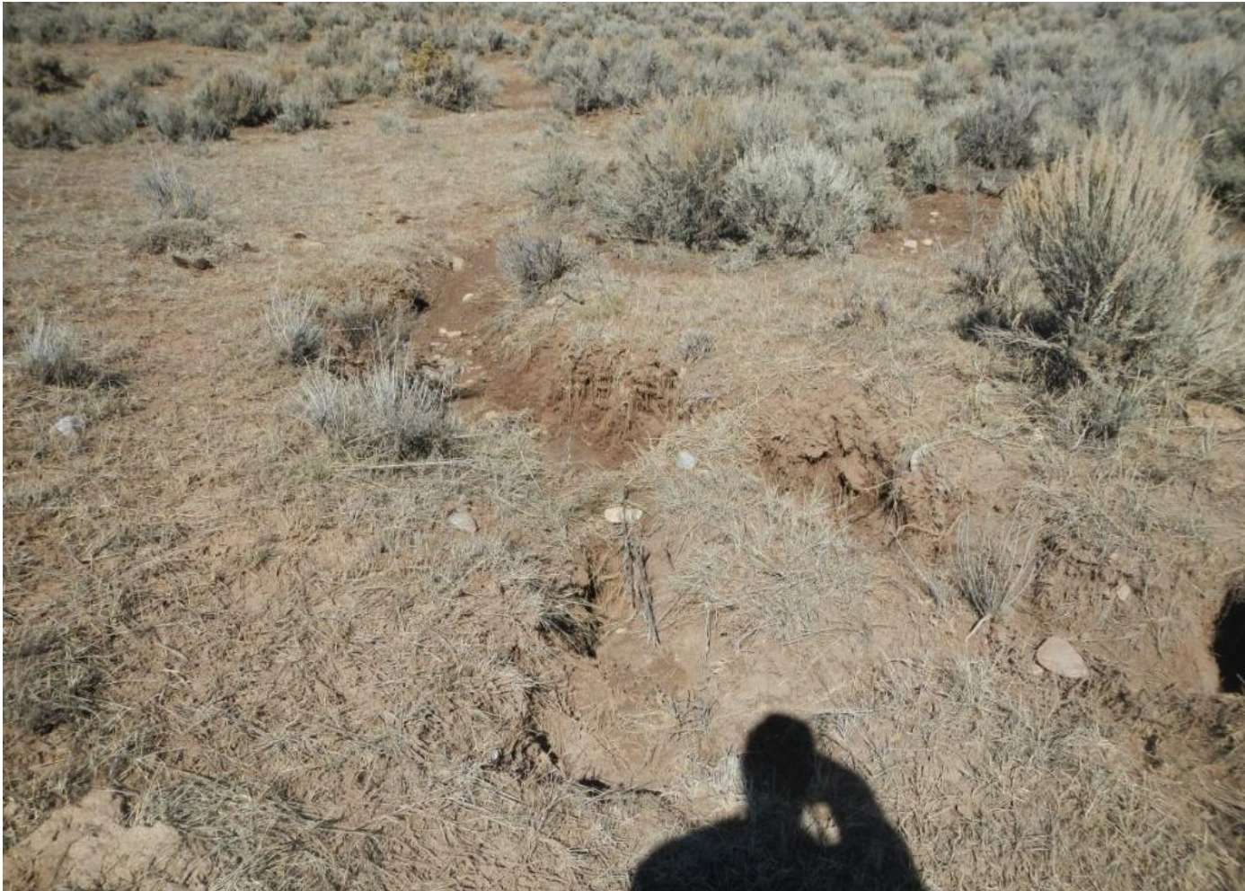
Photo 1. View of erosion channel that is approximately 3 feet wide and deep in the northeastern portion of the project area. This channel needs to be stabilized.
