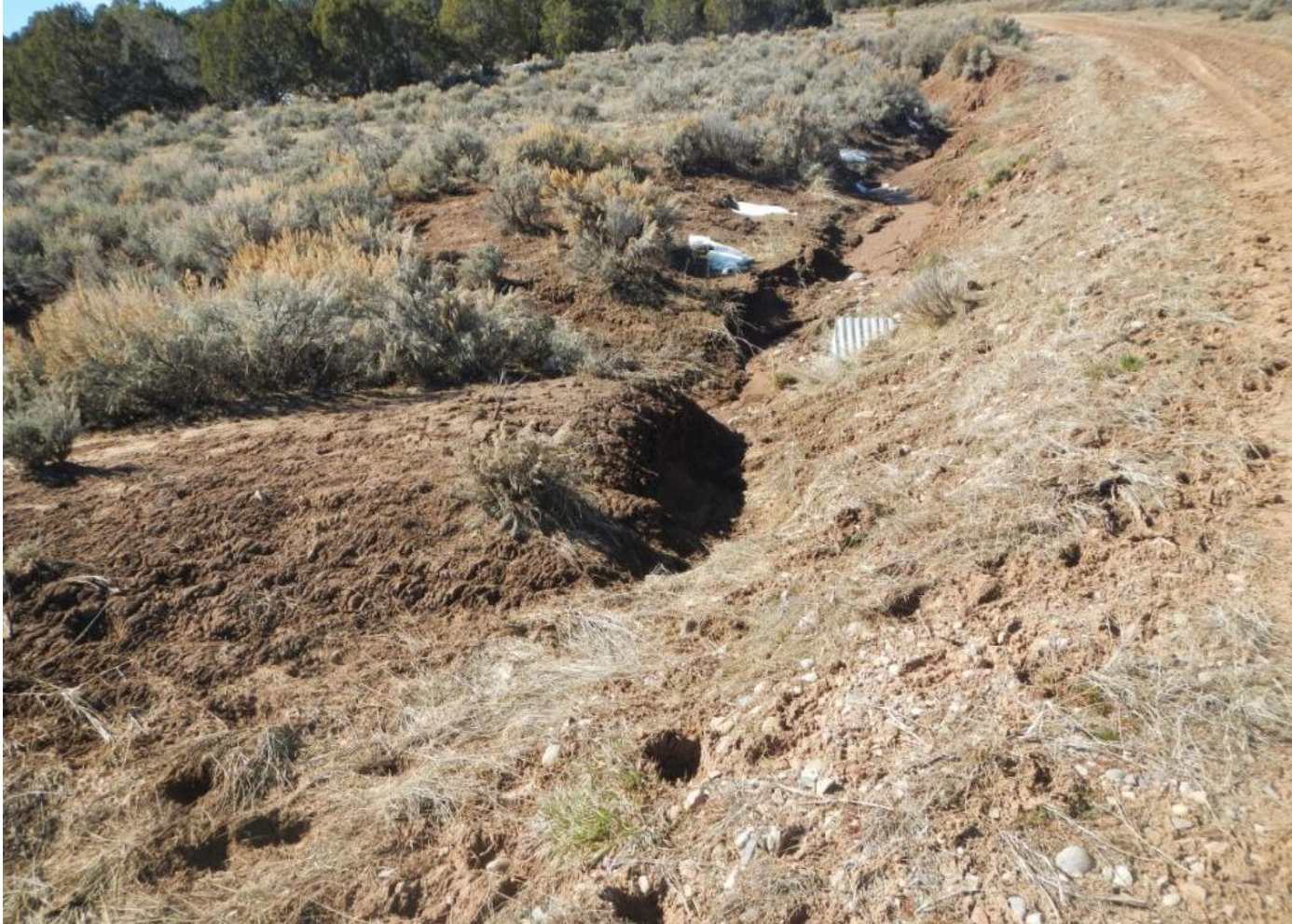
Photo 2. View of area near well pad entrance where stormwater flows off of the project area toward a culvert. Stormwater BMPs need to be installed here to prevent erosion and sediment discharge.
