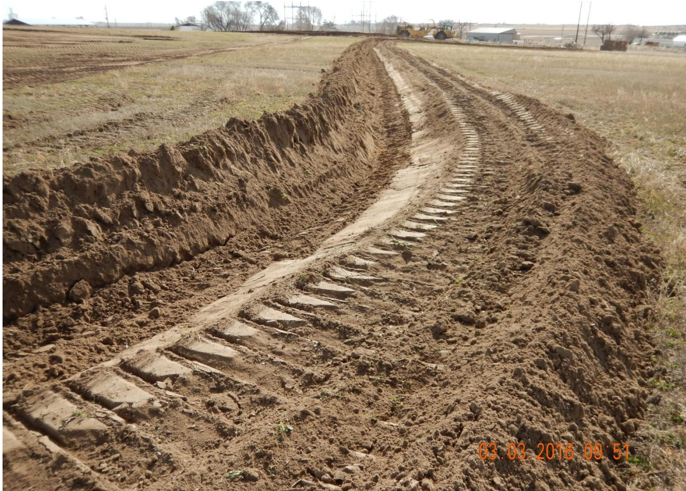
Photo 5. Photo taken from western location, facing East. Stormwater and sediment control BMPs installed in center of photo.
