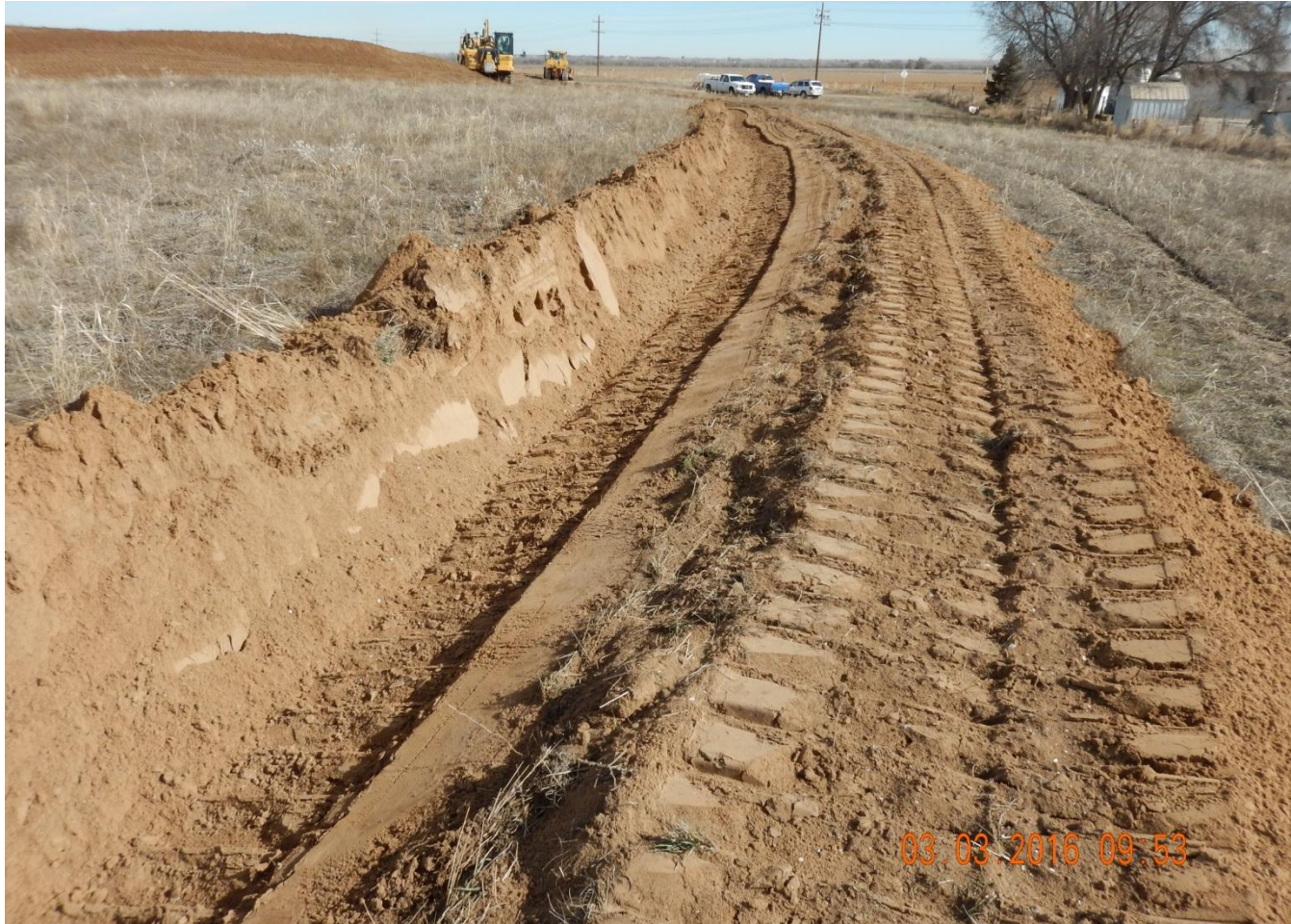
Photo 8. Photo taken from southern location, facing Northeast. Stormwater and sediment control BMPs installed in center of photo.
