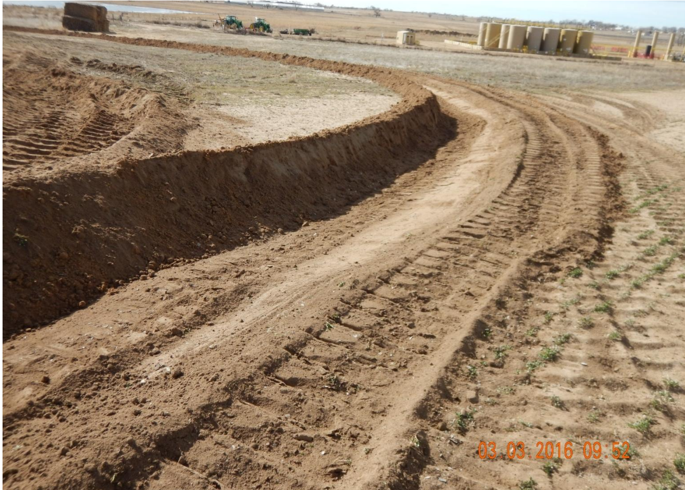
Photo 6. Photo taken from southwest location, facing South. Stormwater and sediment control BMPs installed in center of photo.
