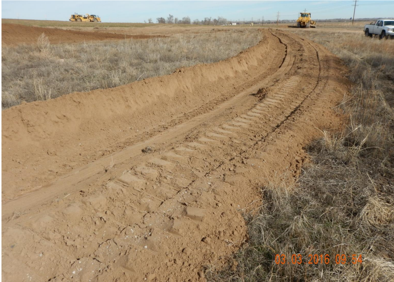
Photo 9. Photo taken from southeast location, facing North. Stormwater and sediment control BMPs installed in center of photo.
