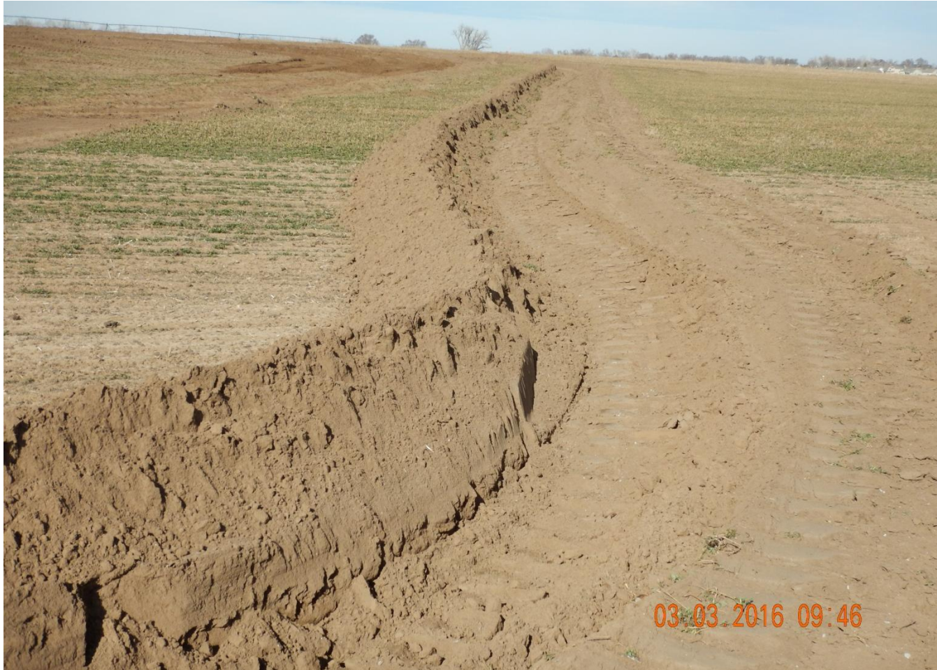
Photo 1. Photo taken from eastern location, facing North. Stormwater and sediment control BMPs installed in center of photo.
