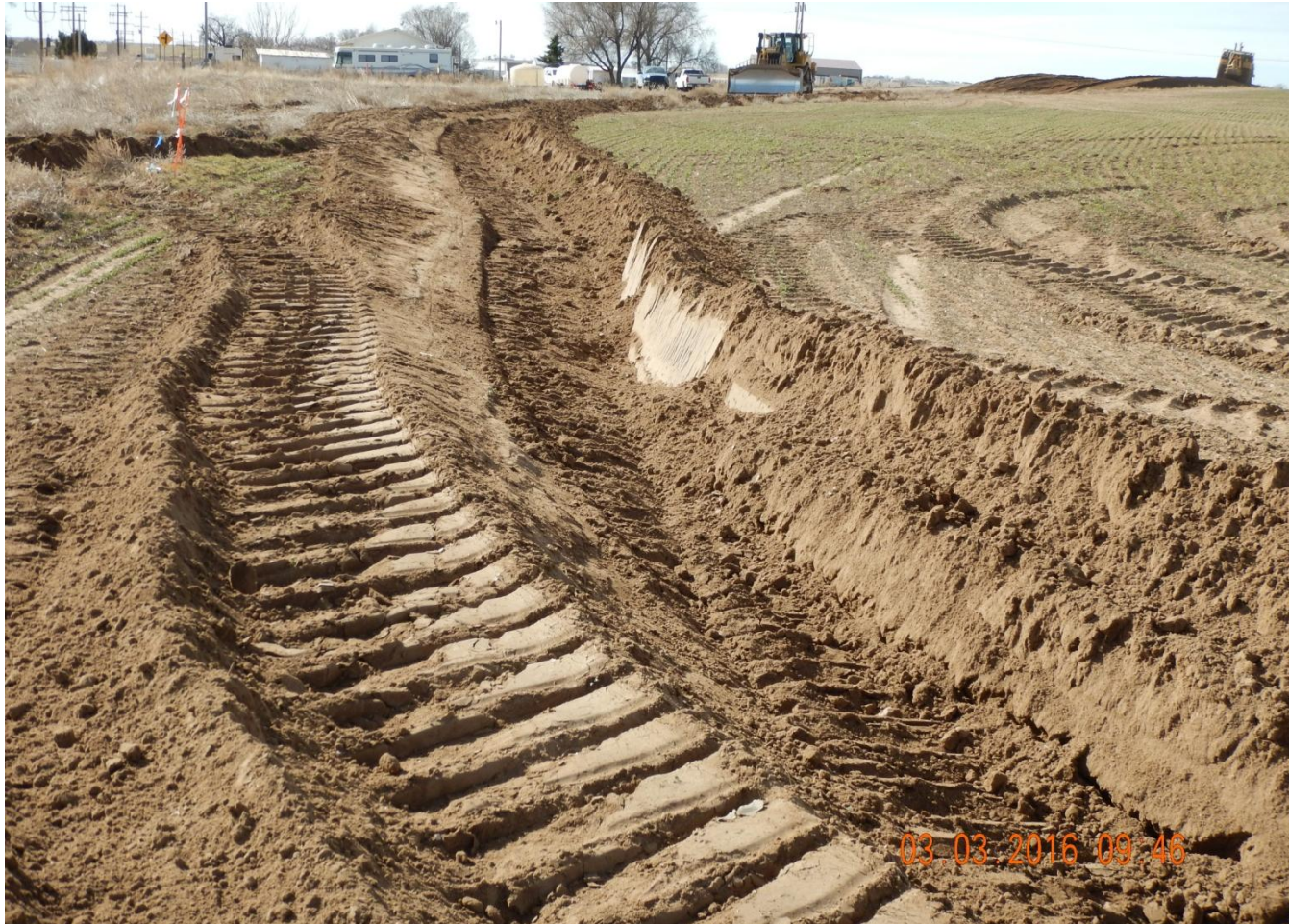
Photo 2. Photo taken from eastern location, facing South. Stormwater and sediment control BMPs installed in center of photo.
