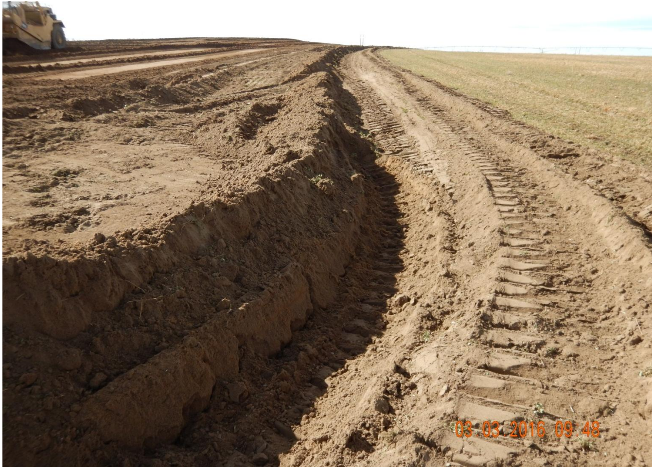
Photo 3. Photo taken from northeast location, facing West. Stormwater and sediment control BMPs installed in center of photo.
