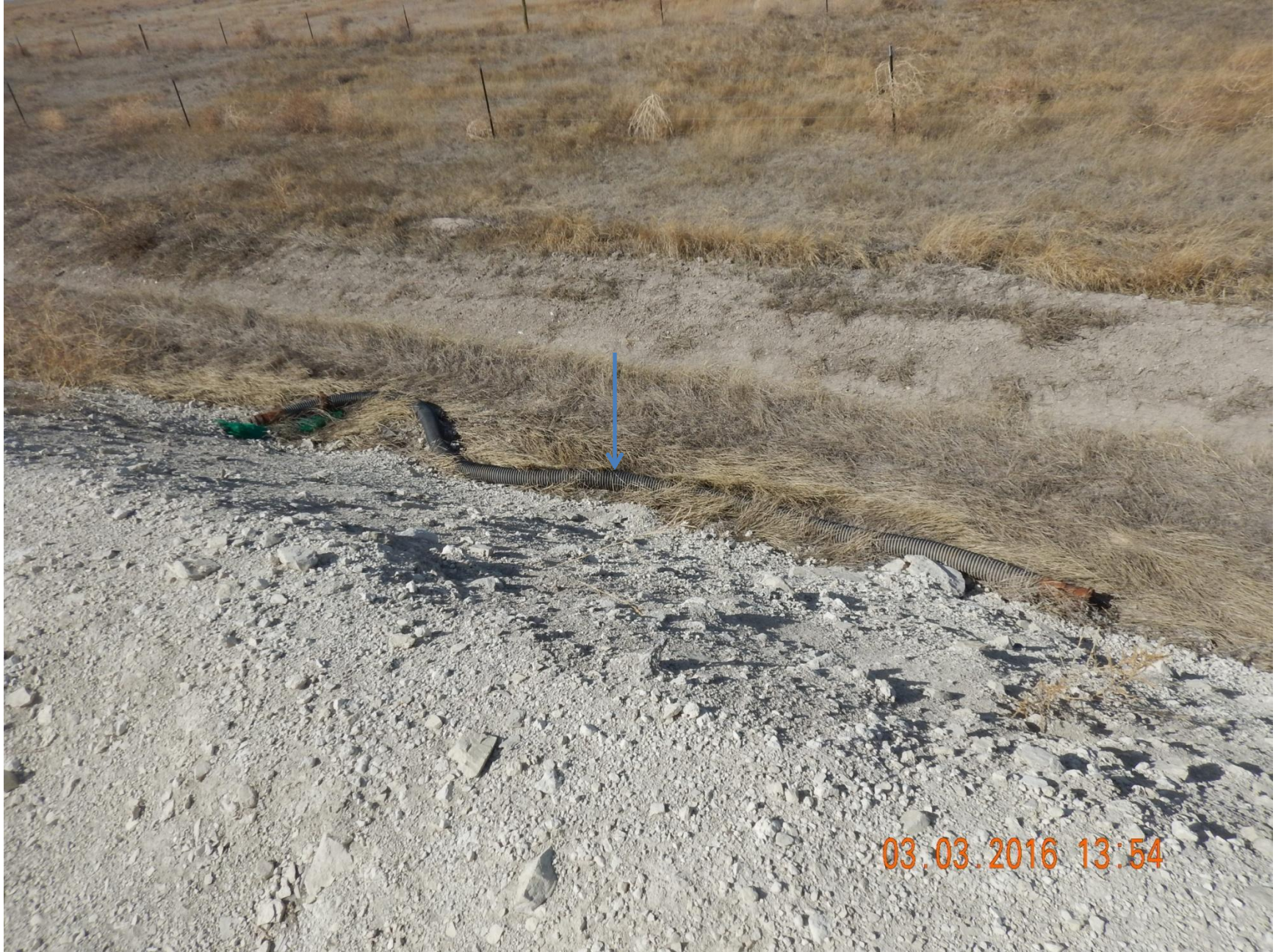
Figure 23: Photo taken from the north end of the project area, facing north. Photo of what appears to be ~15-20 feet of tubing equipment in the interim area.
