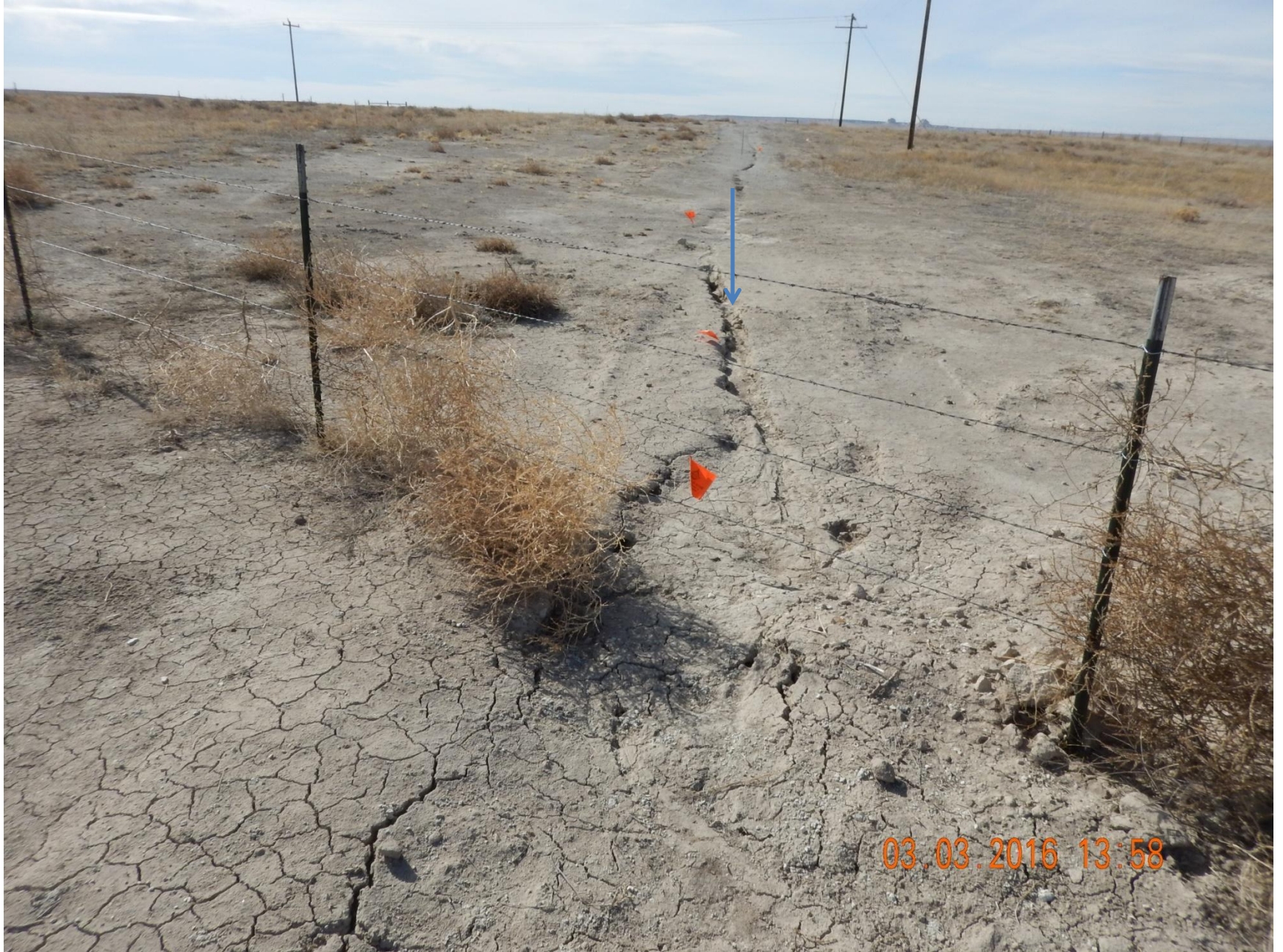
Figure 28: Photo taken from northwest corner of the location, facing west. Photo of pipeline. Photo shows stormwater erosion occurring onto pipeline flowing onto project location and into diversion ditch.
