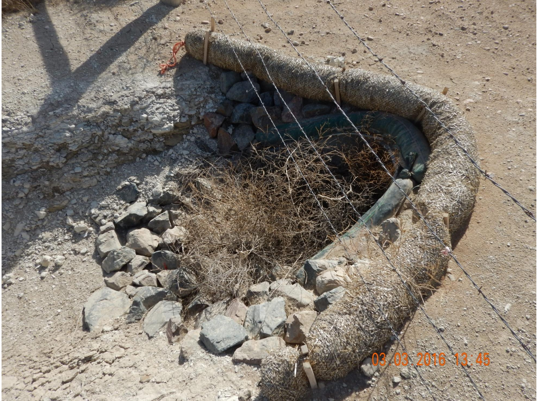
Figure 10: Photo taken from the access road at the south end of the location. Photo of culvert and stormwater and sediment control BMPs
