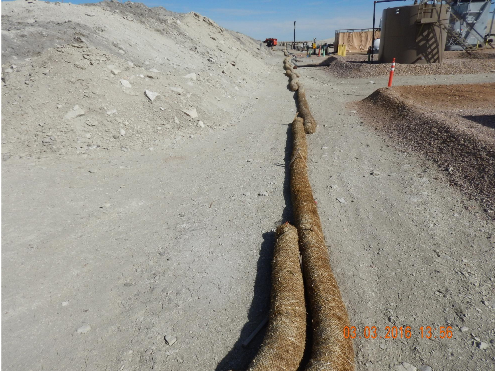
Figure 25: Photo taken from the northern end of the project area, west of the drill cuttings, facing east. Photo shows straw wattles used as a stormwater and sediment control BMP around cuttings
