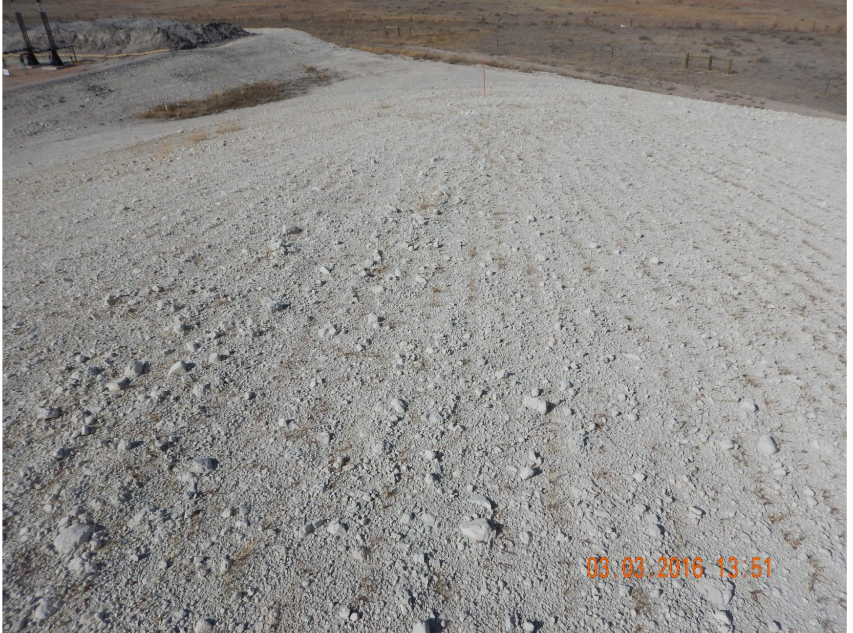
Figure 19: Photo taken from the spoils stockpile berm on the east end of the location, facing north. Photo shows soils on berm, and interim area.
