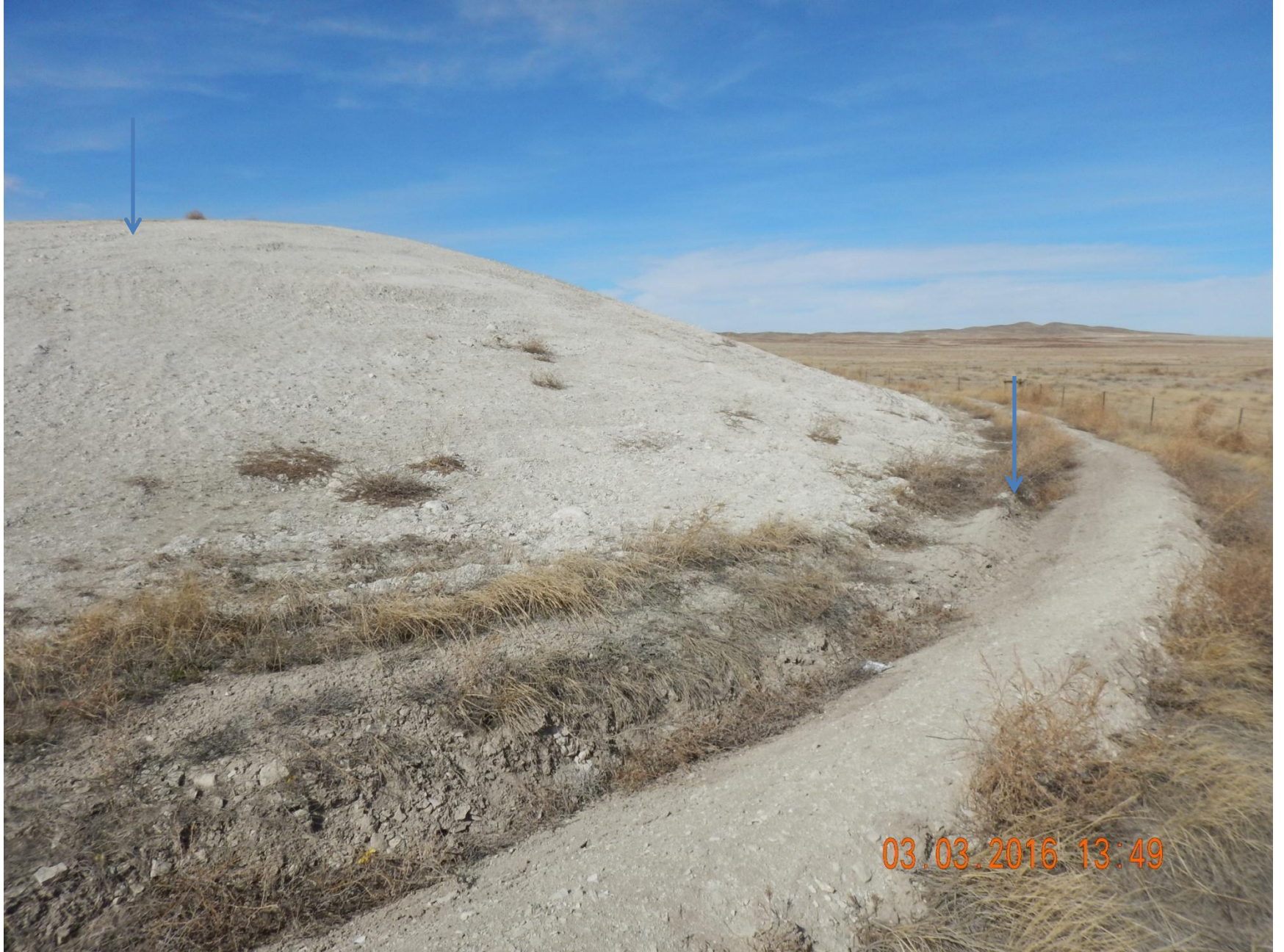
Figure 15: Photo taken from the southeast corner of the interim area facing northeast. Photo shows stormwater diversion ditch, and spoils stockpile berm.
