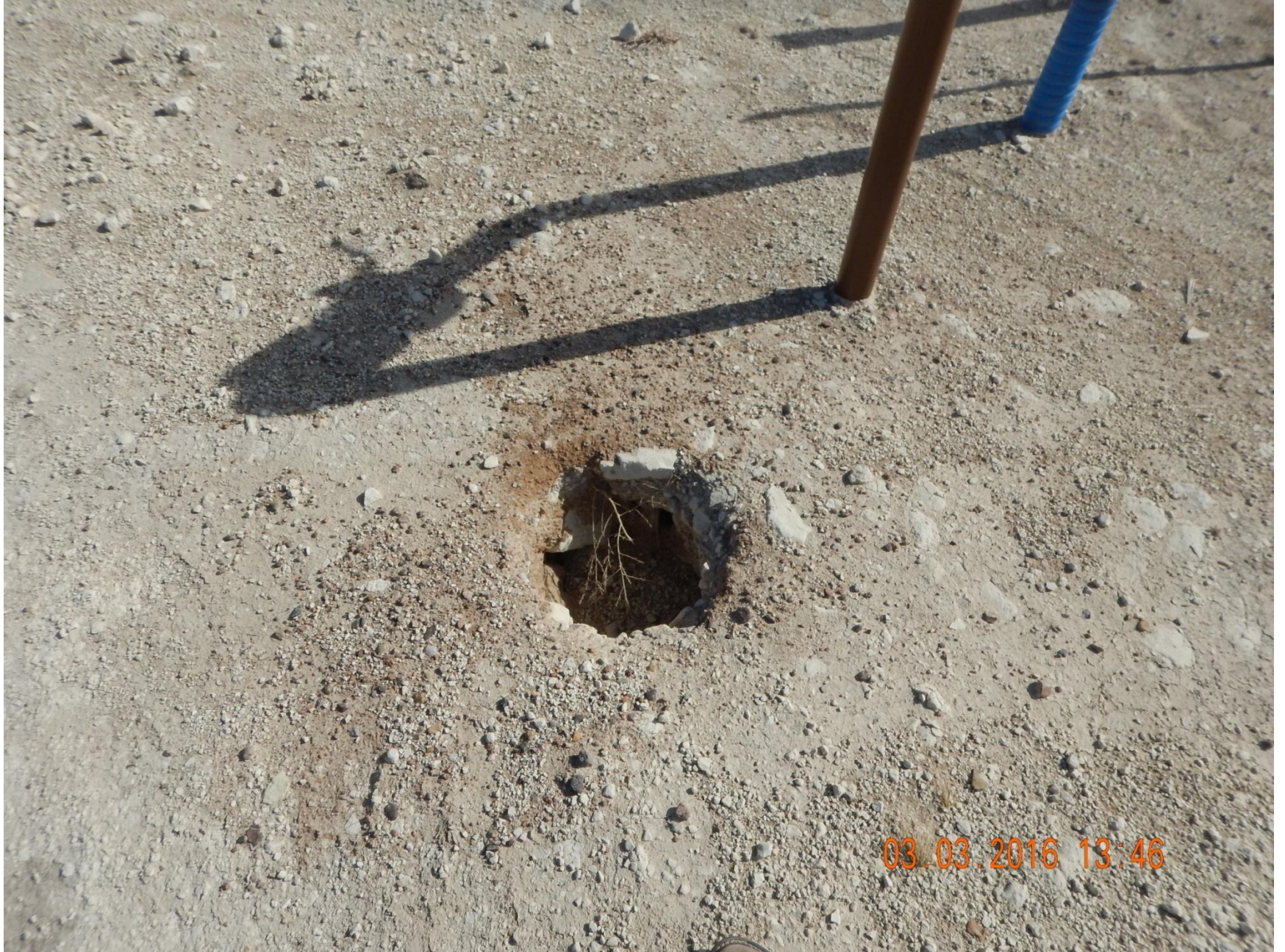
Figure 12: Photo taken from pipe adjacent to the access road on the south end of the location. Photo of exposed hole due to either subsidence or wildlife.
