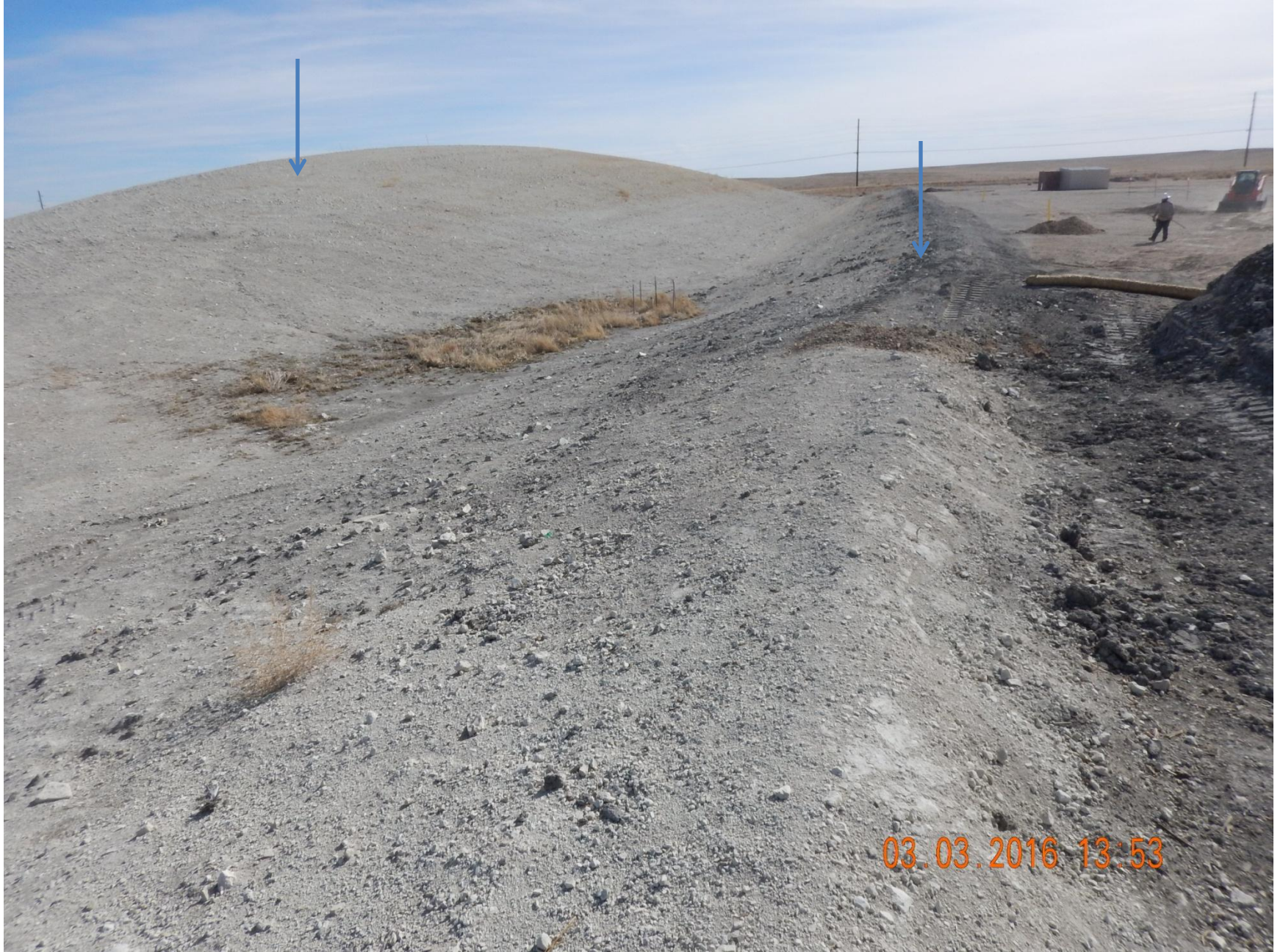
Figure 21: Photo taken from the northeast corner of the project area, facing west. Photo shows spoils stockpile to the left, and containment berm on the east perimeter of the project area.
