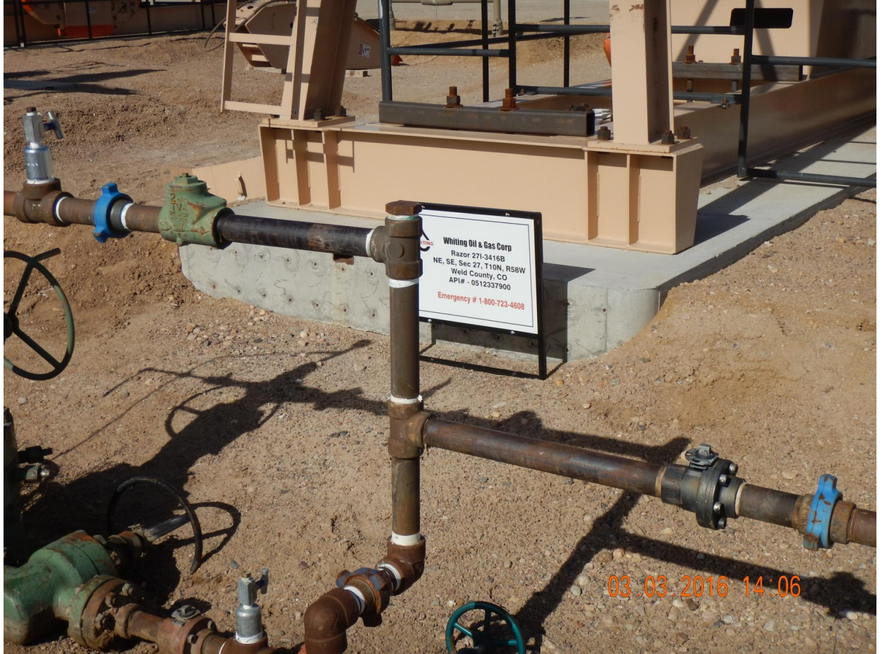
Figure 6: Photo of well #123-37900
