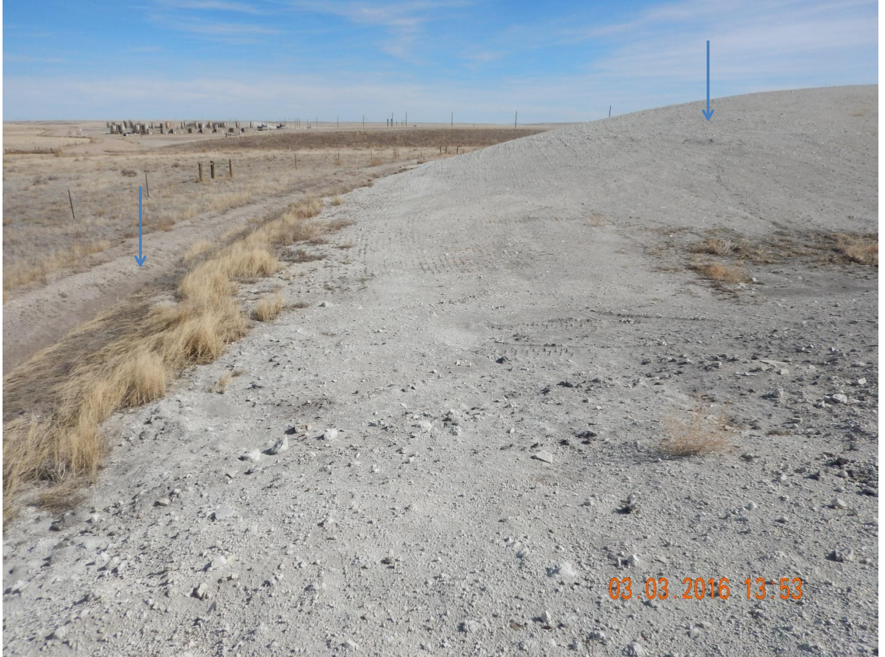
Figure 22: Photo taken from the northeast corner of the project area, facing east. Photo shows spoils stockpile on the right of the photo, and the stormwater diversion ditch on the left. .
