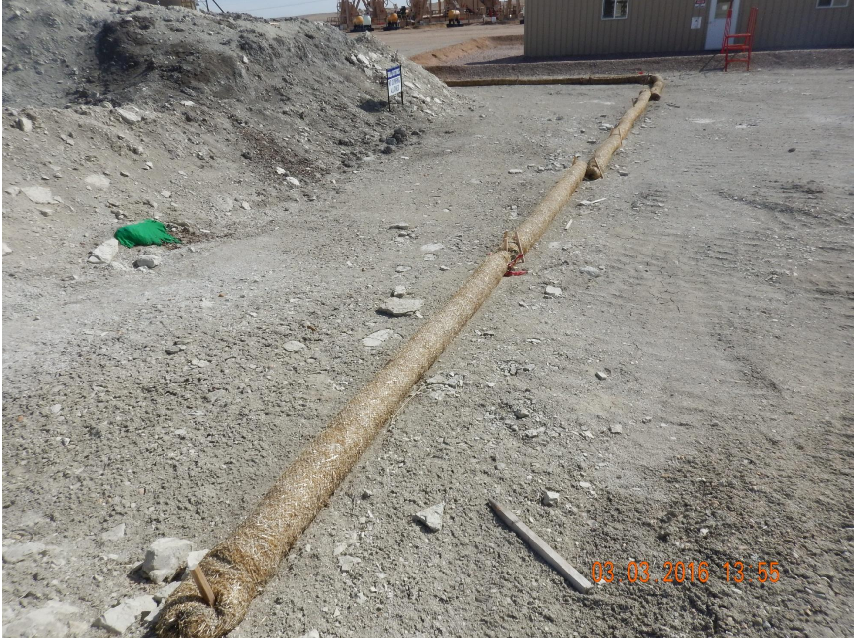
Figure 24: Photo taken from the northern end of the project area, west of the drill cuttings, facing south. Photo shows straw wattles used as a stormwater and sediment control BMP around cuttings.
