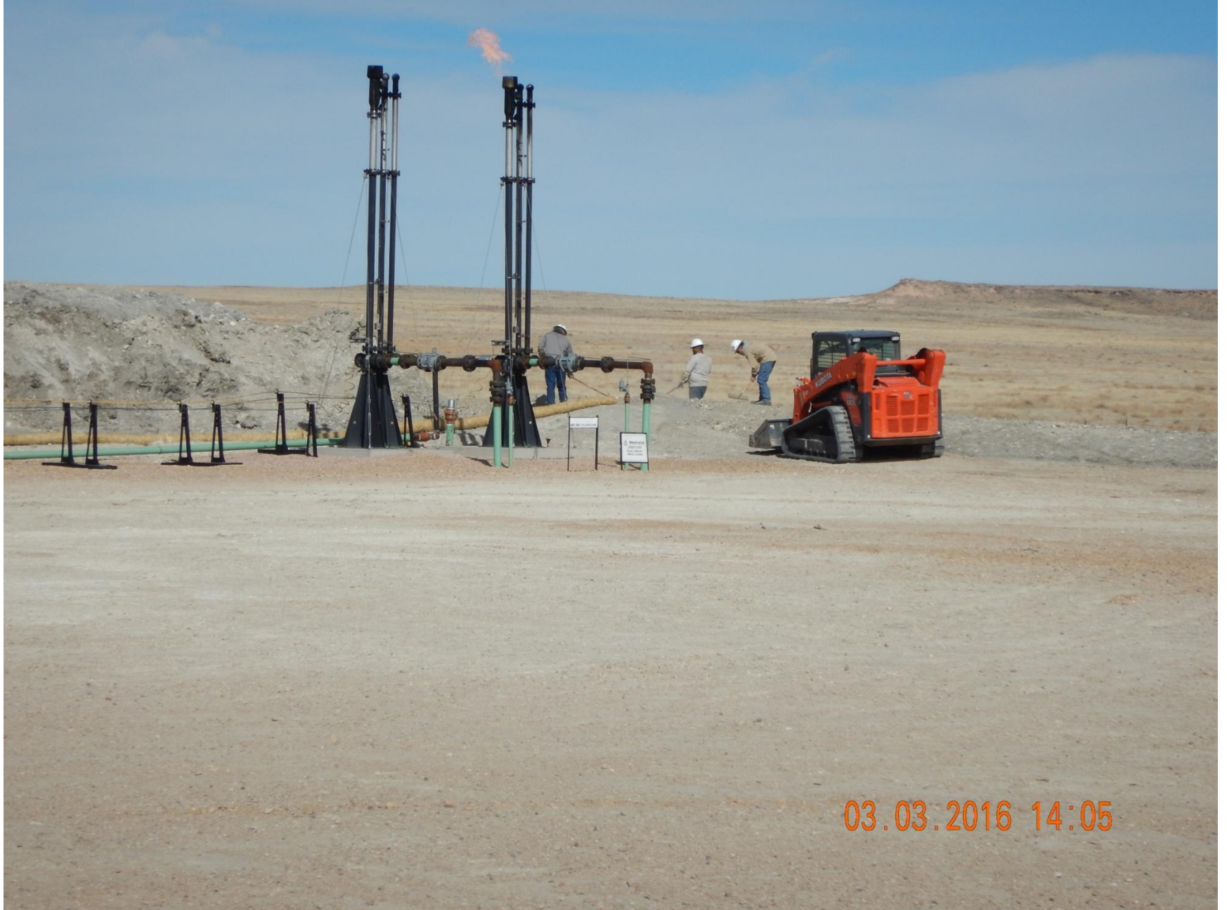
Figure 32: Photo taken from the center of the location, facing northeast. Photo shows workers repairing stormwater control BMPs.
