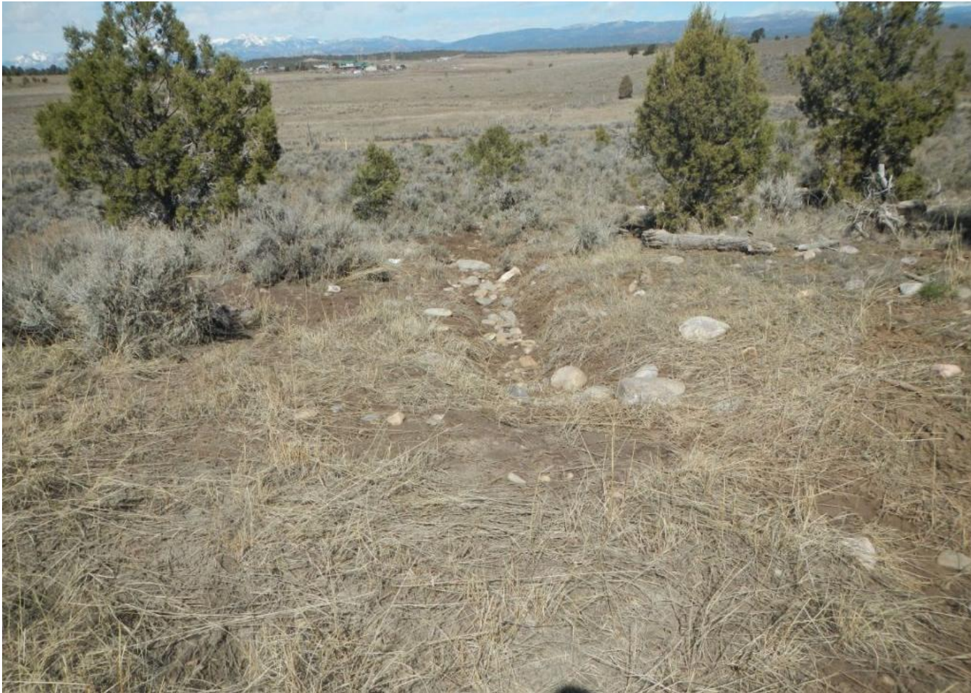
Photo 8. View of stormwater erosion downstream from Photo 7, where stormwater flows are eroding a channel northeast of the project area. Channel is approximately 2 feet wide and 1 foot deep.
