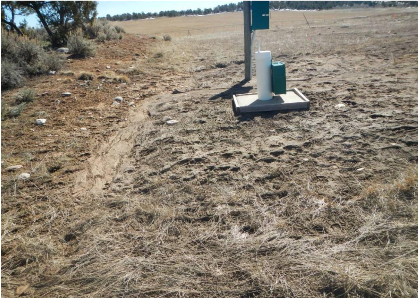
Photo 7. View of area in the northeastern corner of the project area where stormwater flows off of the well pad and is eroding the slope northeast of the project area, shown in Photo 8.
