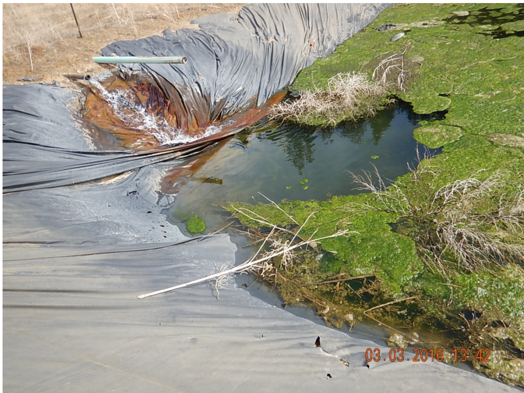
Figure 2 – Water intake on northwest corner of pit. Liner is torn above water level.
