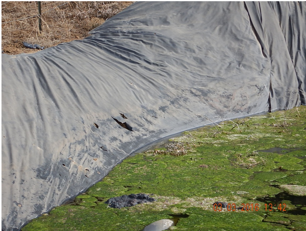
Figure 3 – Torn liner on northeast pit wall.
