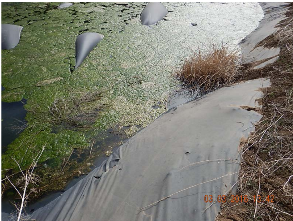
Figure 4 – Torn liner on northwest pit wall.
