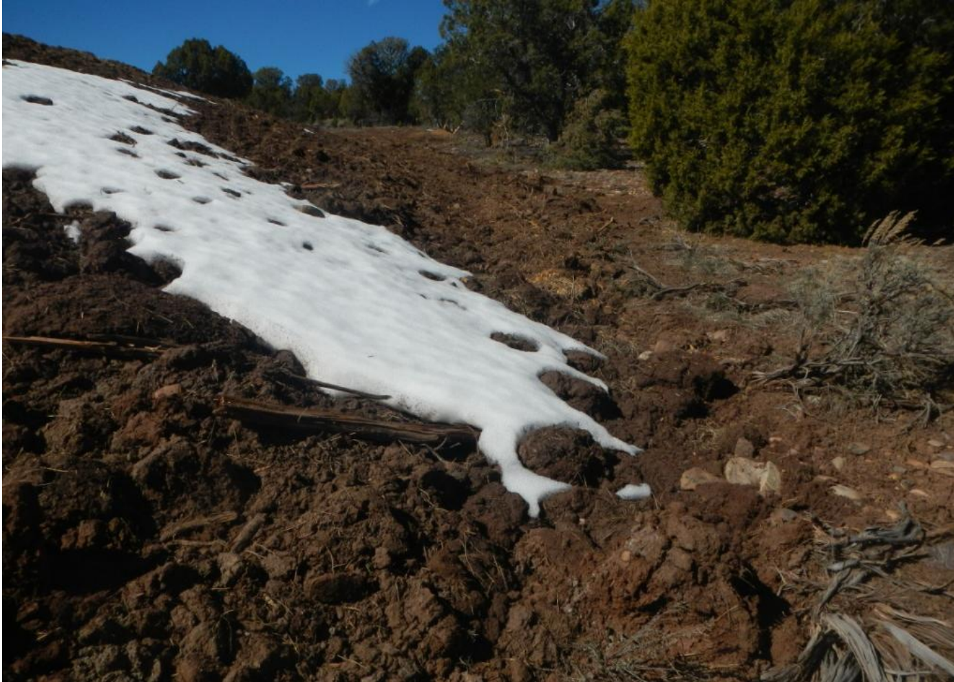
Photo 6. View of the topsoil stockpile in the northeastern corner of the project area. Topsoil stockpile is not stabilized as no BMPs to filter snowmelt or stormwater runoff have been applied.
