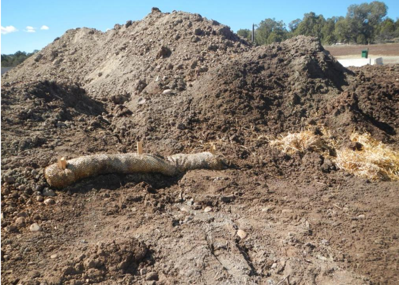
Photo 7. View of one of only two straw wattles in the project area. Wattle is in disrepair and does not appear to be functioning properly.
