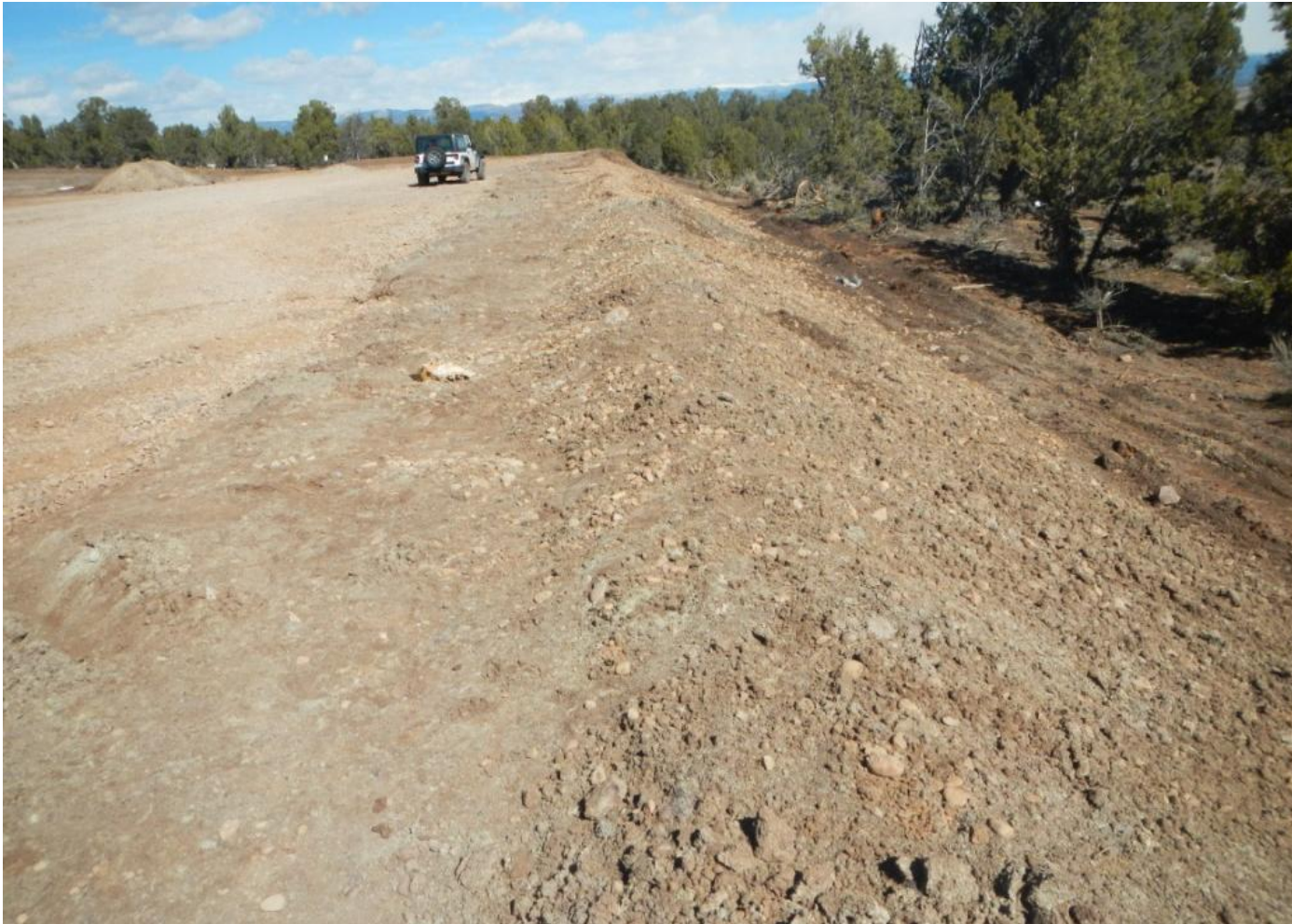
Photo 5. View of the eastern edge of the project area from the southeastern corner facing northward. Fill slopes are not stabilized and need additional stabilization measures.
