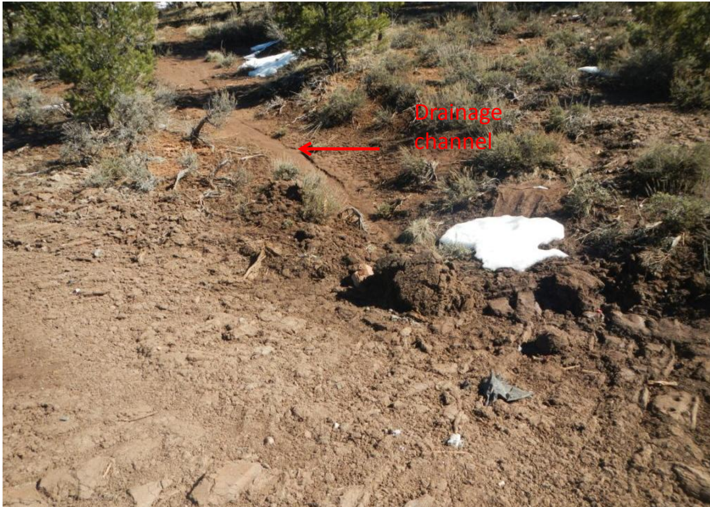
Photo 3. View of a drainage channel that was filled during construction in the eastern portion of the project area. No stormwater BMPs are present on the fill slopes in the foreground to prevent runoff into the channel.
