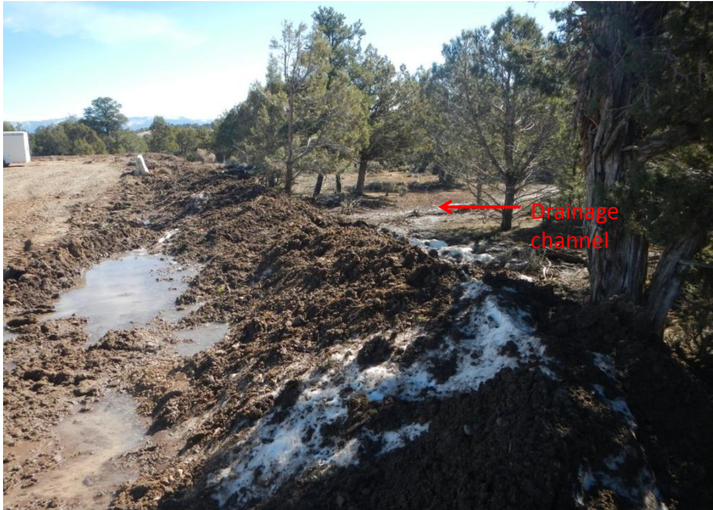
Photo 4. View of a drainage channel that was filled during construction in the southern portion of the project area from the southwestern corner facing eastward. No stormwater BMPs are present on the fill slopes to prevent runoff into the channel or along the southern edge.
