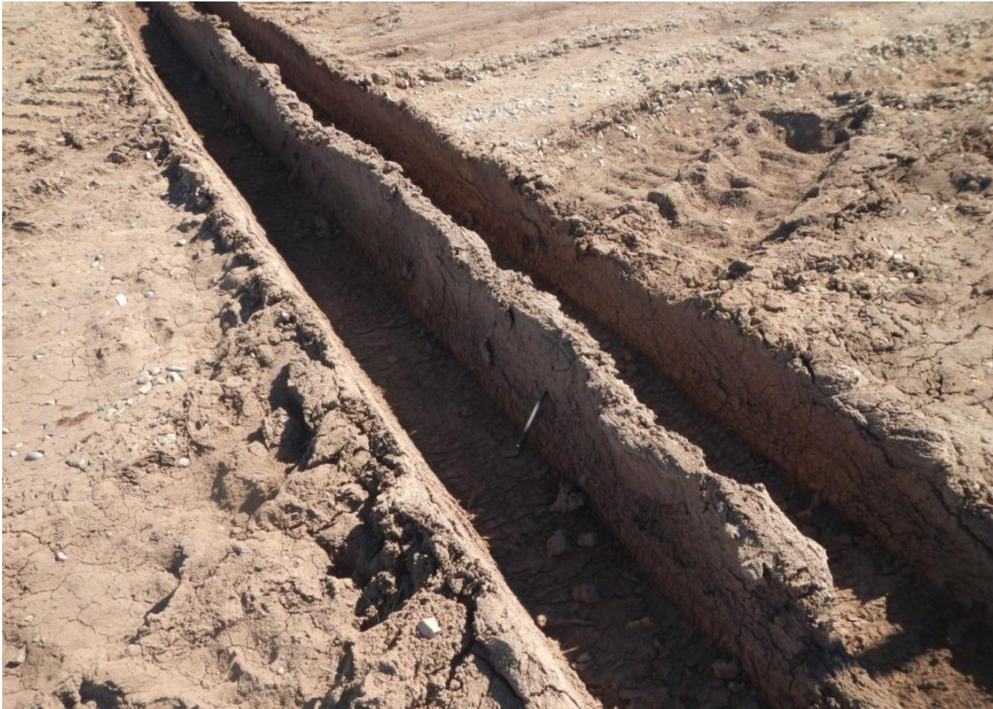
Photo 2. View of ruts in the well pad approximately 20 inches deep. The well pad surface needs better stabilization.
