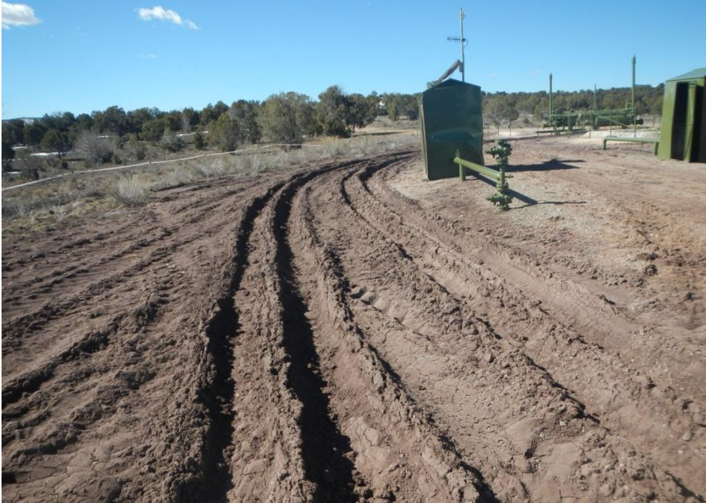
Photo 3. Another view of rutting within the project area. This needs to be stabilized.
