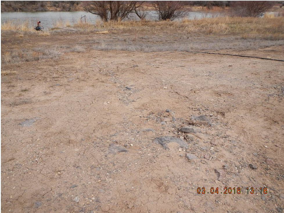
Second area of run-off and erosion 3/4/16
