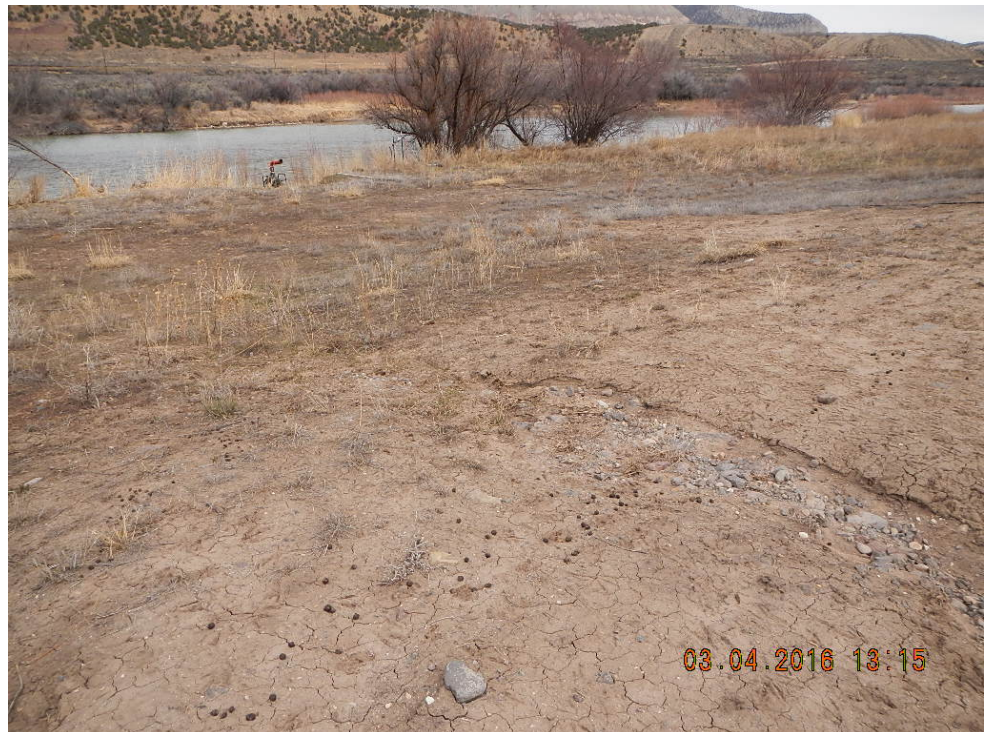
Same area with run-off and erosion 3/4/16
