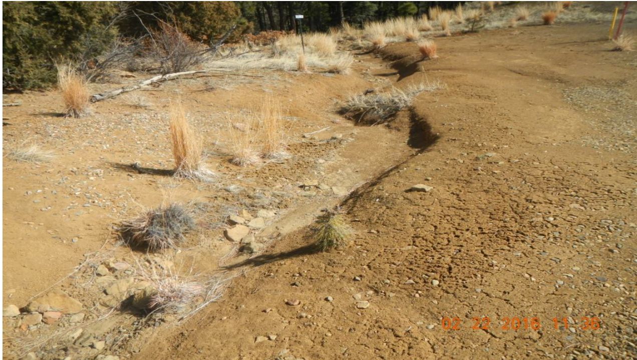
photo 3: Erosion channel transporting sediment off the northwest corner of the location.
