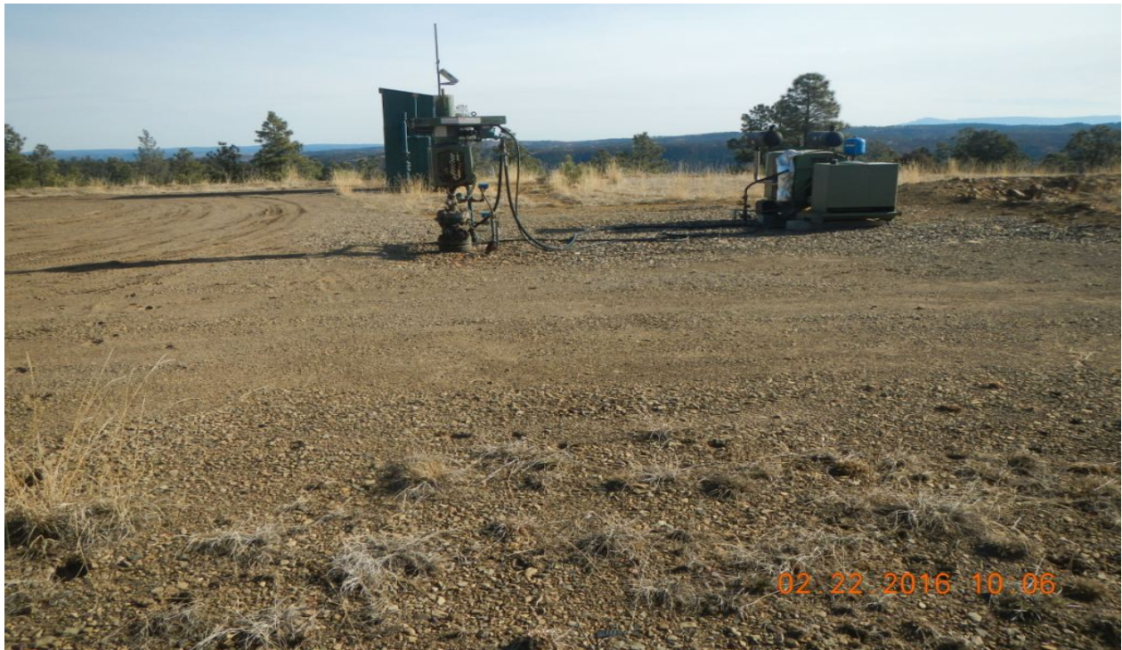
photo 3: Facing northeast toward the well head.
