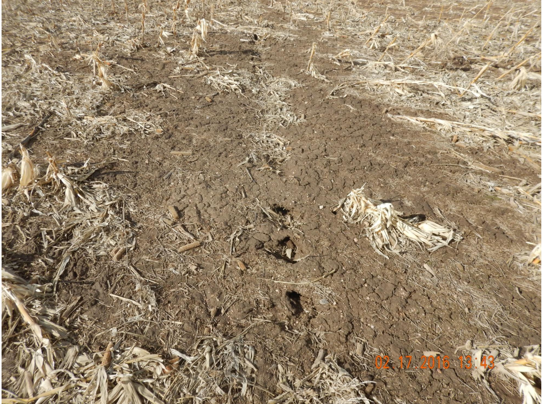
Figure 14: Photo taken northwest of project area, facing northwest. Photo shows subsidence occurring along pipeline.
