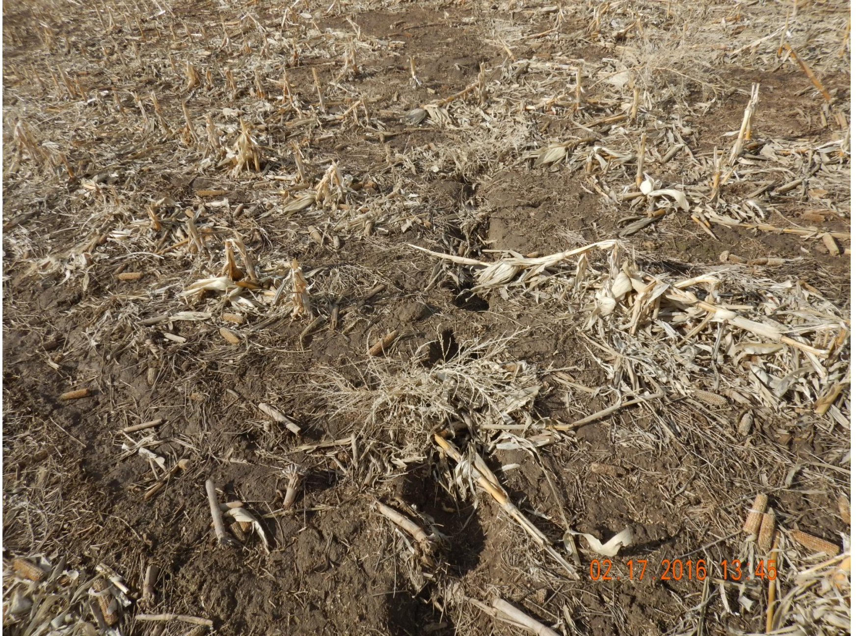
Figure 15: Photo taken northwest of project area, facing northwest. Photo shows subsidence occurring along pipeline.
