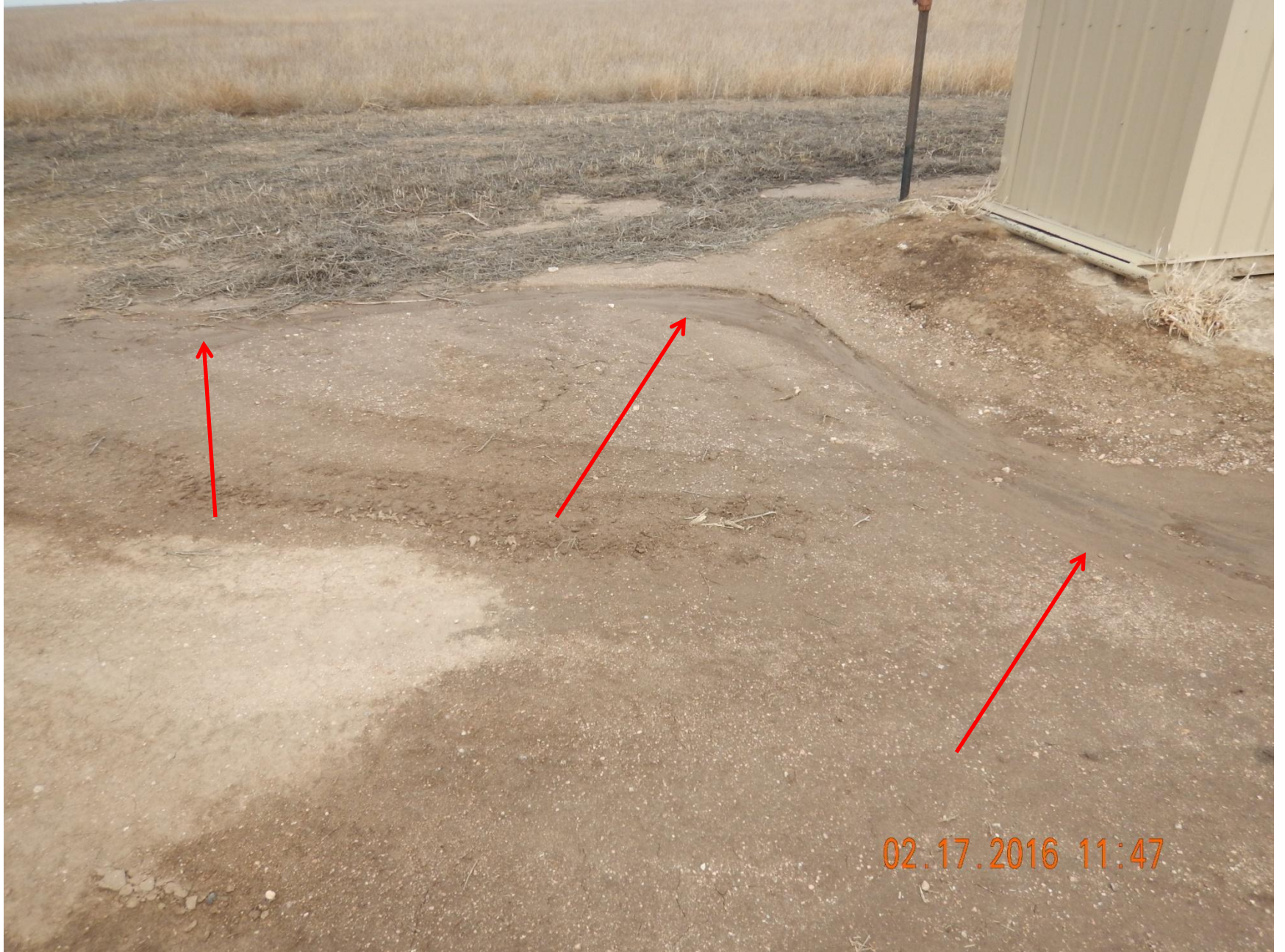
Figure 12: Photo taken from the southern end of location, facing north. Photo shows erosion patterns on project area.
