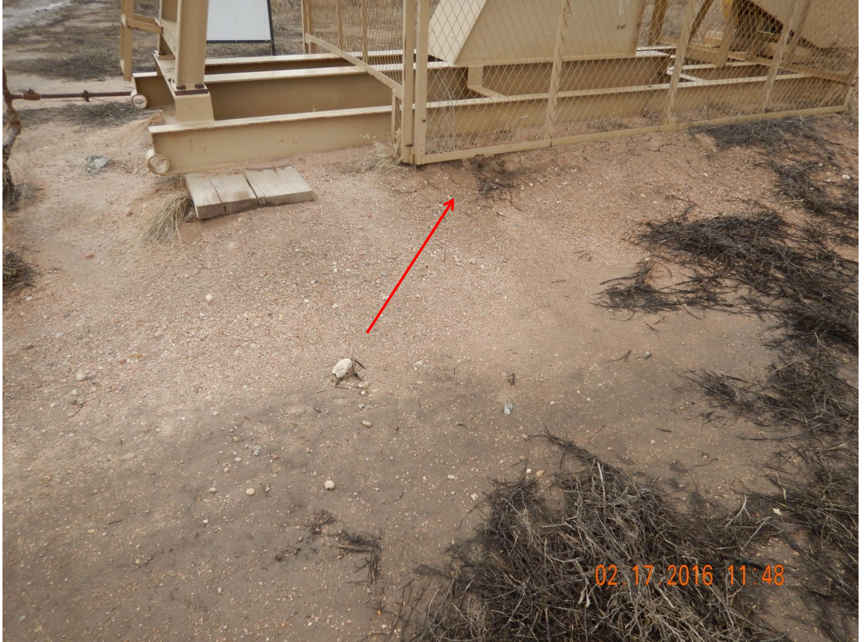
Figure 15: Photo taken from the northwest end of location, facing south. Photo shows erosion occurring at pump.
