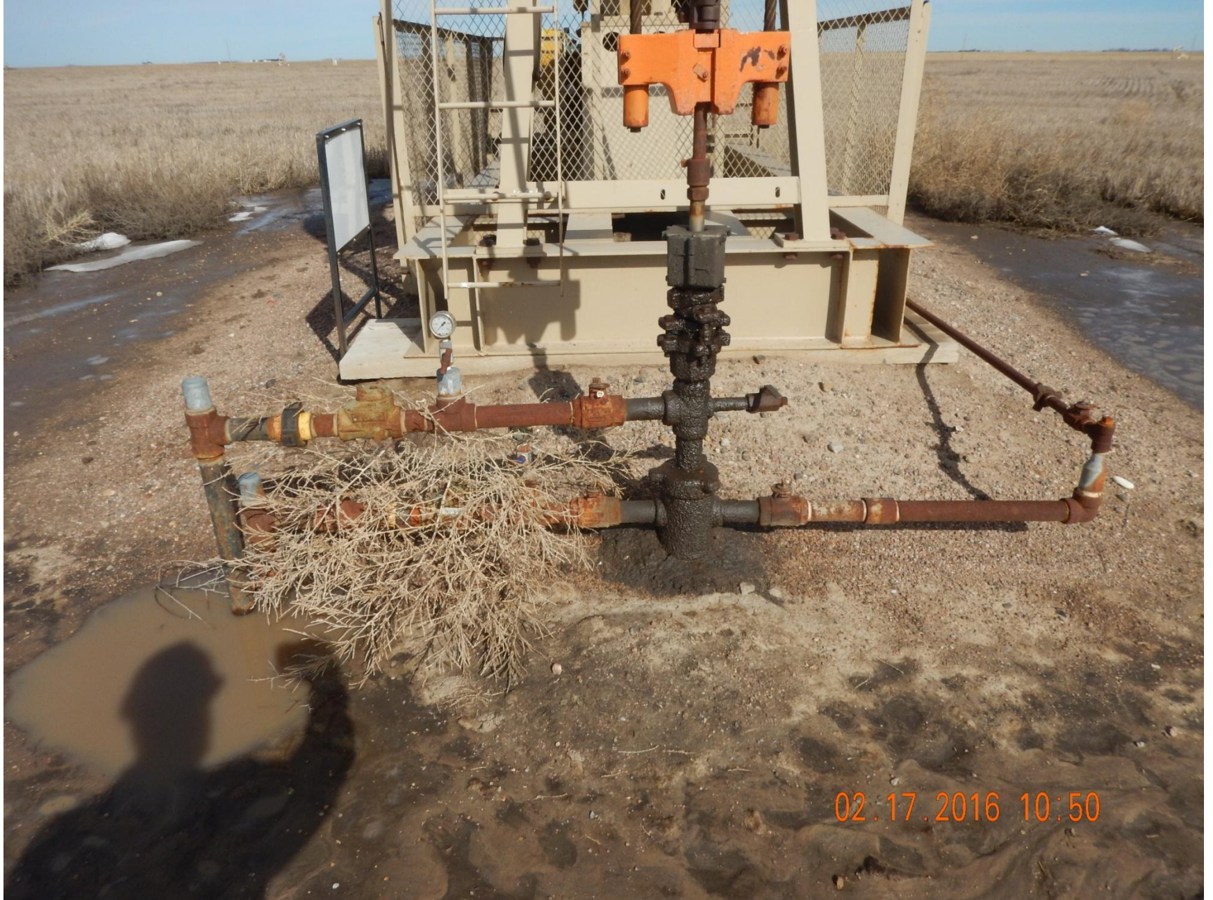
Figure 10: Photo taken at well head, facing north. Photo shows dark staining on soil at base of well on and equipment.
