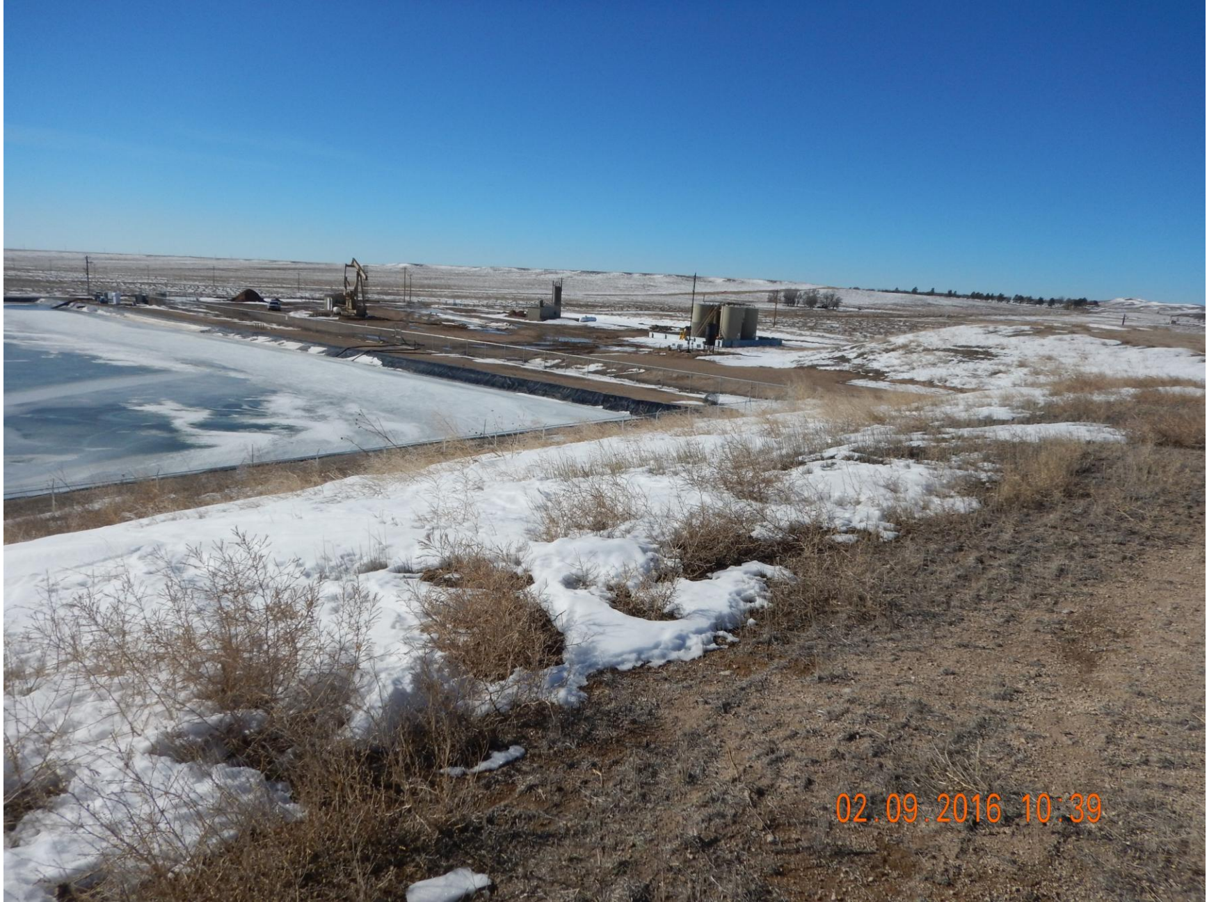
Figure 17: Photo taken from berm on the northeast end of interim area, facing southwest. Photo of erosion forming on berm.
