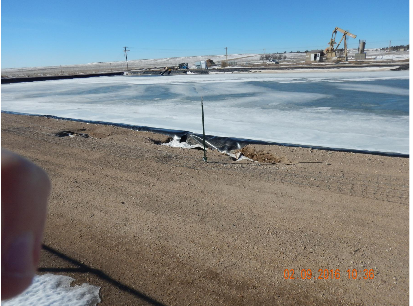
Figure 11: Photo taken from east end of pit location, facing west. Photo shows erosion occurring on pit containment berm.
