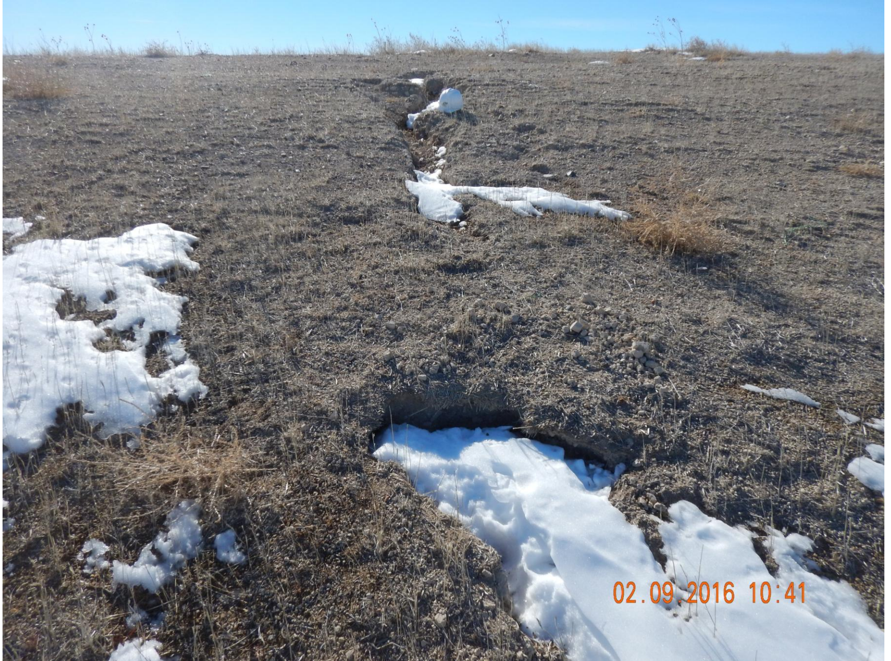
Figure 19: Photo taken from northern end berm on interim area, facing south. Photo shows rill erosion occurring on berm.
