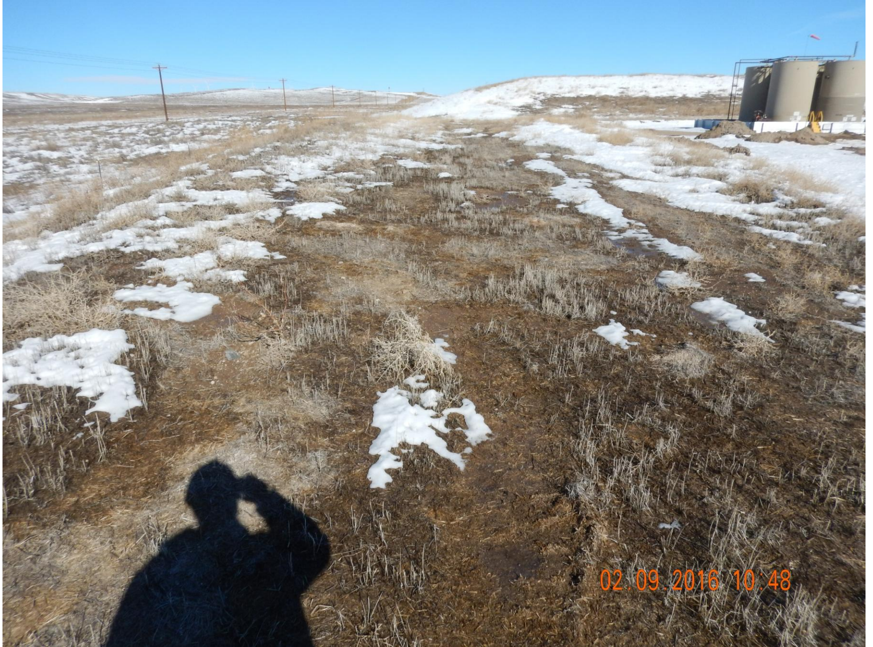
Figure 28: Photo taken from northwest end of project area. Photo of erosion forming on berm.
