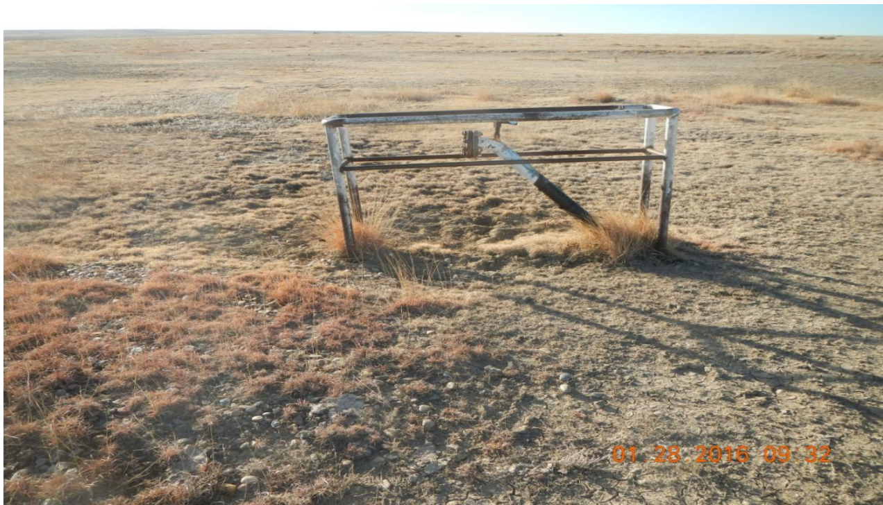
photo 4: One of two pipe risers that remain at the location. Lat/Long:37.09063,-102.48639.
