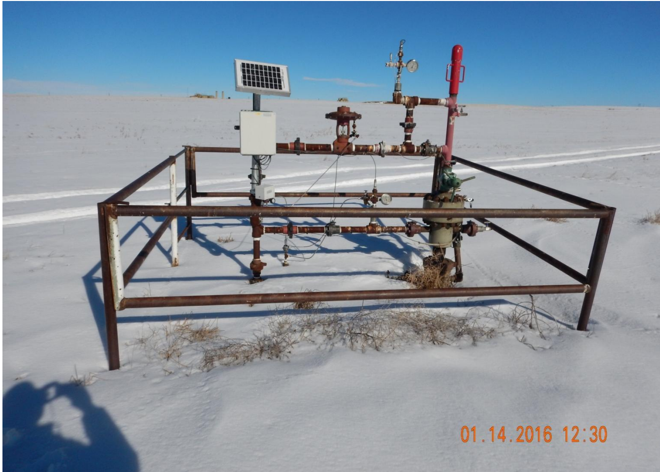
Photo 1. Photo taken of PR well API: 123-19596, facing North. Need to comply with Rule 210 and install sign at wellhead.
