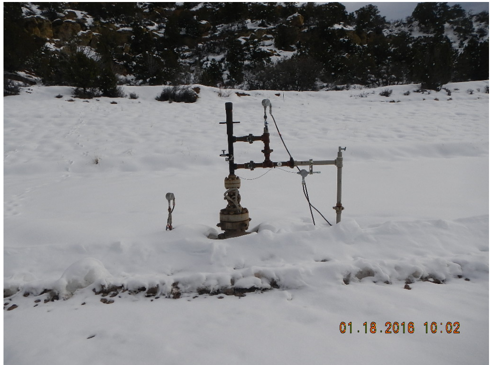
Wellhead with no sign
