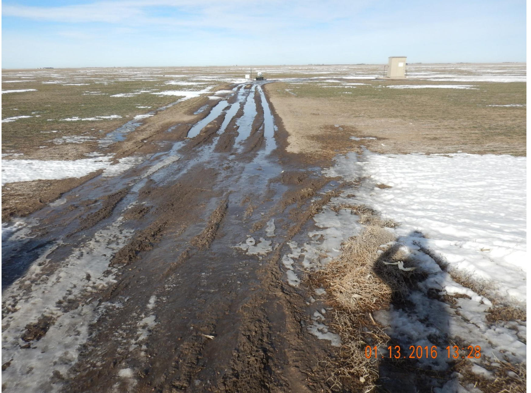
Figure 3: Photo taken from access road, south of location, facing north. Photo shows access road in disrepair.
