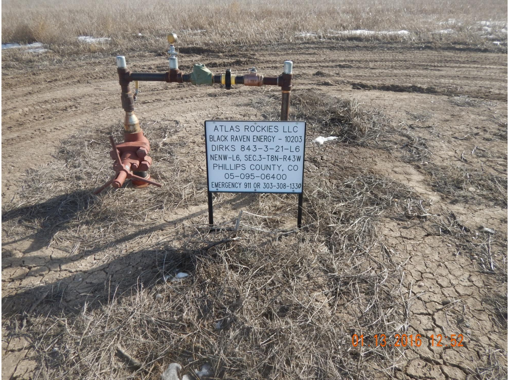
Figure 1: Photo of sign at wellhead.
