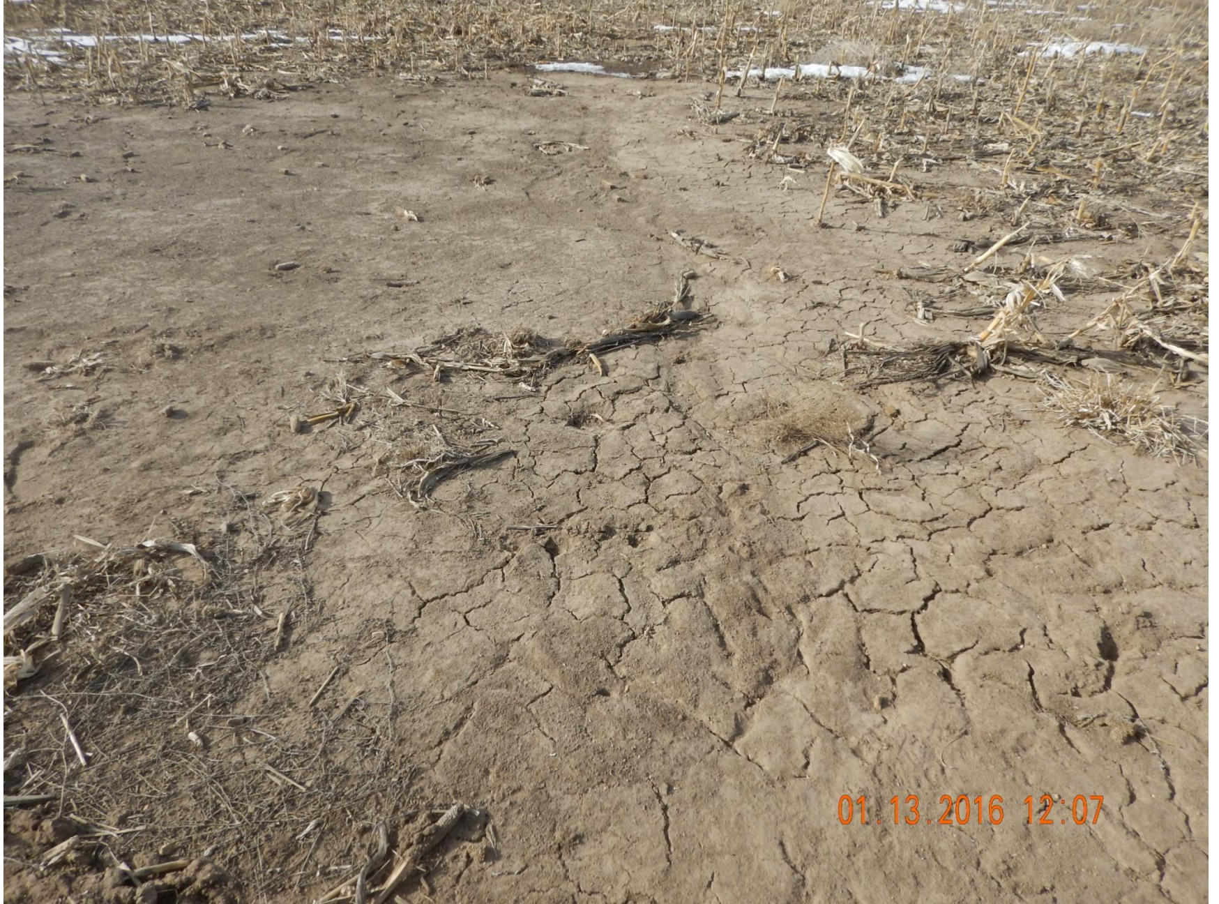
Figure 6: Photo taken north end of location, facing west. Photo shows erosion starting to occur from the project area leaving location.
