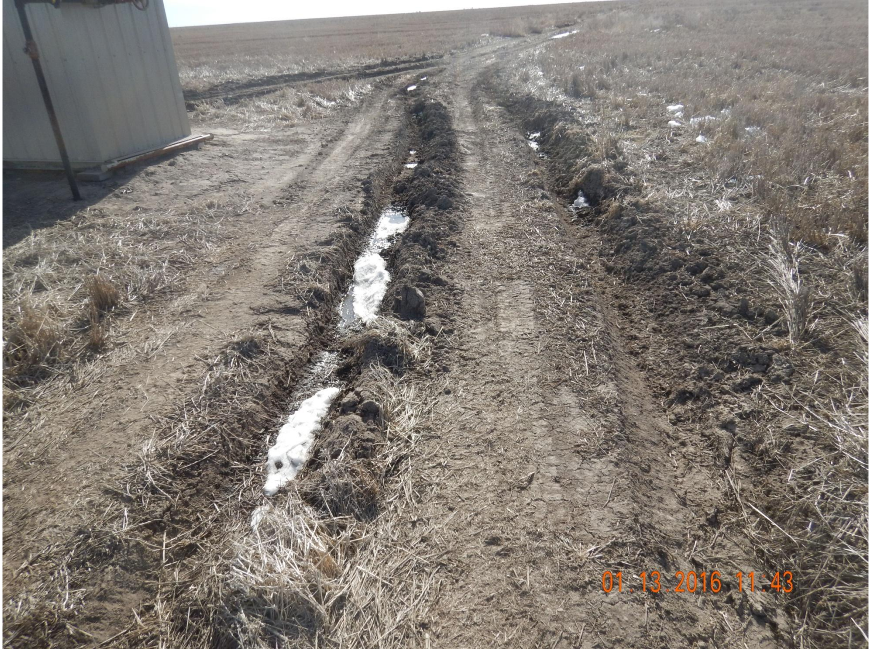
Figure 6: Photo taken from the west end of location, facing south. Photo shows access road in disrepair.
