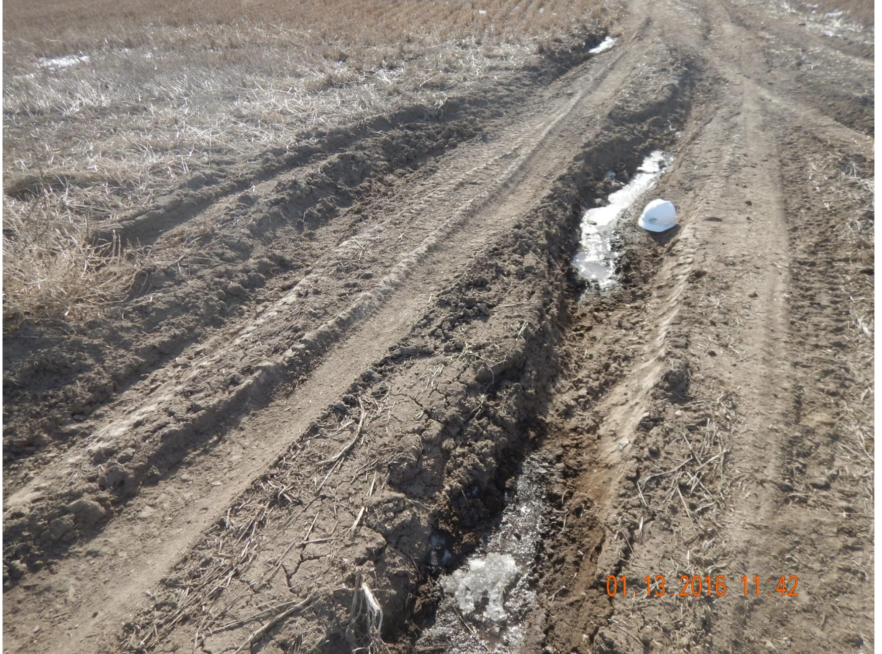
Figure 4: Photo taken from the south end of location, facing south. Photo shows access road in disrepair.
