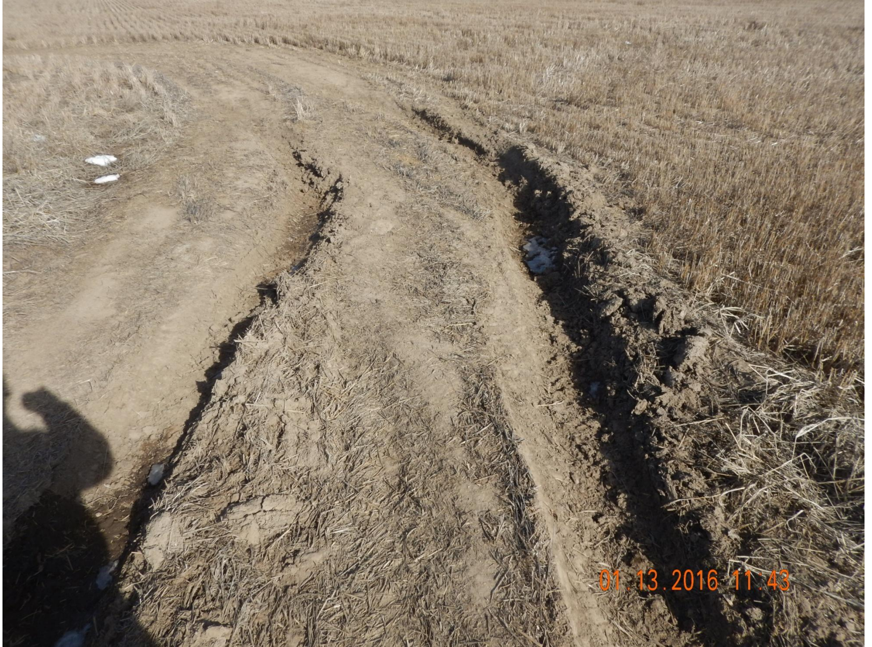
Figure 5: Photo taken from the east end of location, facing north. Photo shows access road in disrepair.
