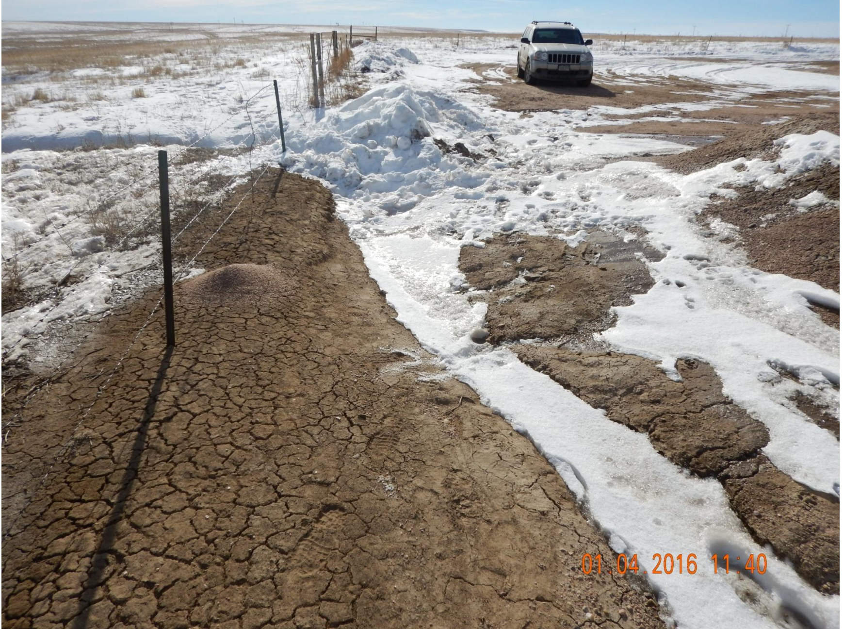
Figure 4: Photo taken from east end of location, facing south. Photo shows stormwater and sediment control BMPs have not been installed.
