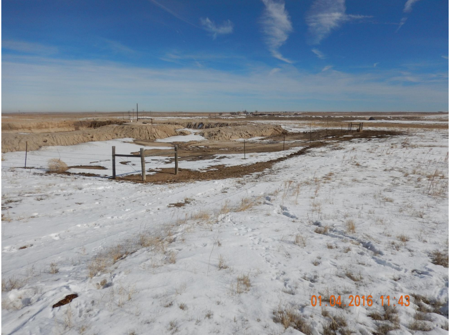
Figure 9: Photo taken from southwest end of pit location, facing northeast. Photo shows stormwater and sediment control BMPs have not been installed.
