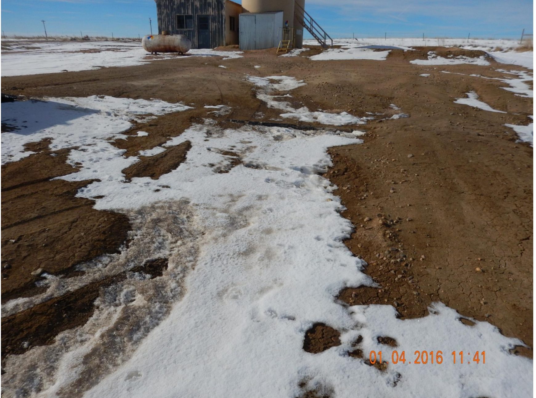
Figure 5: Photo taken from north end of location, facing west. Photo of erosion and exposed pipe.
