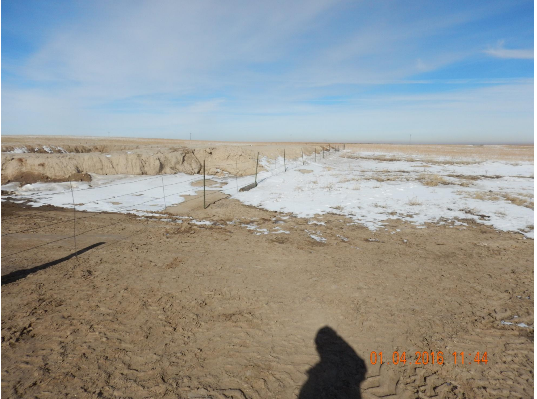
Figure 11: Photo taken southeast end of pit location, facing north. Photo shows stormwater and sediment control BMPs have not been installed.
