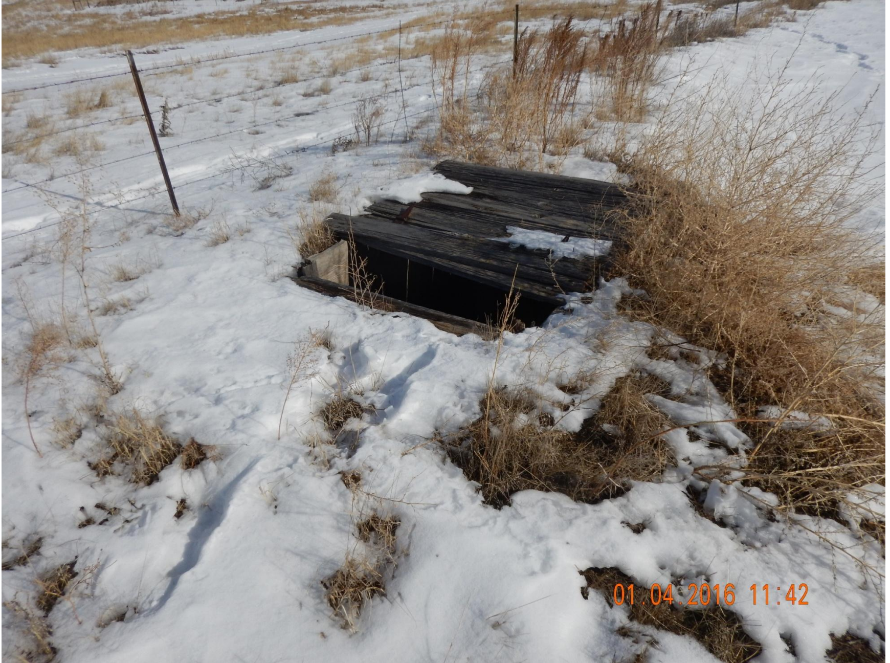
Figure 7: Photo taken from northwest portion of location, facing south. Photo shows door to box-framed subsurface structure remains in disrepair.
