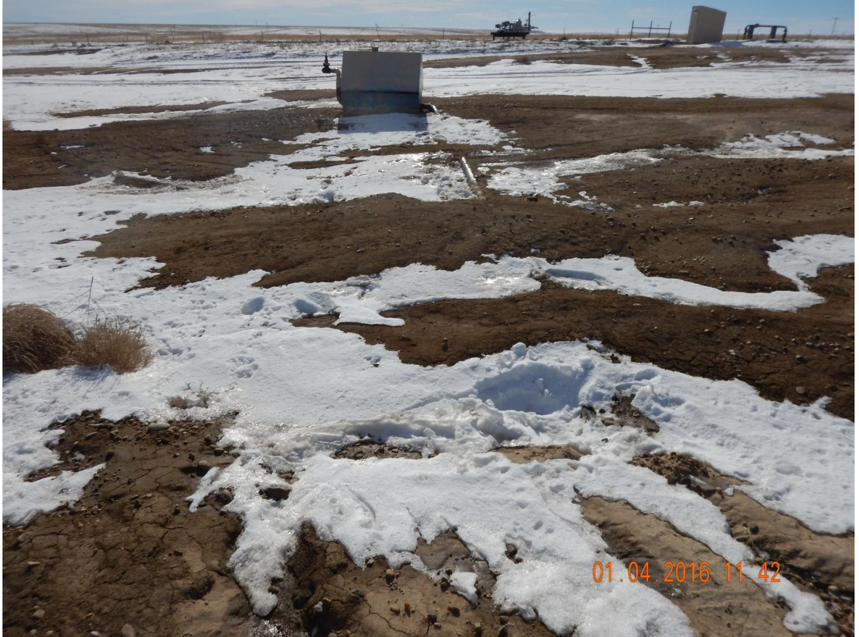
Figure 6: Photo taken from north end of location, facing south. Photo of erosion and exposed pipe.
