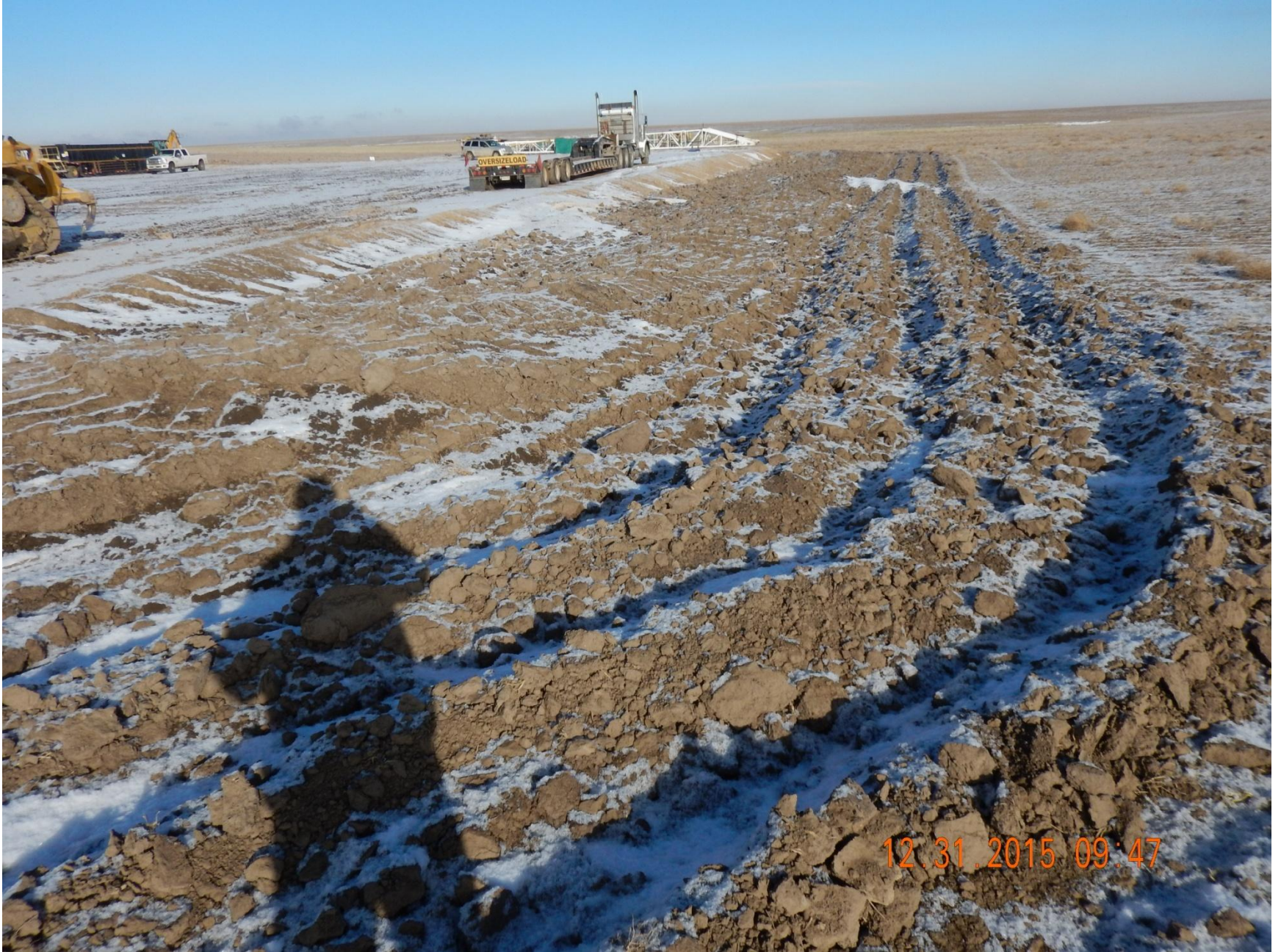
Figure 5: Photo taken from southeast end of location, facing north. Photo of stormwater BMPs
