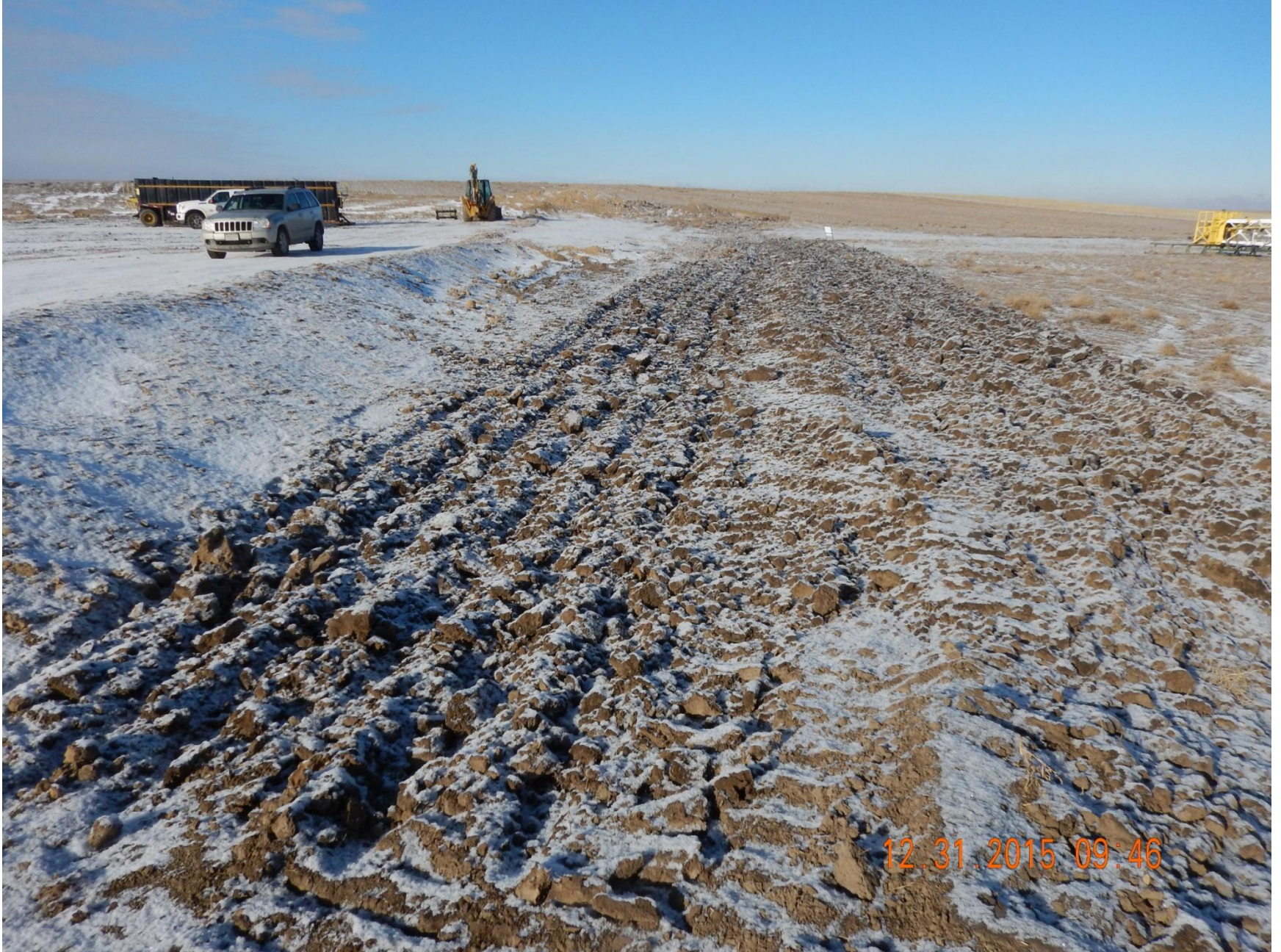
Figure 4: Photo taken from northeast end of location, facing west. Photo of stormwater BMPs
