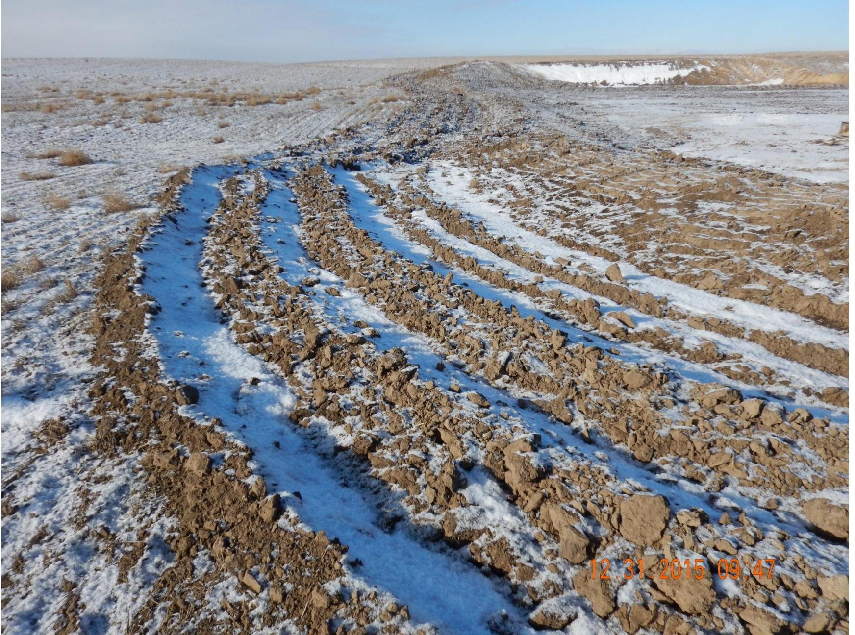
Figure 6: Photo taken from southeast end of location, facing west. Photo of stormwater BMPs
