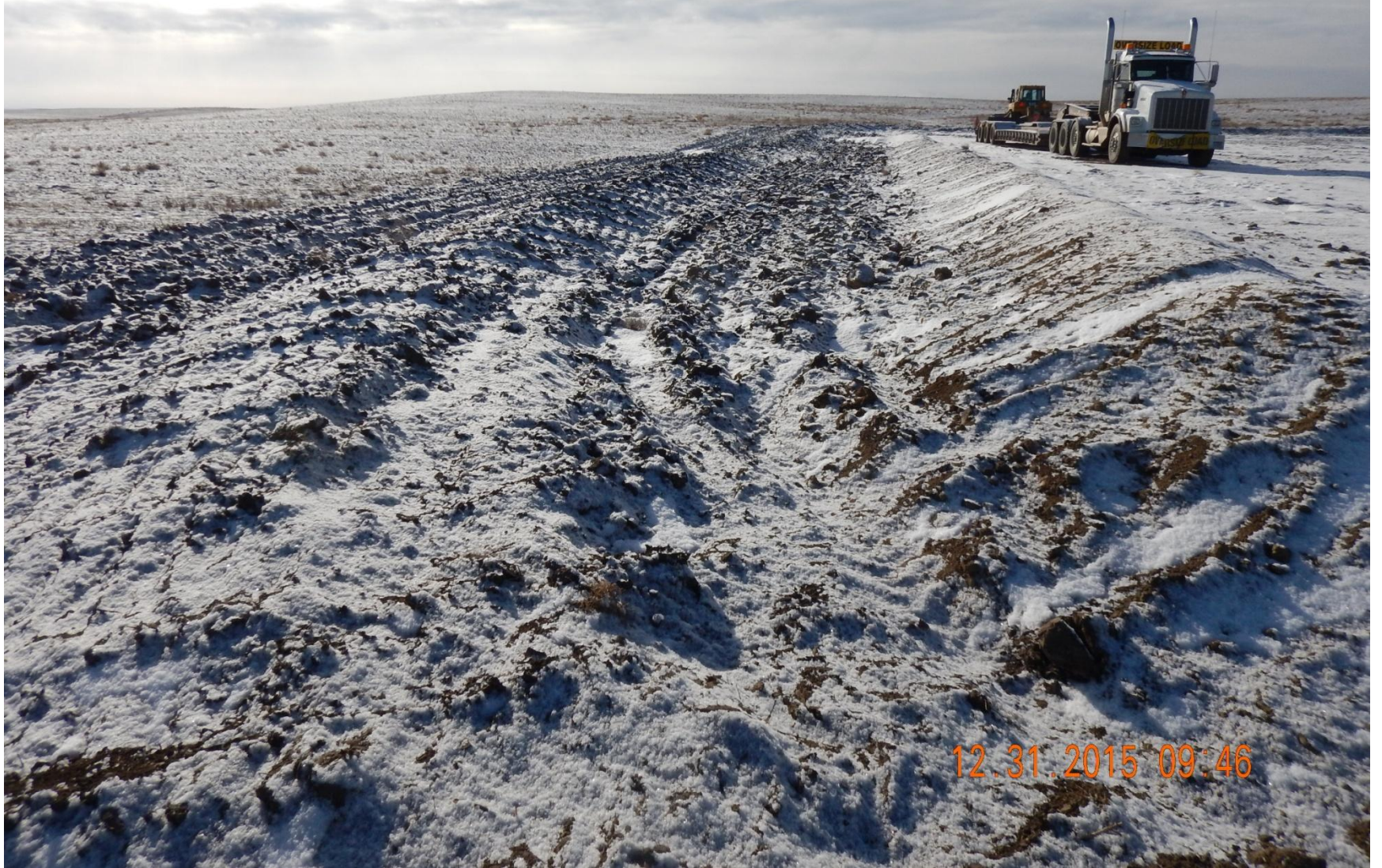
Figure 3: Photo taken from northeast end of location, facing south. Photo shows stormwater BMPs
