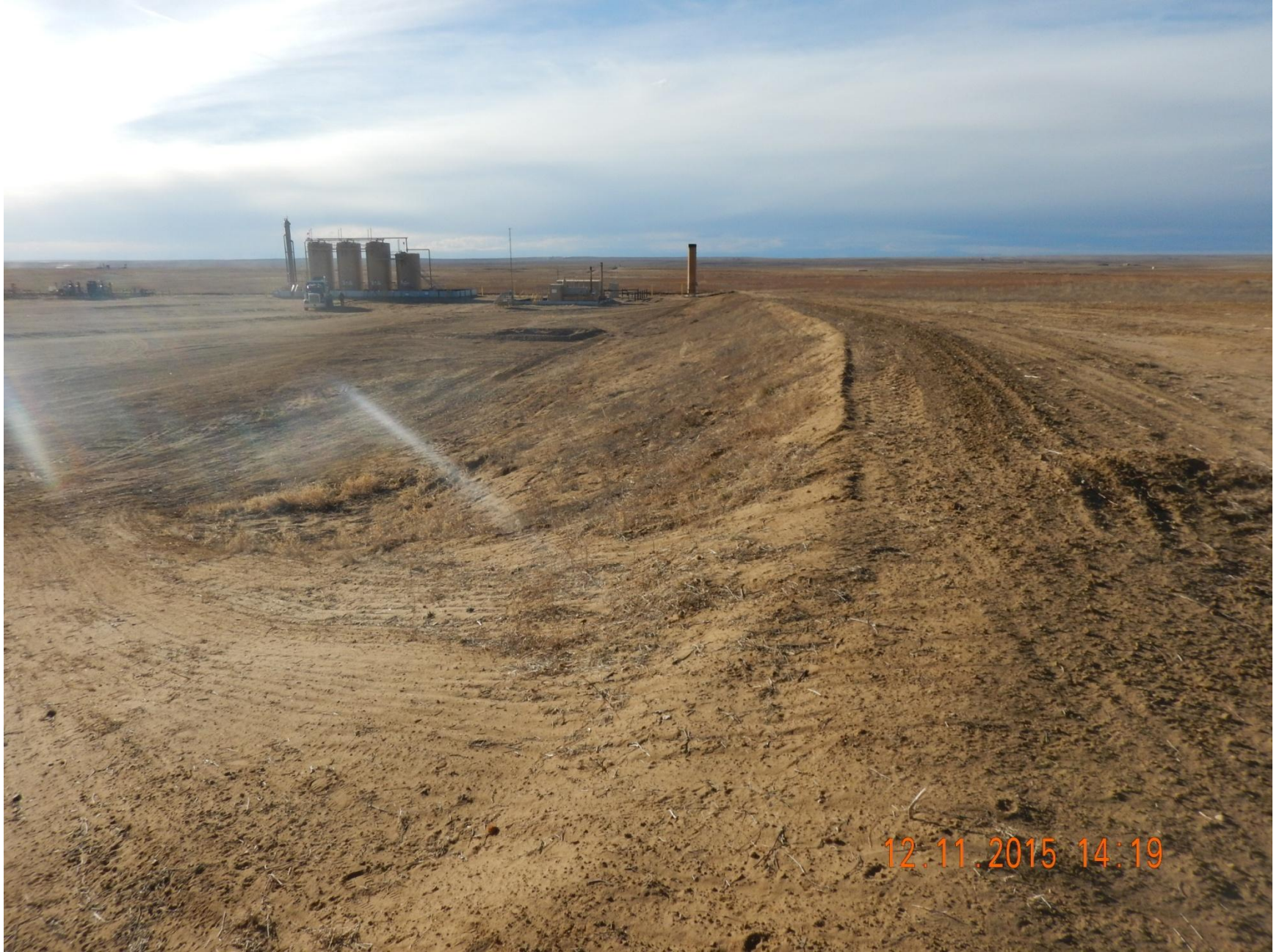
Figure 2: Photo taken from the northeast end of location, facing west. Photo shows weed debris has been removed.
