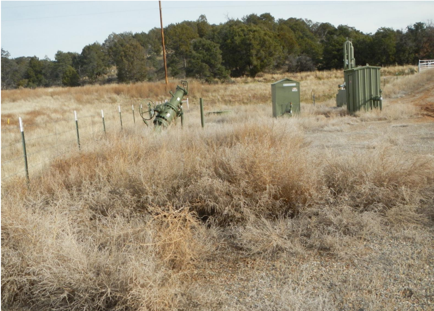
Photo 3. View of the northern portion of the project area from the northwestern corner facing eastward. The majority of the well pad surface is infested with kochia debris that needs removal.
