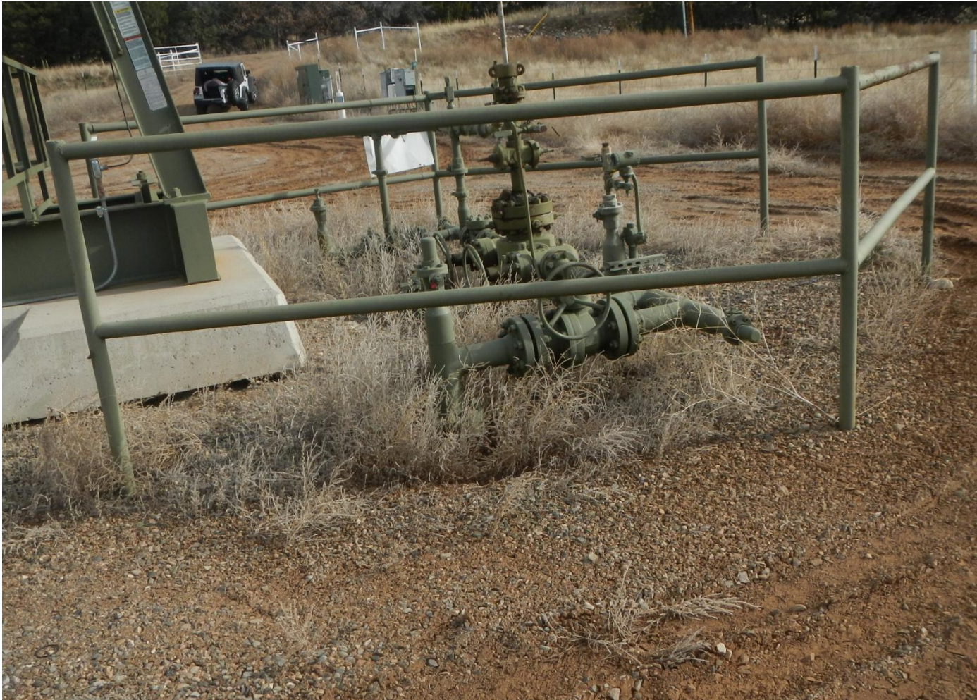
Photo 5. View of weeds around facilities that needs to be removed.
