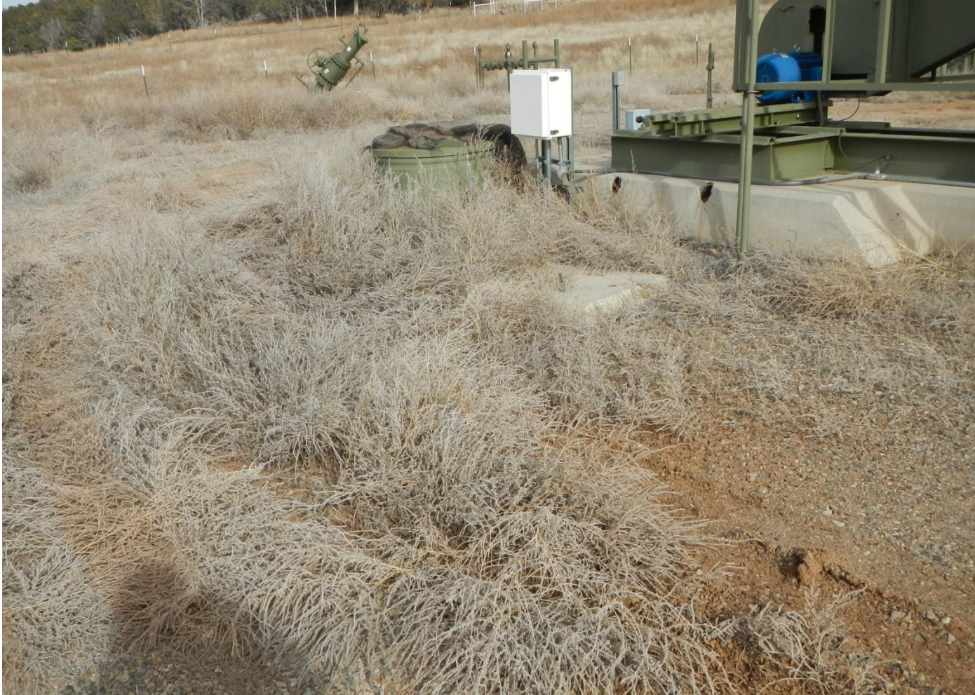
Photo 6. Another view of weeds around facilities that needs to be removed.
