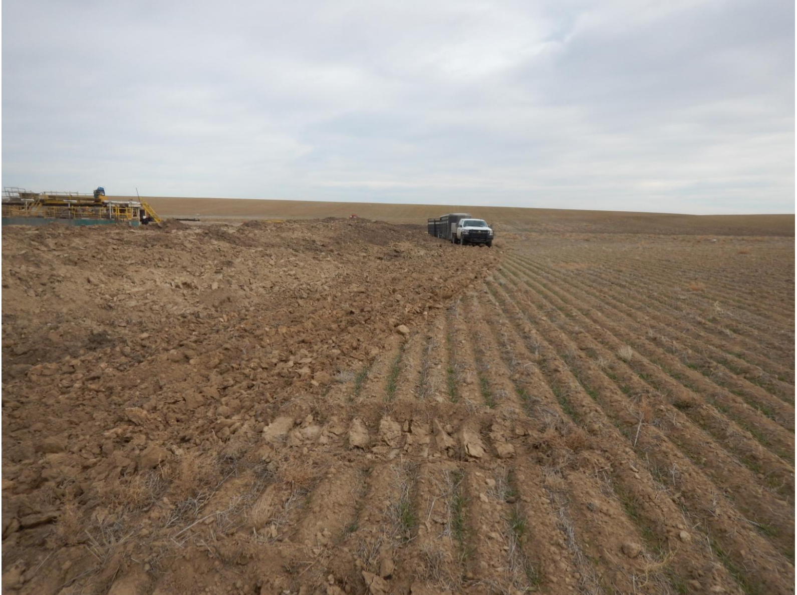
Figure 6: Photo taken from Southwest portion of location, facing east. Photo shows surface roughening (sediment control BMP), and vehicle park on said sediment control BMP.
