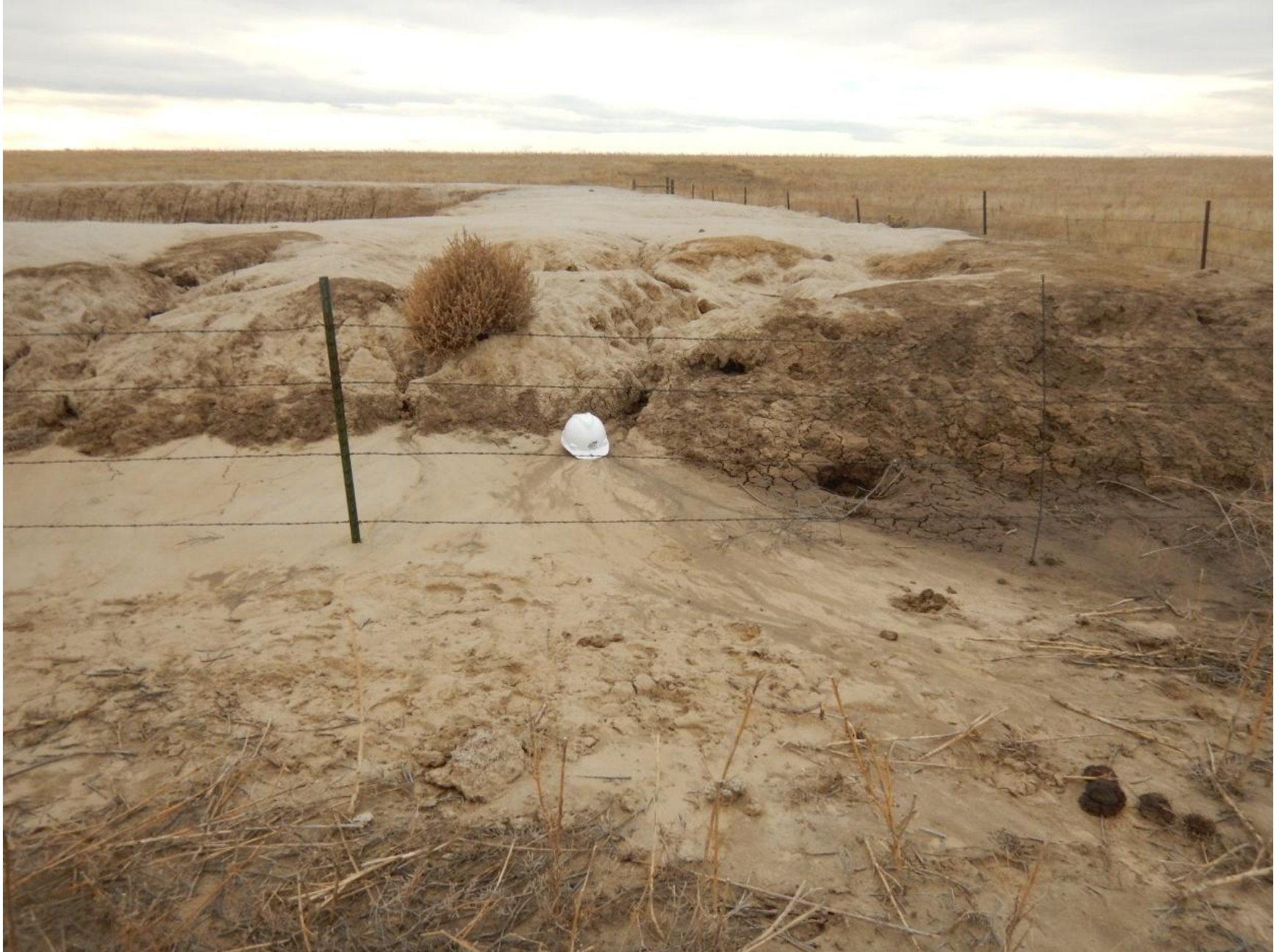
Figure 20: Photo taken from northeast end of pit location. Photo shows stormwater erosion on pit's containment berm, sediment deposition off of location, and insufficient stormwater BMPs.
