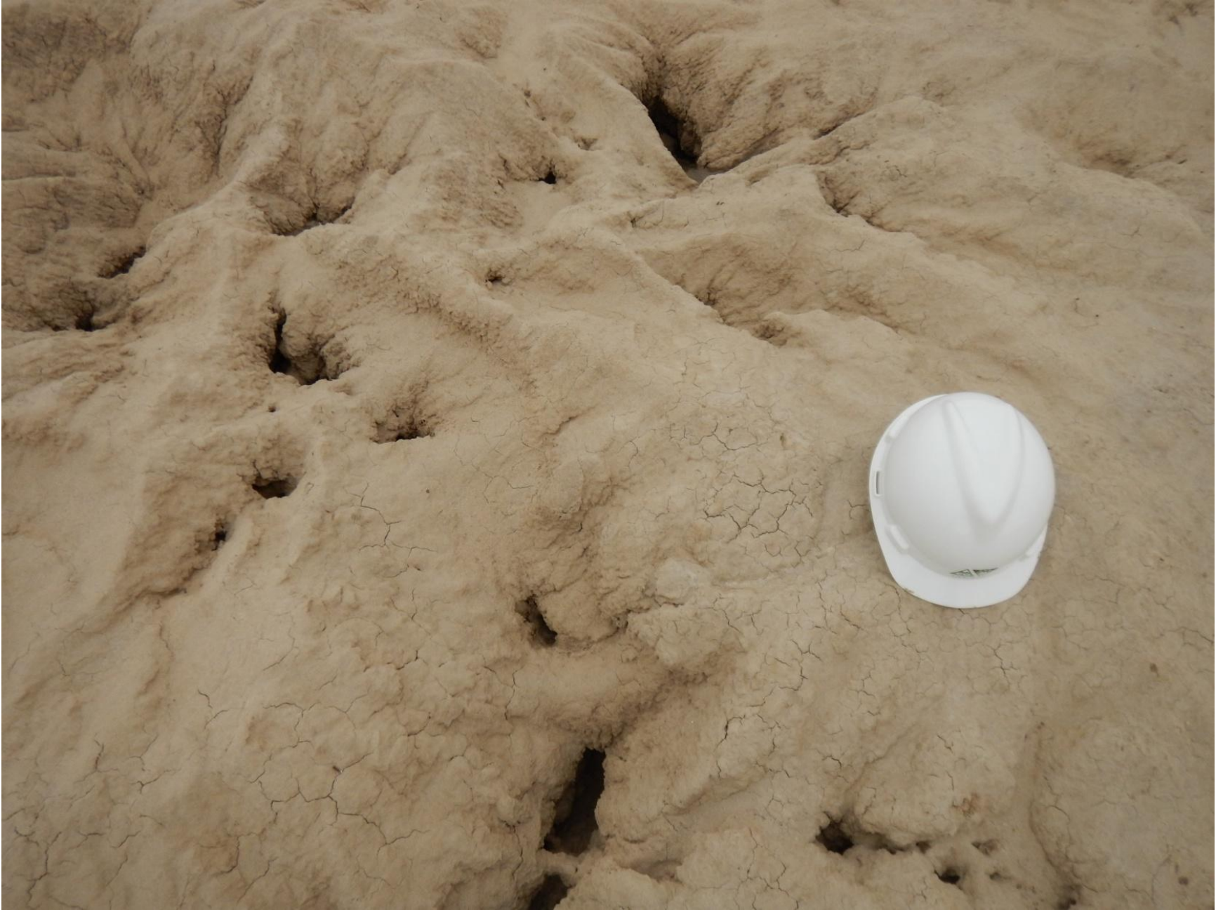
Figure 24: Photo taken from east end of pit location . Photo shows stormwater erosion on pit's containment berm. Stormwater flow occurring on surface, as well as the subsurface of the berm
