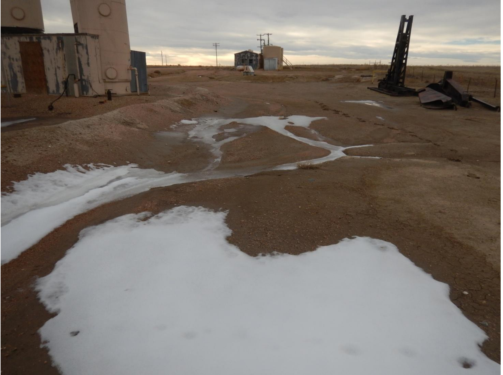
Figure 12: Photo taken from northeast end of location. Photo shows surface erosion on location and insufficient stormwater BMPs.
