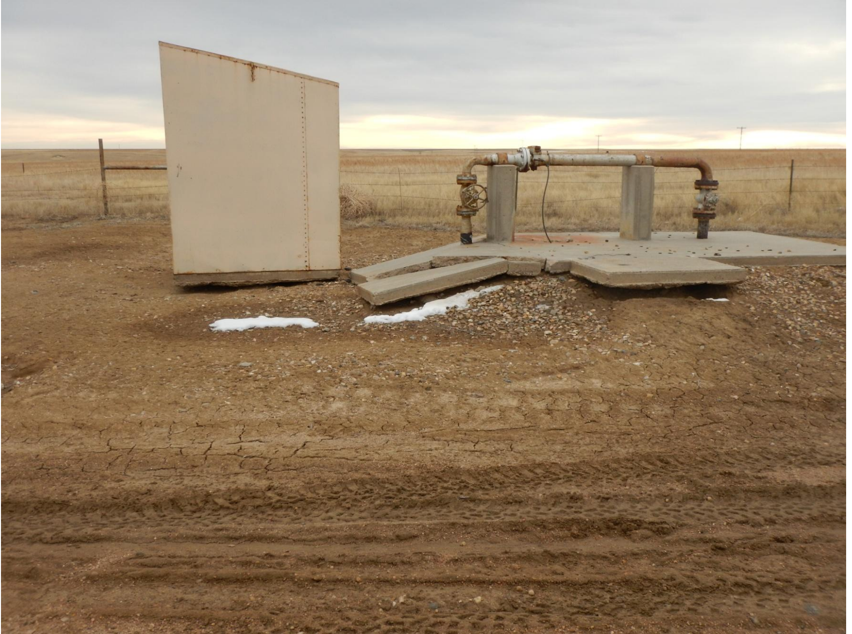
Figure 16: Photo taken from south end of location. Photo of sediment erosion occurring under concrete structure.
