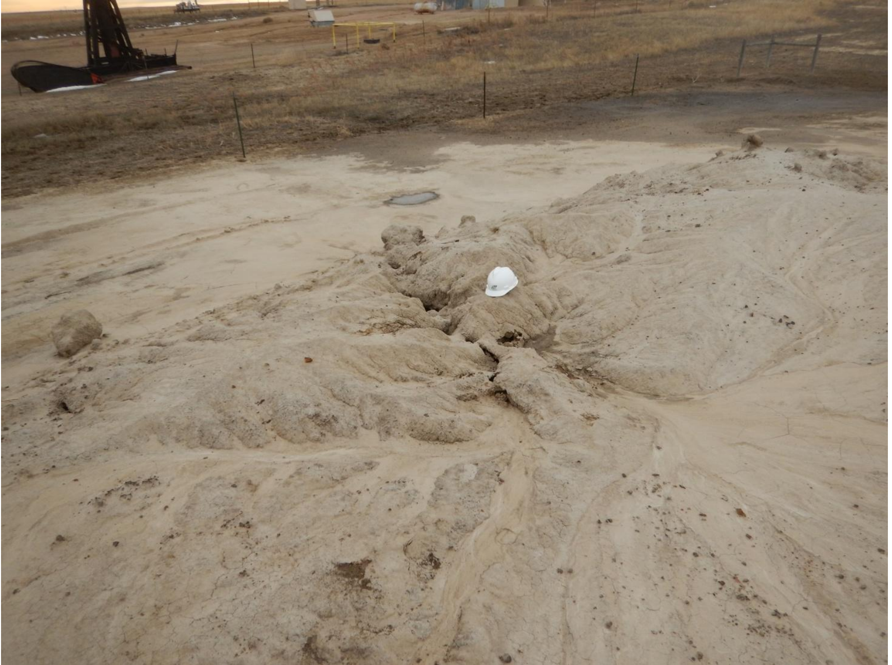
Figure 25: Photo taken from southwest end of pit location. Photo shows stormwater erosion on pit's containment berm, sediment deposition off of location, and insufficient stormwater BMPs.
