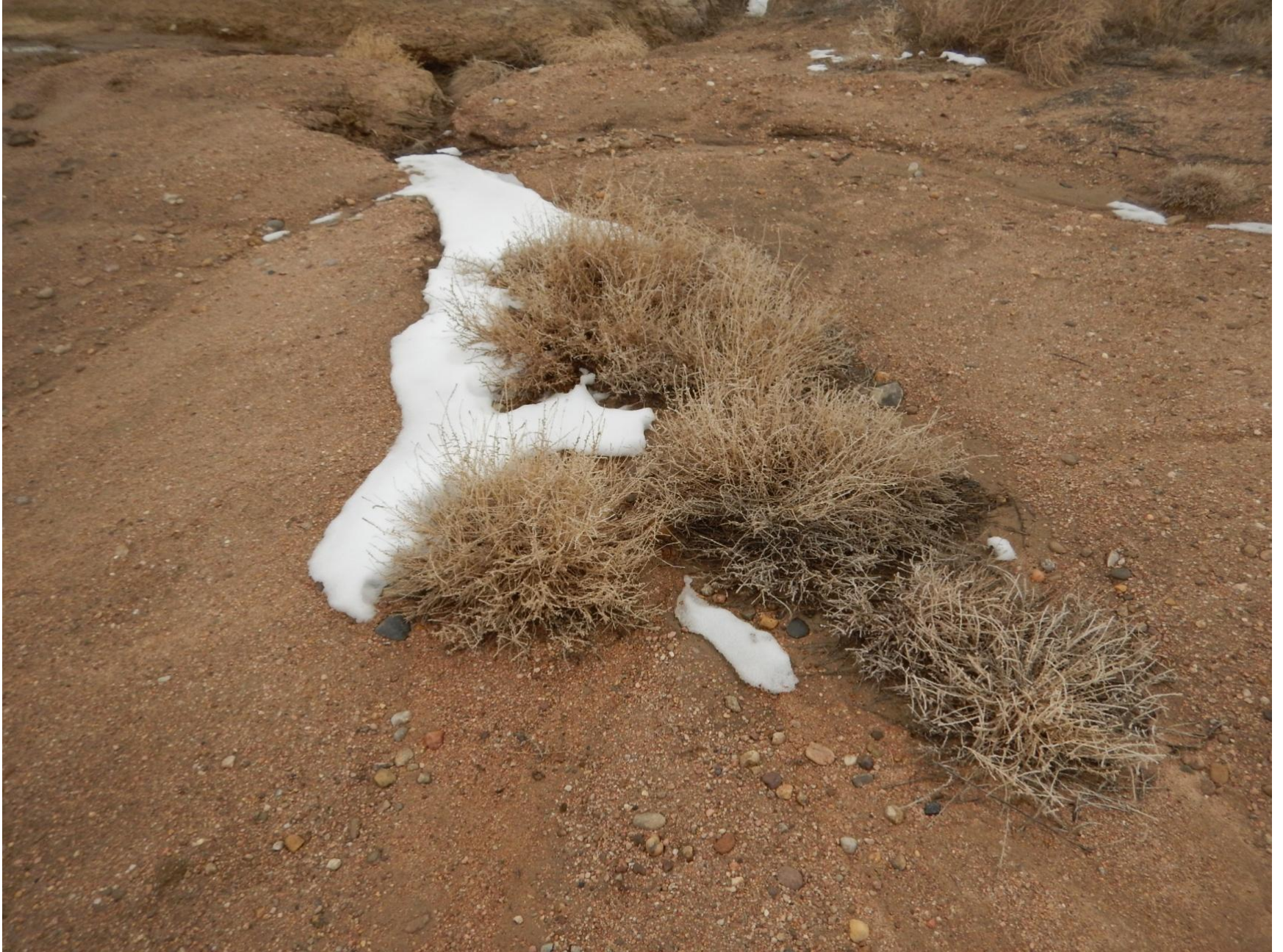
Figure 2: Photo taken from east end of location. Photo of gully formation, Russian thistle weed debris and insufficient stormwater BMPs.
