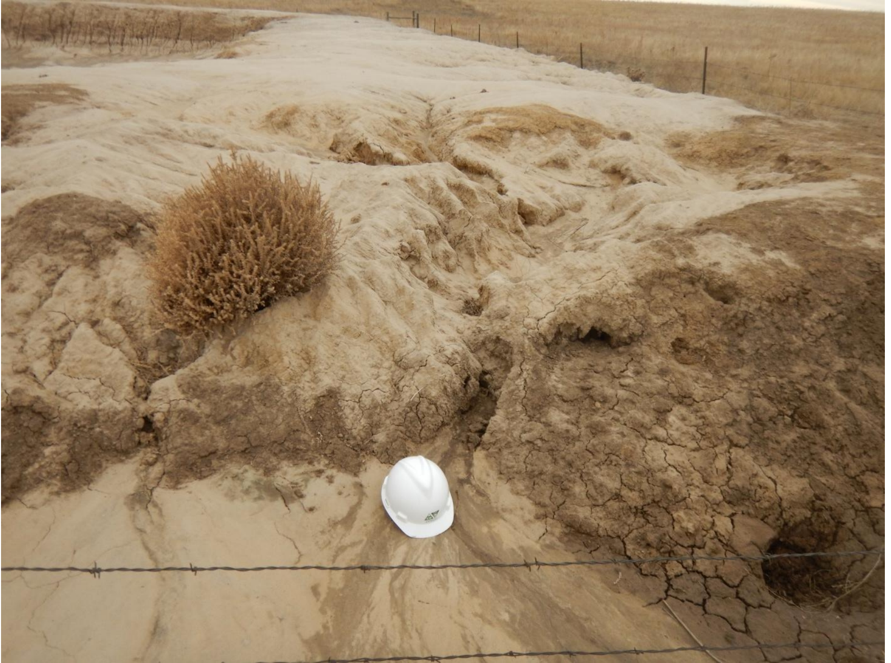
Figure 19: Photo taken from northeast end of pit location. Photo shows stormwater erosion on pit's containment berm and insufficient stormwater BMPs.
