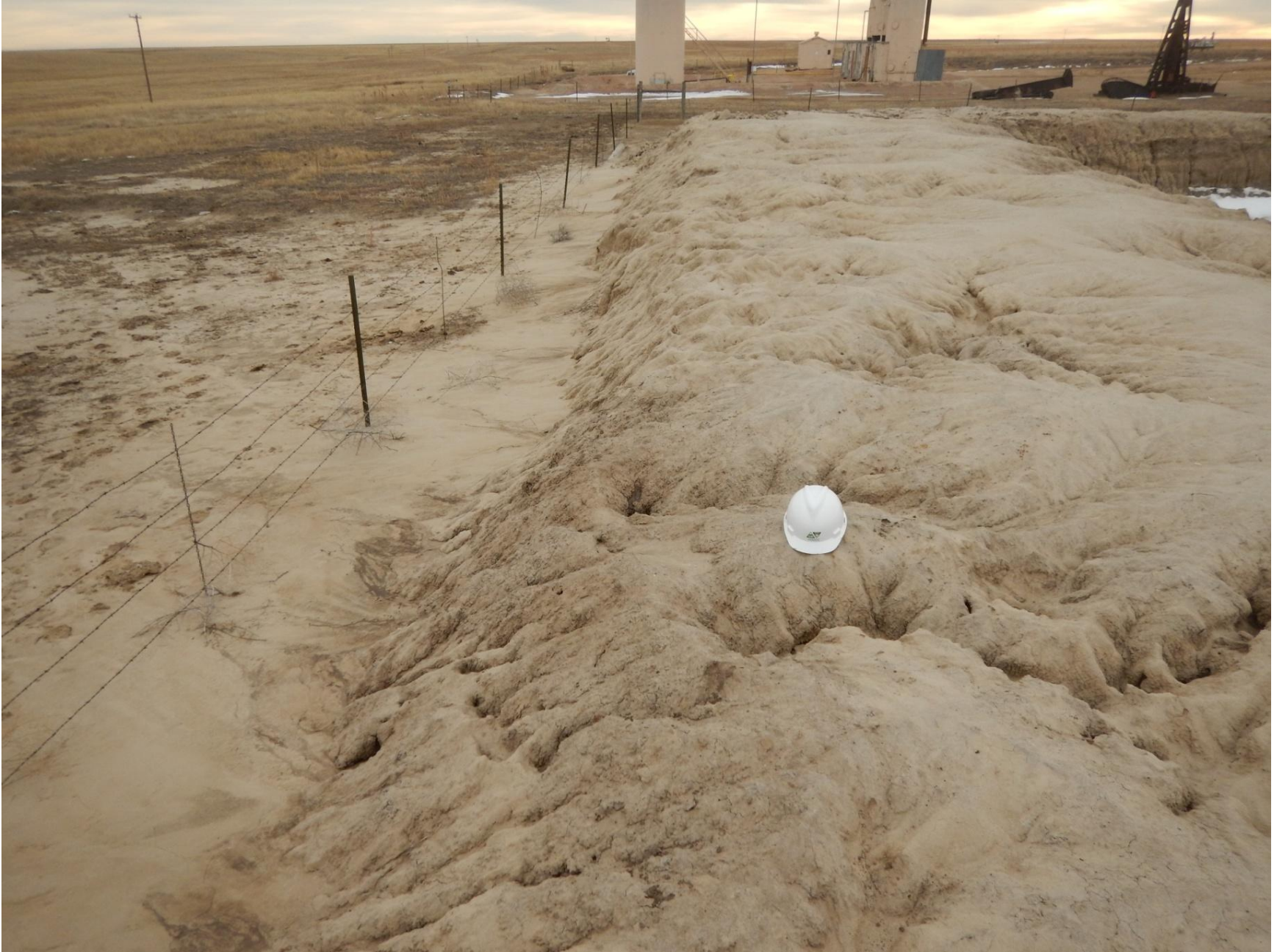
Figure 22: Photo taken from east end of pit location. Photo shows stormwater erosion on pit's containment berm. Stormwater flow occurring on surface, as well as the subsurface of the berm.
