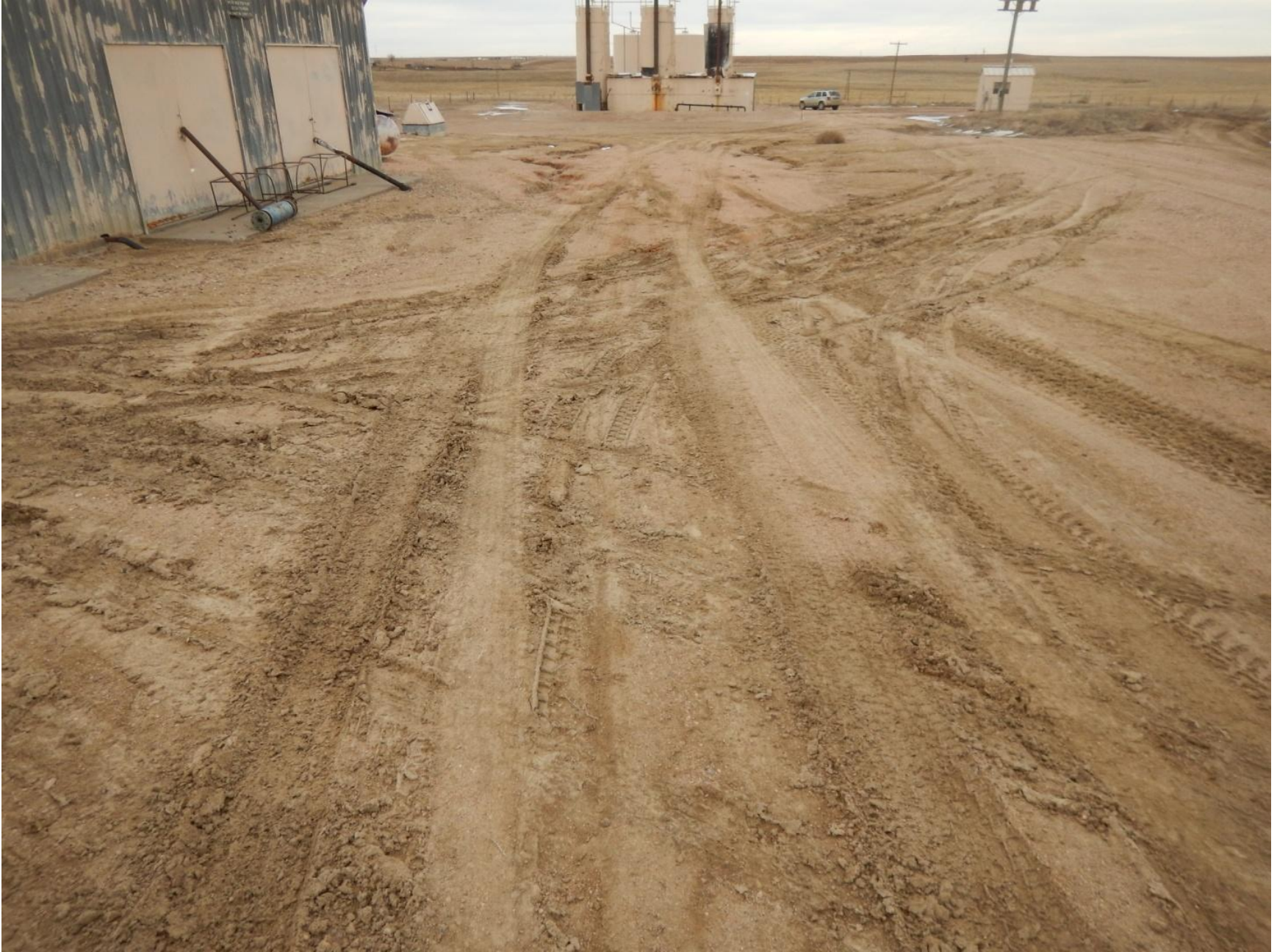
Figure 11: Photo taken from west end of location. Photo shows surface erosion on location and insufficient stormwater BMPs.
