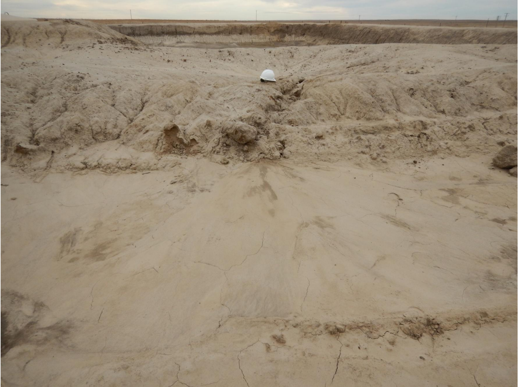
Figure 26: Photo taken from southwest end of pit location facing north. Photo shows stormwater erosion on pit's containment berm, sediment deposition, and insufficient stormwater BMPs.
