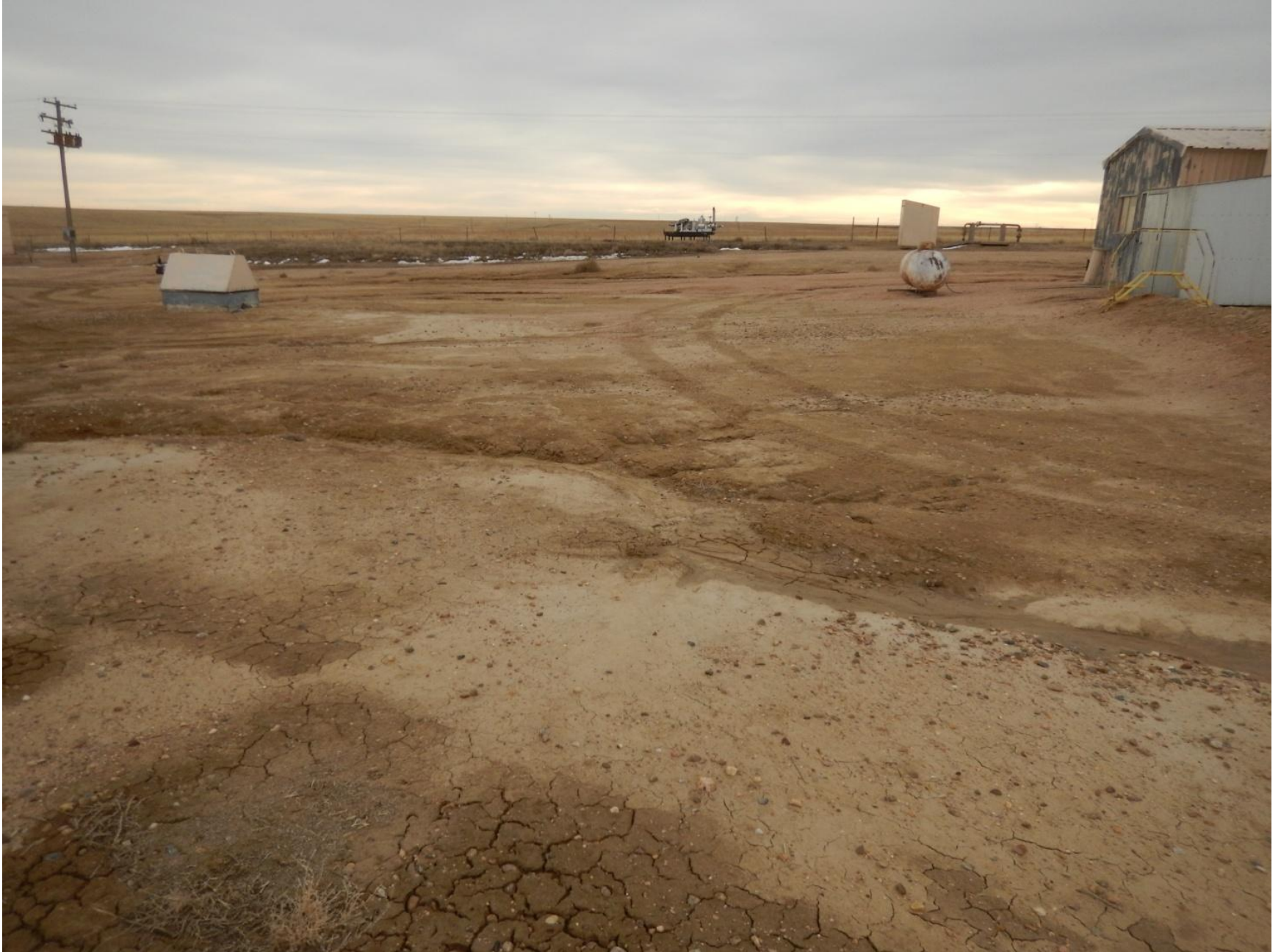
Figure 7: Photo taken from north end of location facing south. Photo shows surface erosion on location and insufficient stormwater BMPs.
