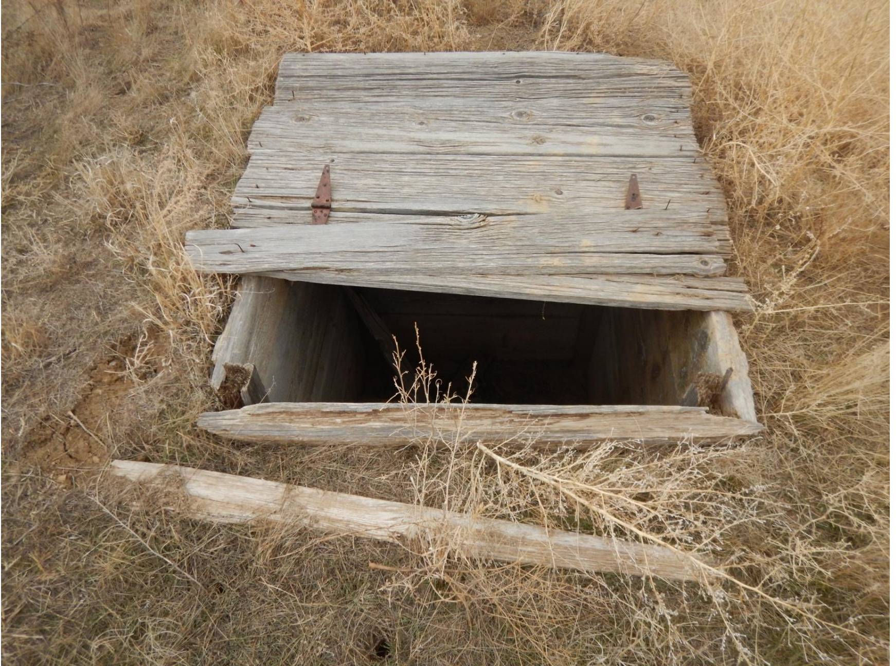
Figure 9: Photo taken from northwest end of location. Photo shows broken door of wooden sub-surface structure. This poses a hazard to wildlife and human safety.
