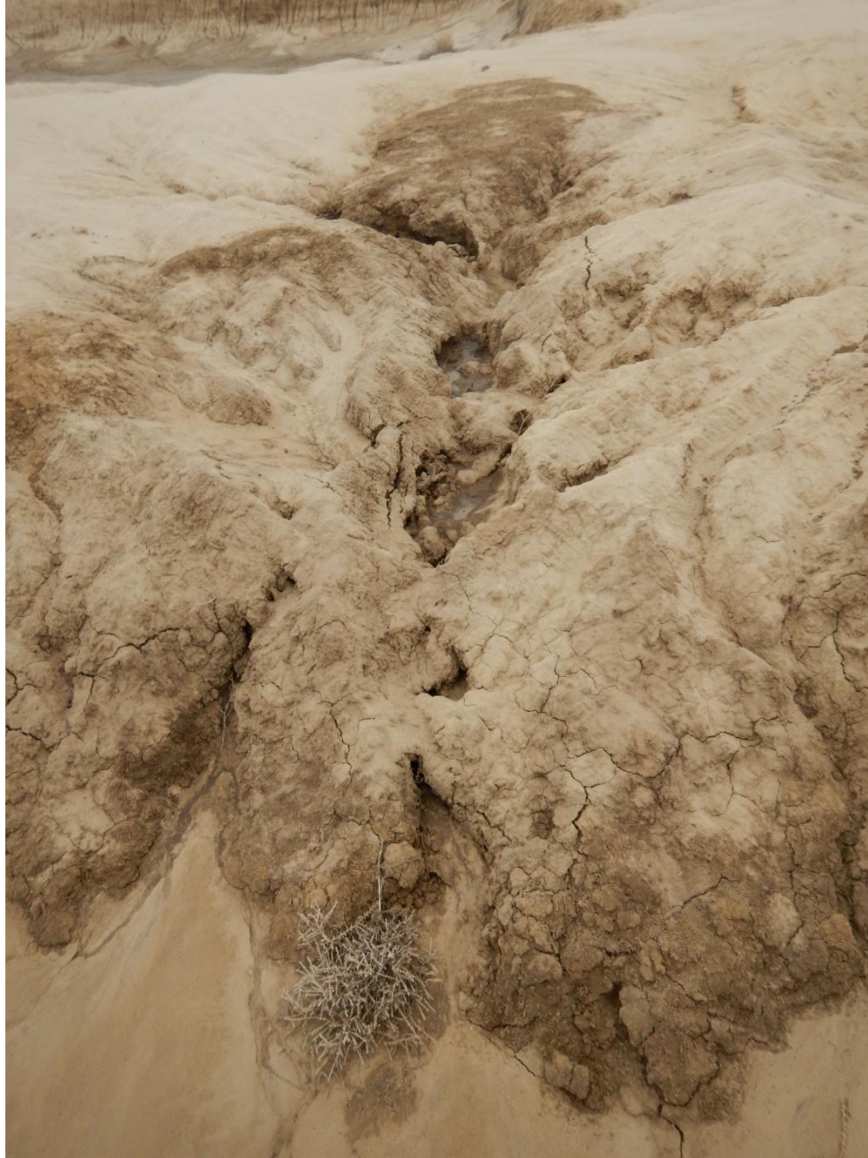
Figure 21: Photo taken from east end of pit location. Photo shows stormwater erosion on pit's containment berm. Stormwater flow occurring on surface, as well as the subsurface of the berm.
