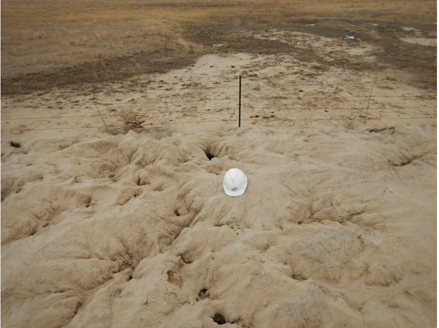
Figure 23: Photo taken from east end of pit location facing east. Photo shows stormwater erosion on pit's containment berm and sediment deposition off the site.
