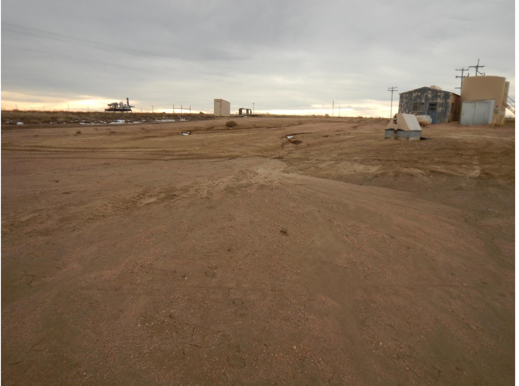
Figure 5: Photo taken from north end of location facing southwest. Photo shows surface erosion on location and insufficient stormwater BMPs.
