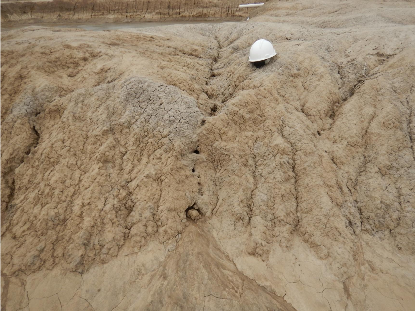
Figure 27: Photo taken from west end of pit location . Photo shows stormwater erosion on pit's containment berm. Stormwater flow occurring on surface, as well as the subsurface of the berm
