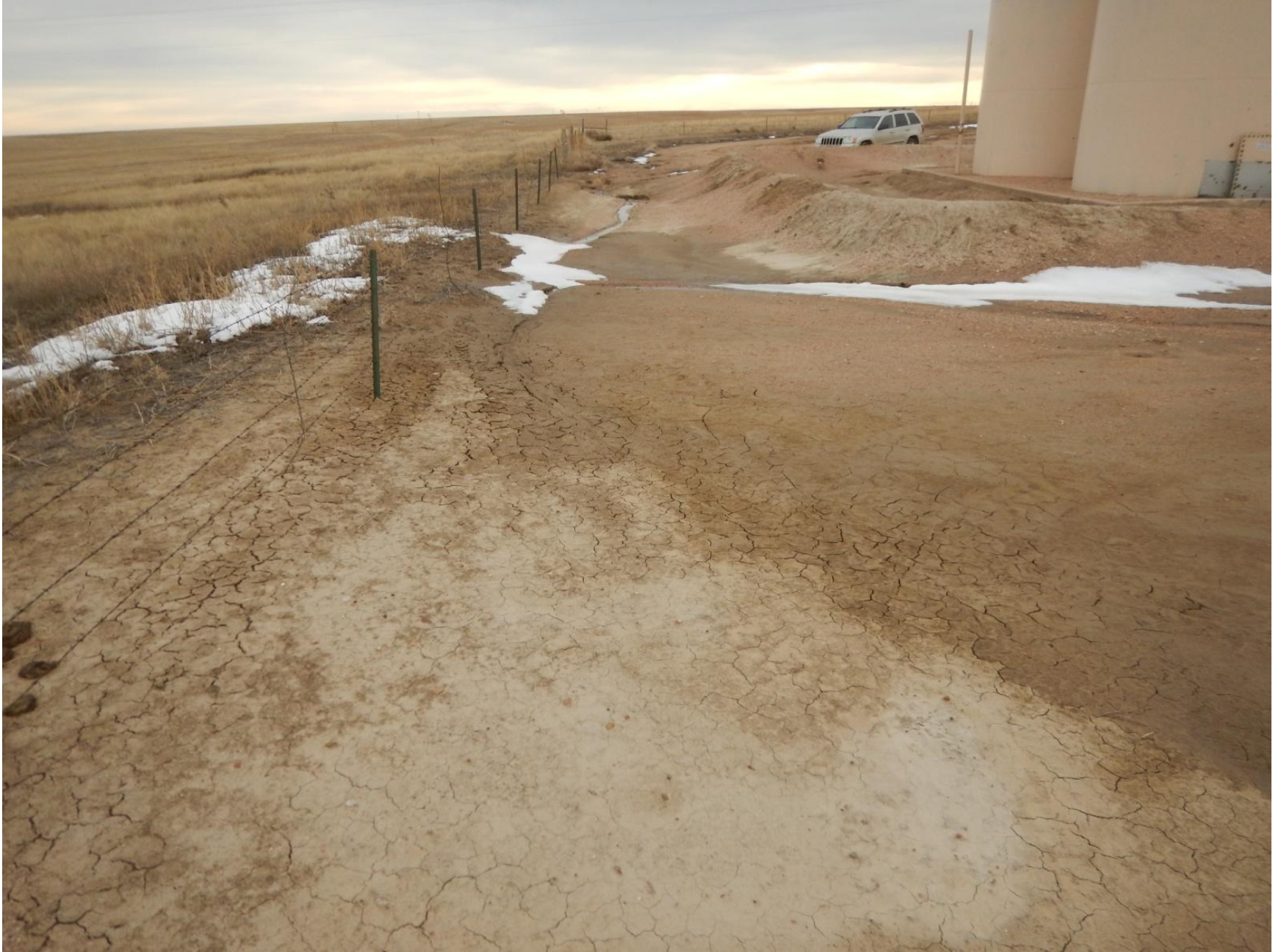
Figure 4: Photo taken from northeast end of location facing south. Photo shows surface erosion on location and insufficient stormwater BMPs.
