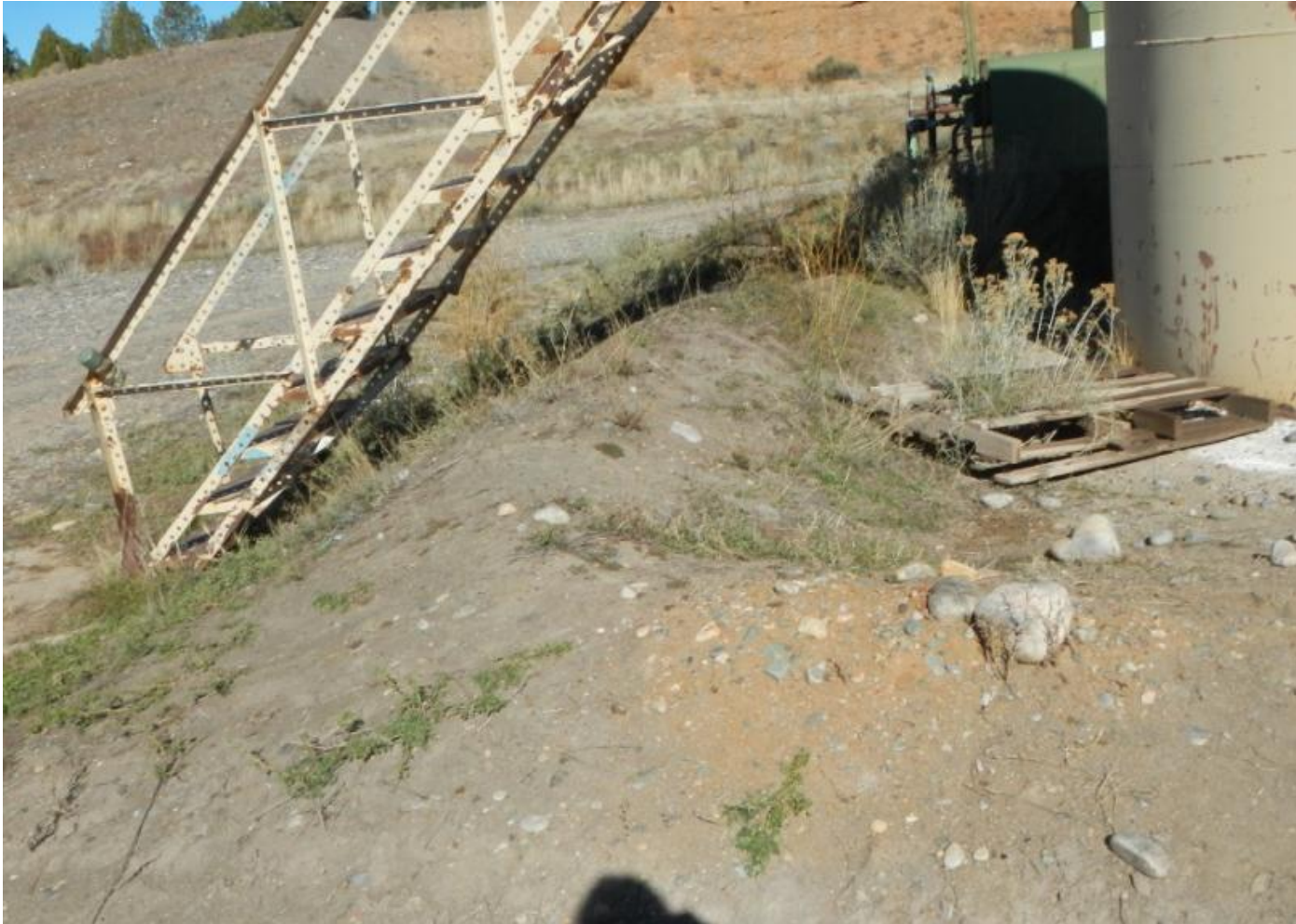
Photo 5. View of weeds and debris within tank berm area.
