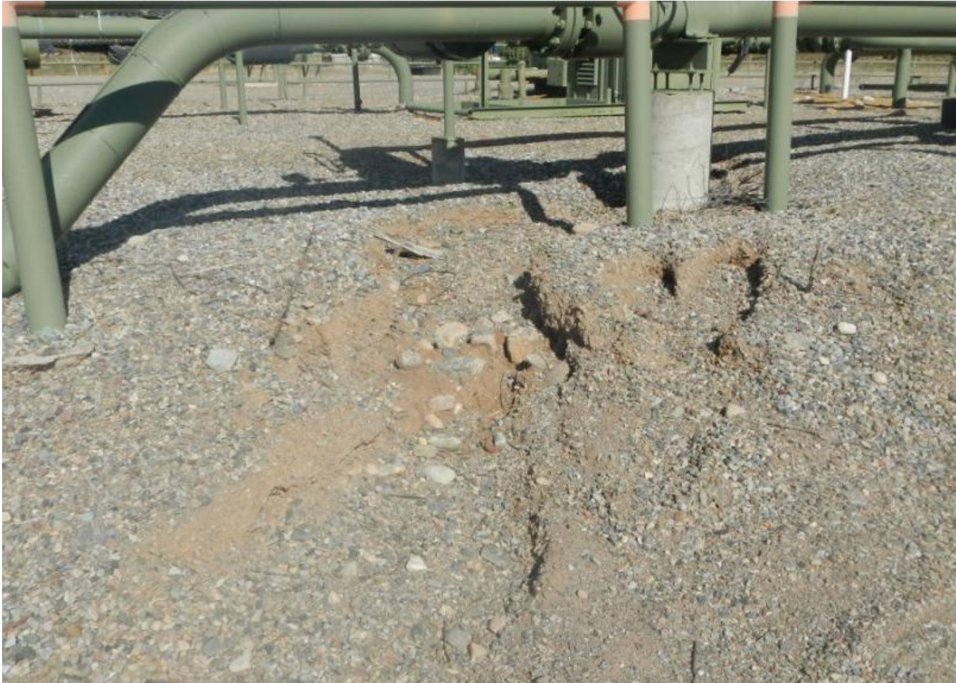
Photo 4. View of erosion in southern portion of project area that appears to be eroding off of facilities area. This should be monitored and repaired if it worsens.
