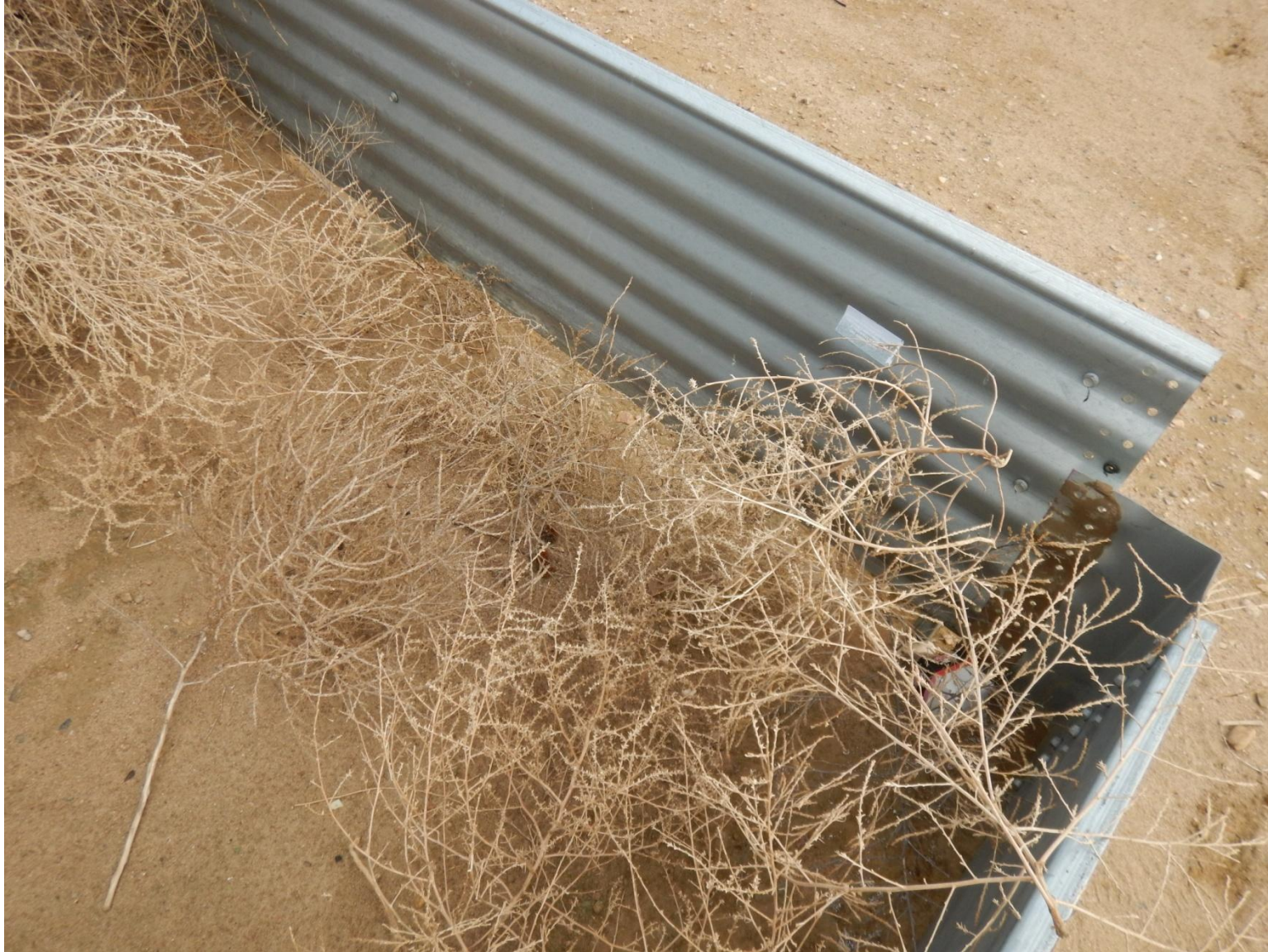
Photo 6: Photo taken from eastern part of location. Photo of panel surrounding equipment in disrepair and weed debris.
