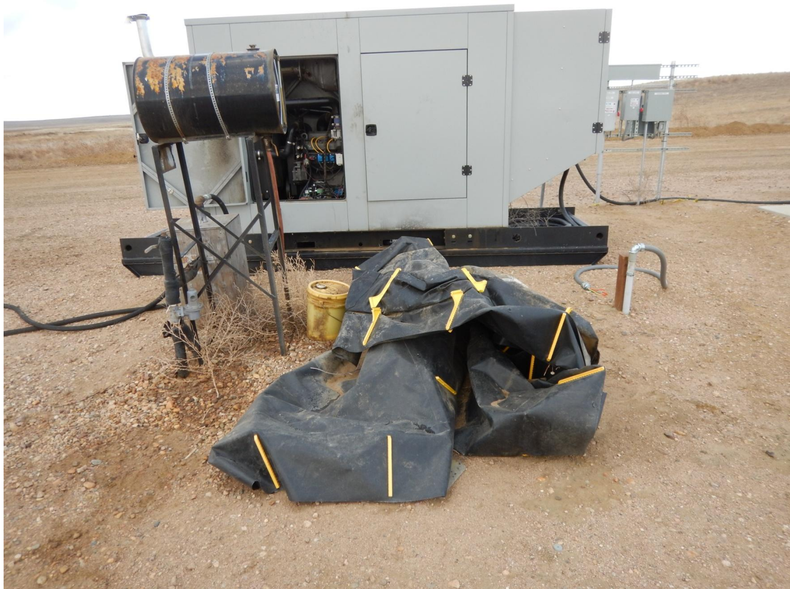
Photo 11: Photo taken from western part of location. Photo of weed debris in equipment, and trash debris. Trash debris appears to be a black tarp. Stained soil evident on ground below equipment.
