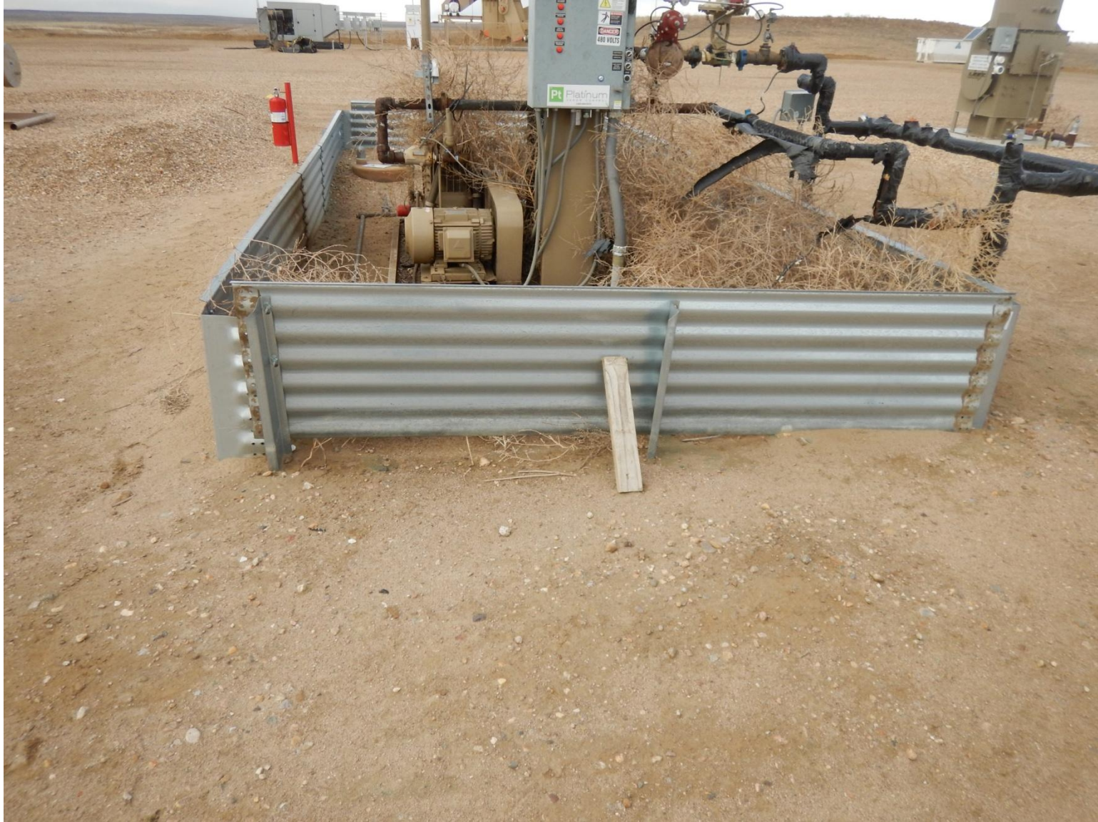
Photo 5: Photo taken from eastern part of location. Photo of panel surrounding equipment in disrepair and weed debris.
