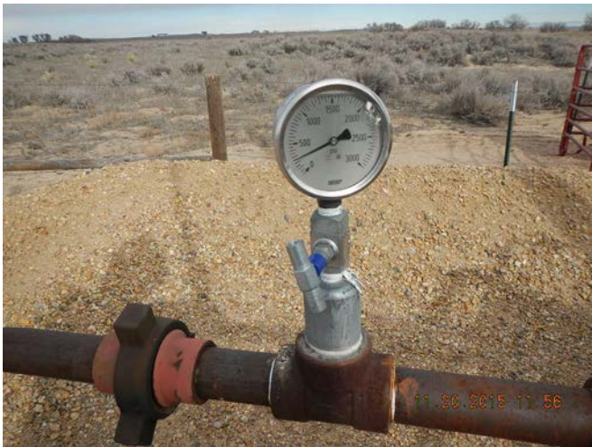
Initial well site flowline gauge reading.
