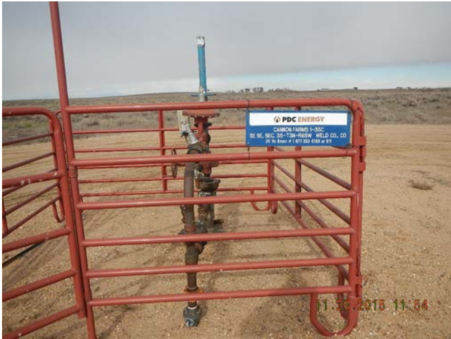
Cannon Farms 1-35C Wellhead – starting point of well site flowline.
