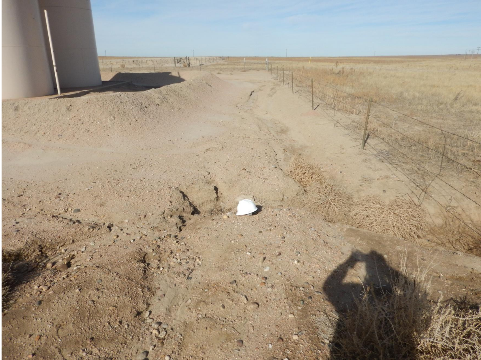
Photo 14: Photo taken from east end of location facing north. Photo shows confluence of storm water erosion channels from northern and southern halves of location.
