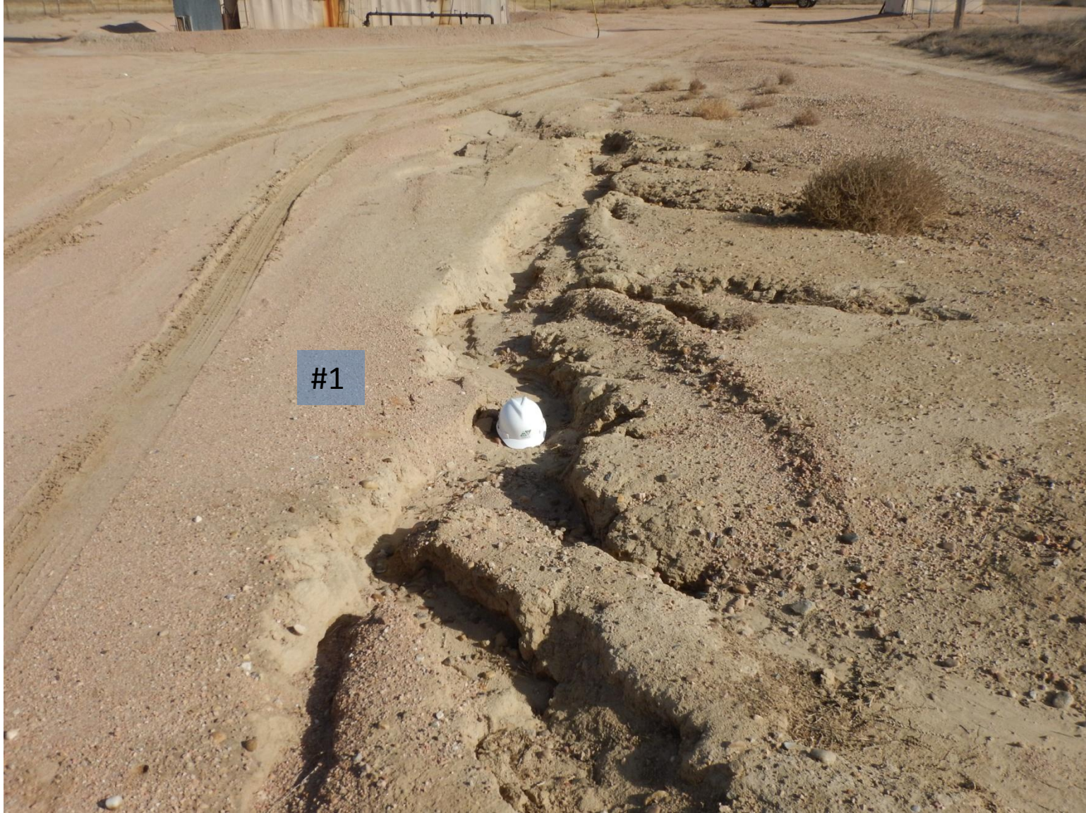
Photo 5: Photo taken from southern end of location, facing east. Note the rill erosion forming stormwater erosion channel #1.
