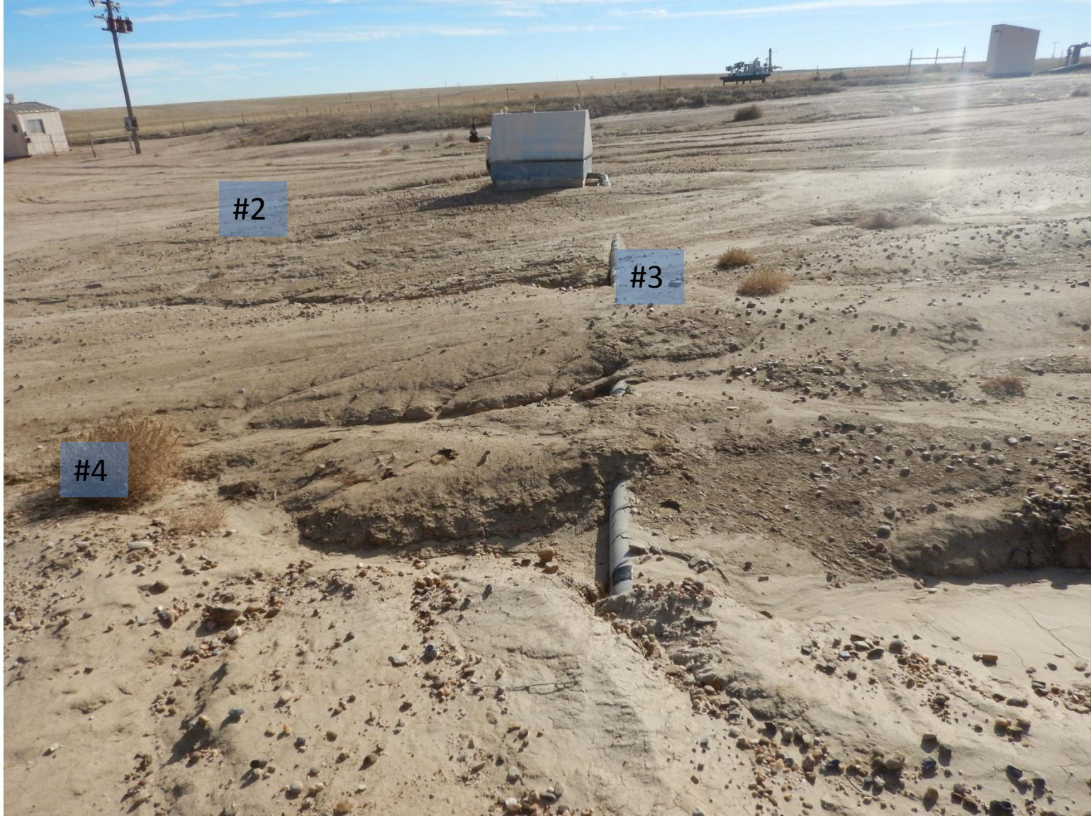
Photo 9: Photo taken from north end of location facing south. Photo of exposed pipe and stormwater erosion.
