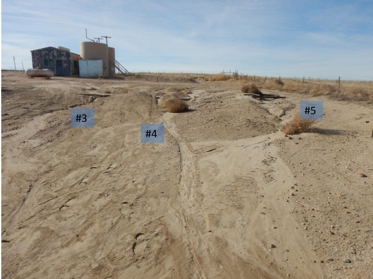
Photo 11: Photo taken from northern end of location facing west. Photo of stormwater erosion channels #3, #4, and #5 on northern half of location.
