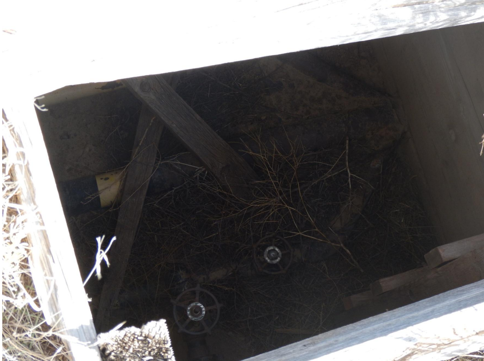
Photo 7: Photo of pipe and valves within exposed wooden sub-surface structure. This poses a hazard to wildlife and human safety.
