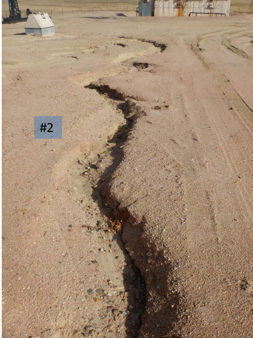
Photo 8: Photo taken from southwestern end of location facing east. Note erosion forming stormwater erosion channel #2.
