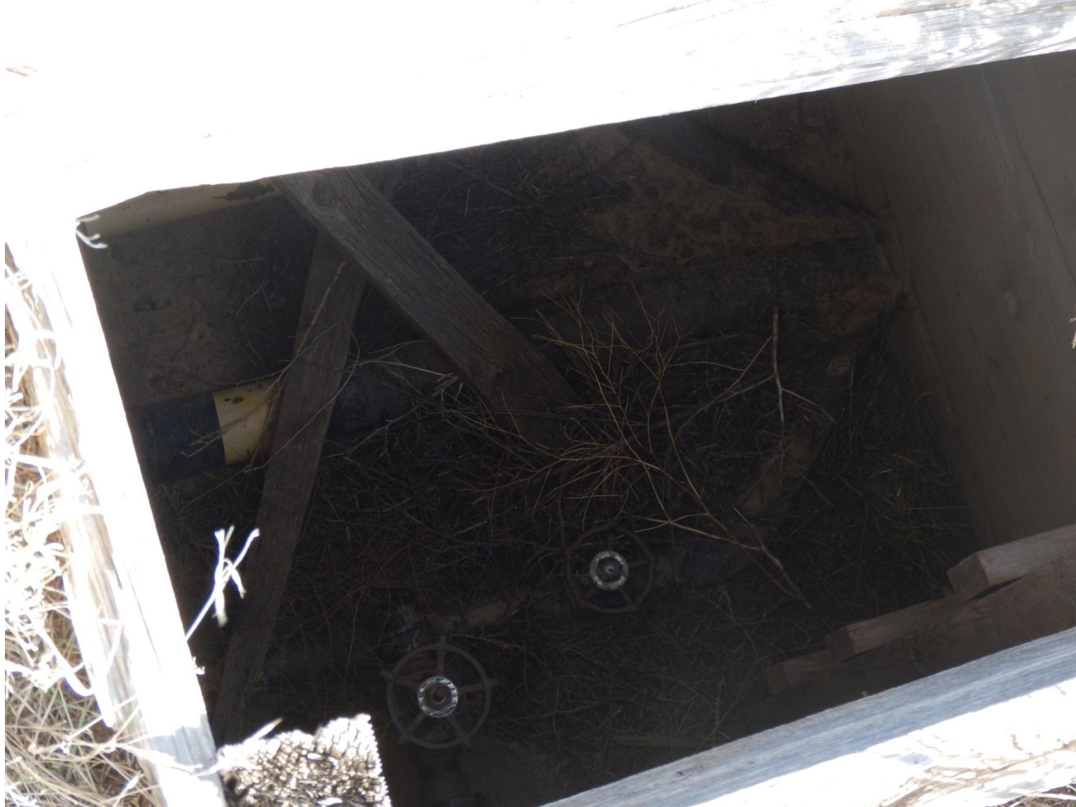
Photo 7: Photo of pipe and valves within exposed wooden sub-surface structure. This poses a hazard to wildlife and human safety.
