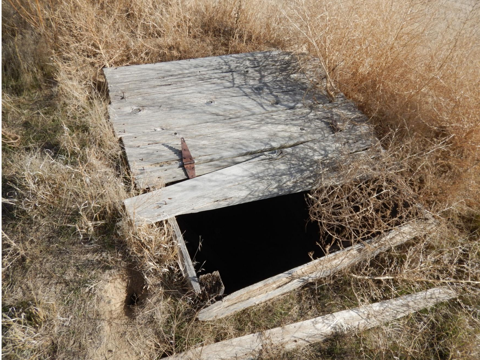
Photo 6: Photo taken from northwestern end of location. Photo of exposed wooden sub-surface structure.
