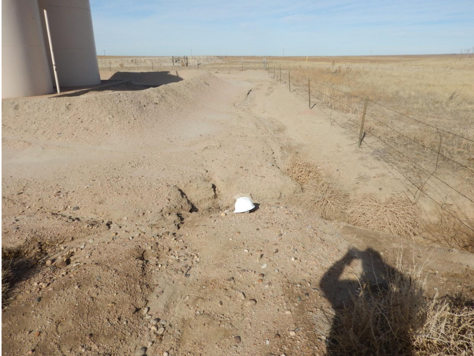
Photo 14: Photo taken from east end of location facing north. Photo shows confluence of storm water erosion channels from northern and southern halves of location.
