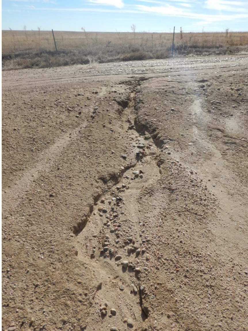
Photo 3: Photo taken on southern end of location. Photo of rill erosion.
