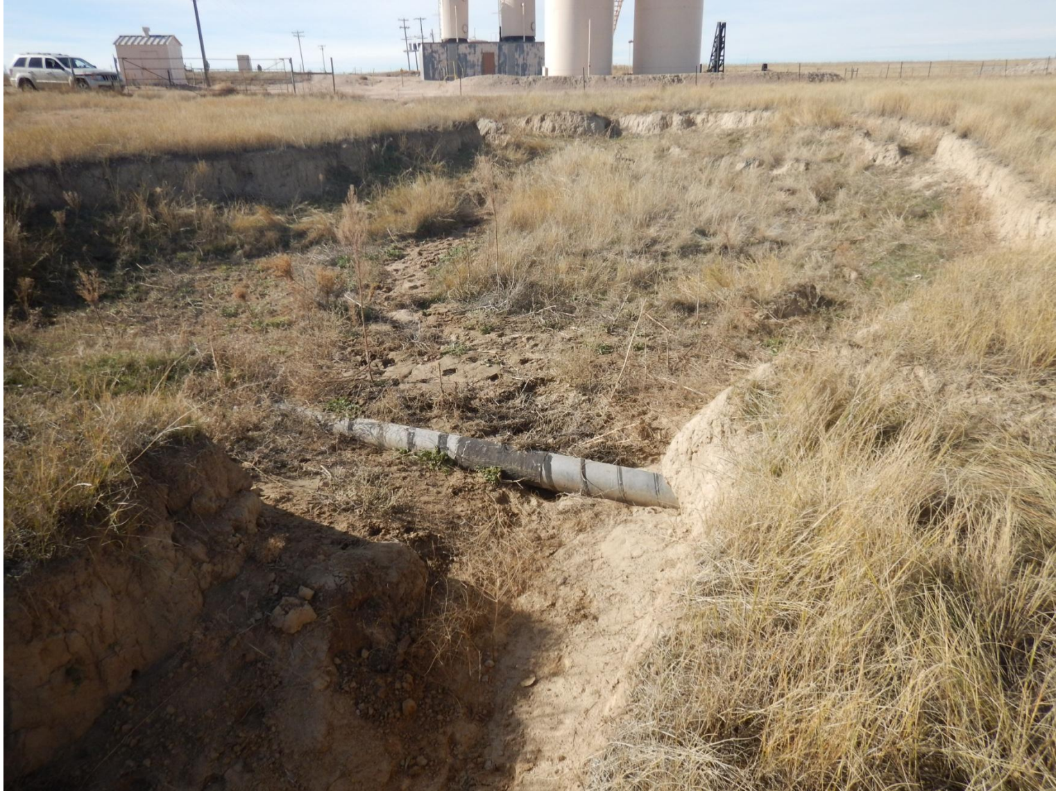
Photo 20: Photo taken east of location facing west towards location. Photo of exposed pipeline.
