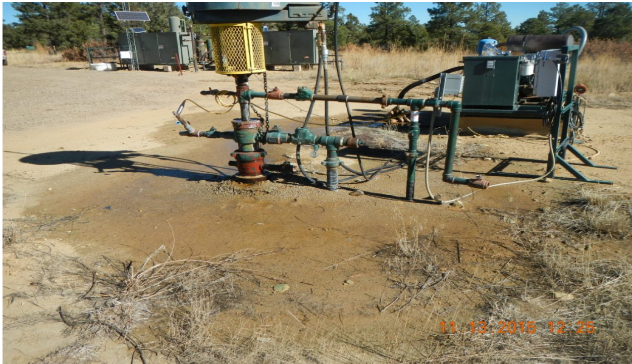
photo 3: Water leak is dripping out of the well head.
