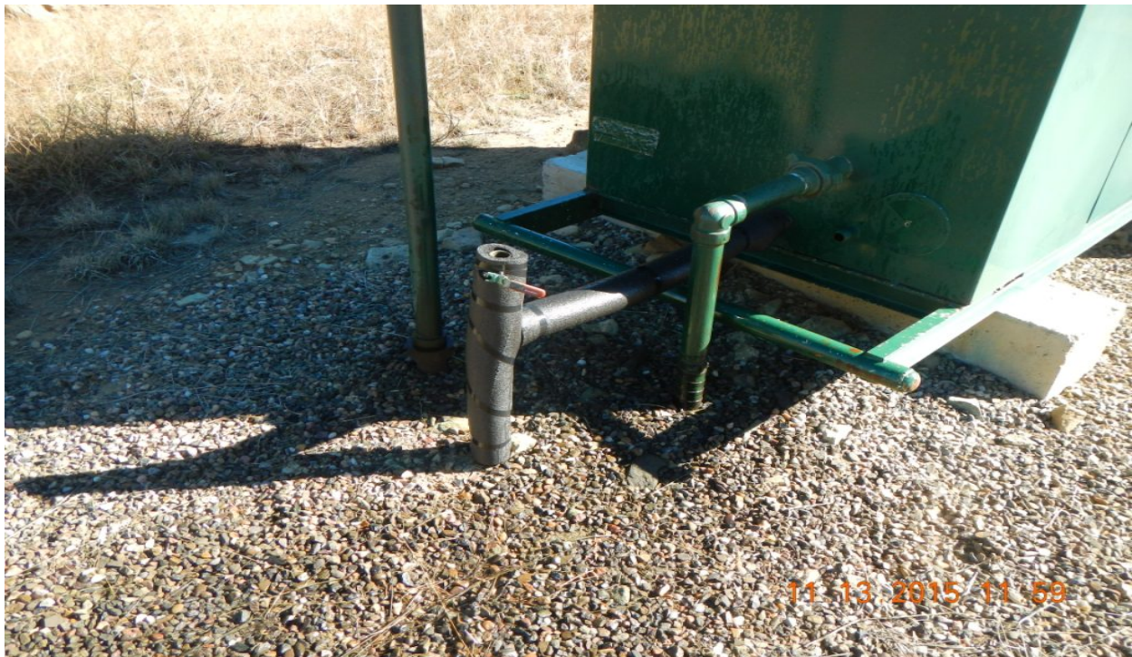
photo 6: Point where fluid may have been released from.
