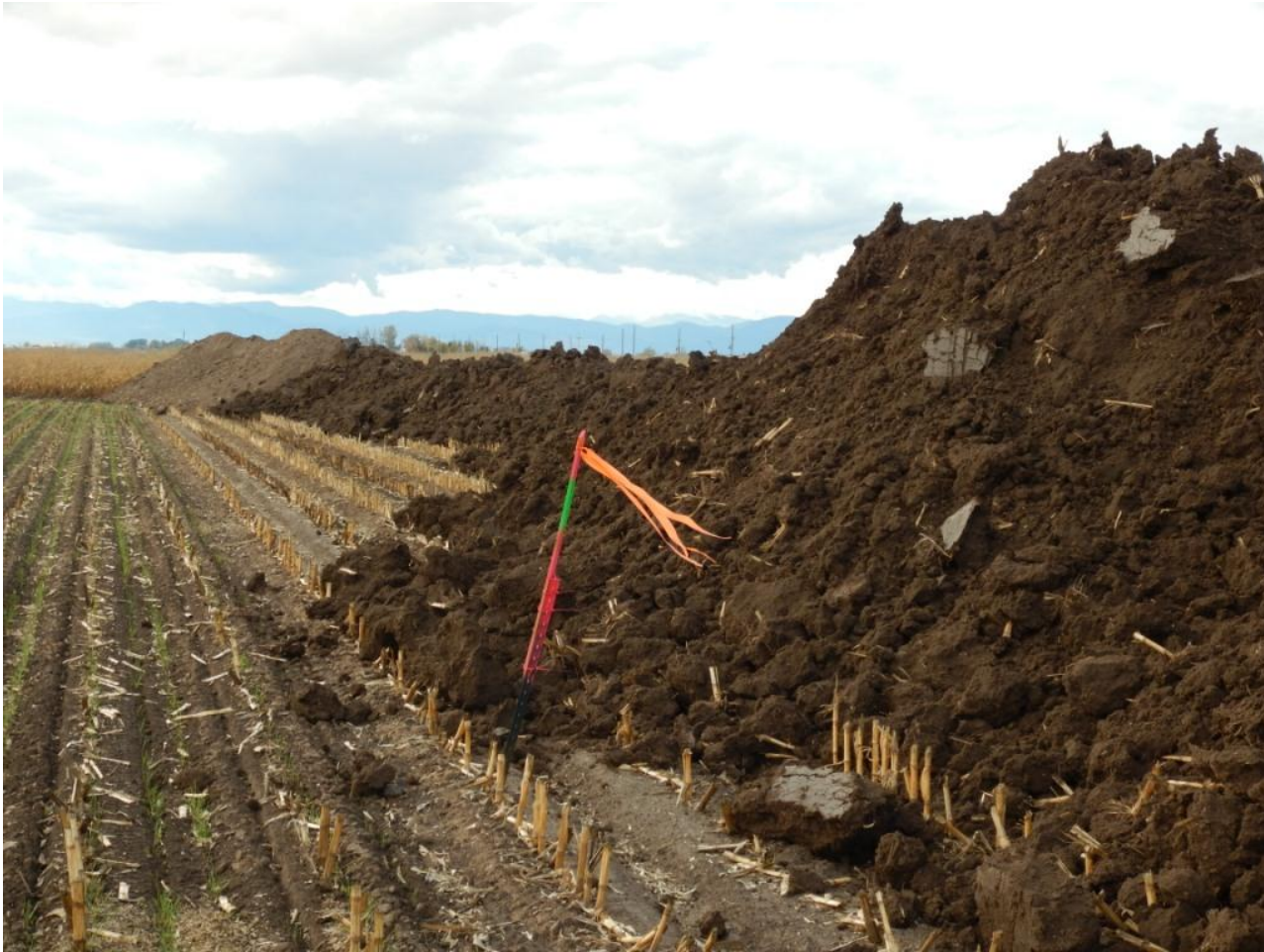
Photo 6. Photo taken of southern topsoil stockpile, facing Northwest. Need to stabilize topsoil stockpile. Topsoil salvage process was not complete during this inspection.
