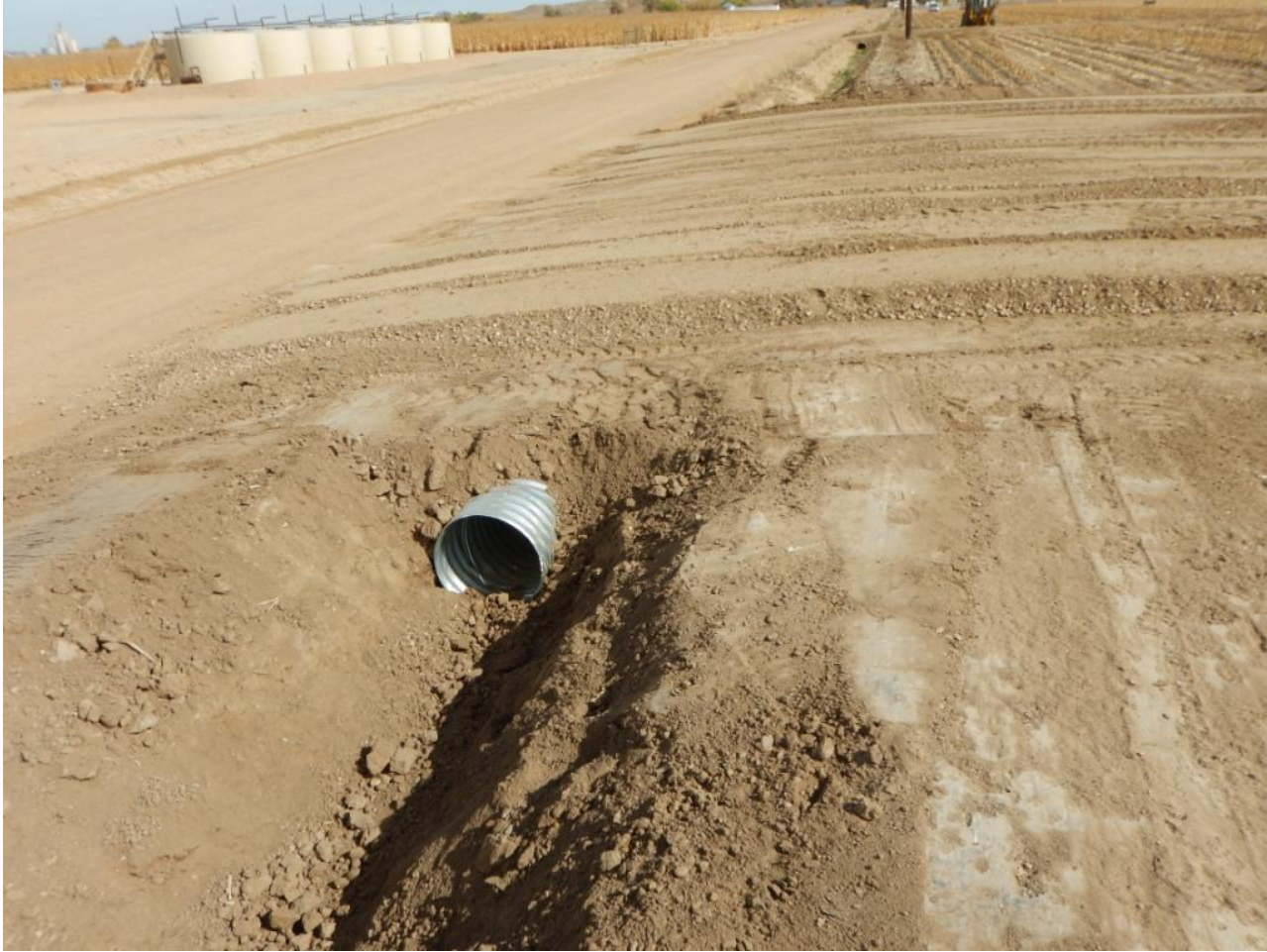
Photo 4. Photo taken of west, northern access road, facing East. Stormwater control ditch with culvert in center of photo.
