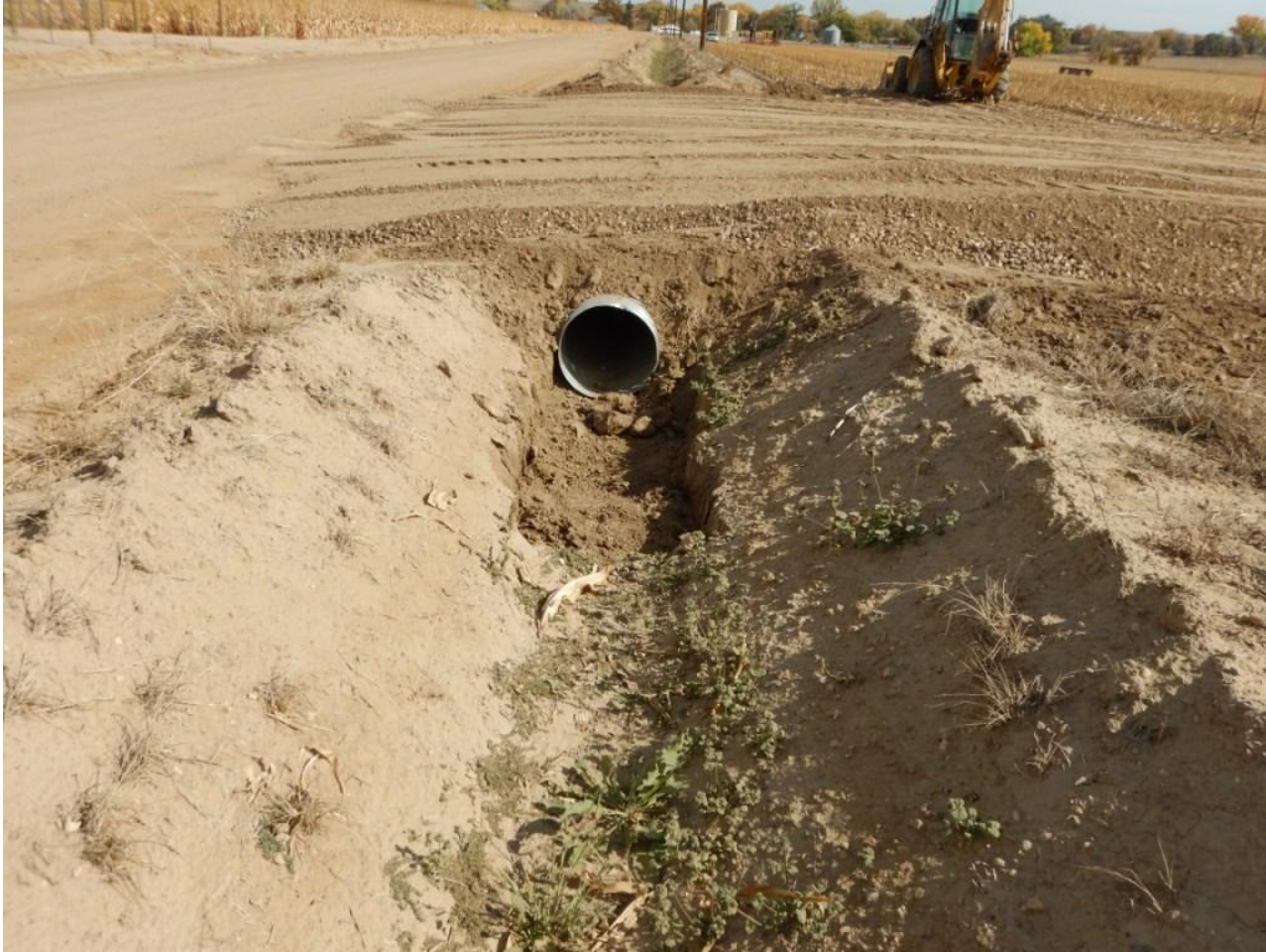
Photo 2. Photo taken of east, northern access road, facing East. Stormwater control ditch with culvert in center of photo.
