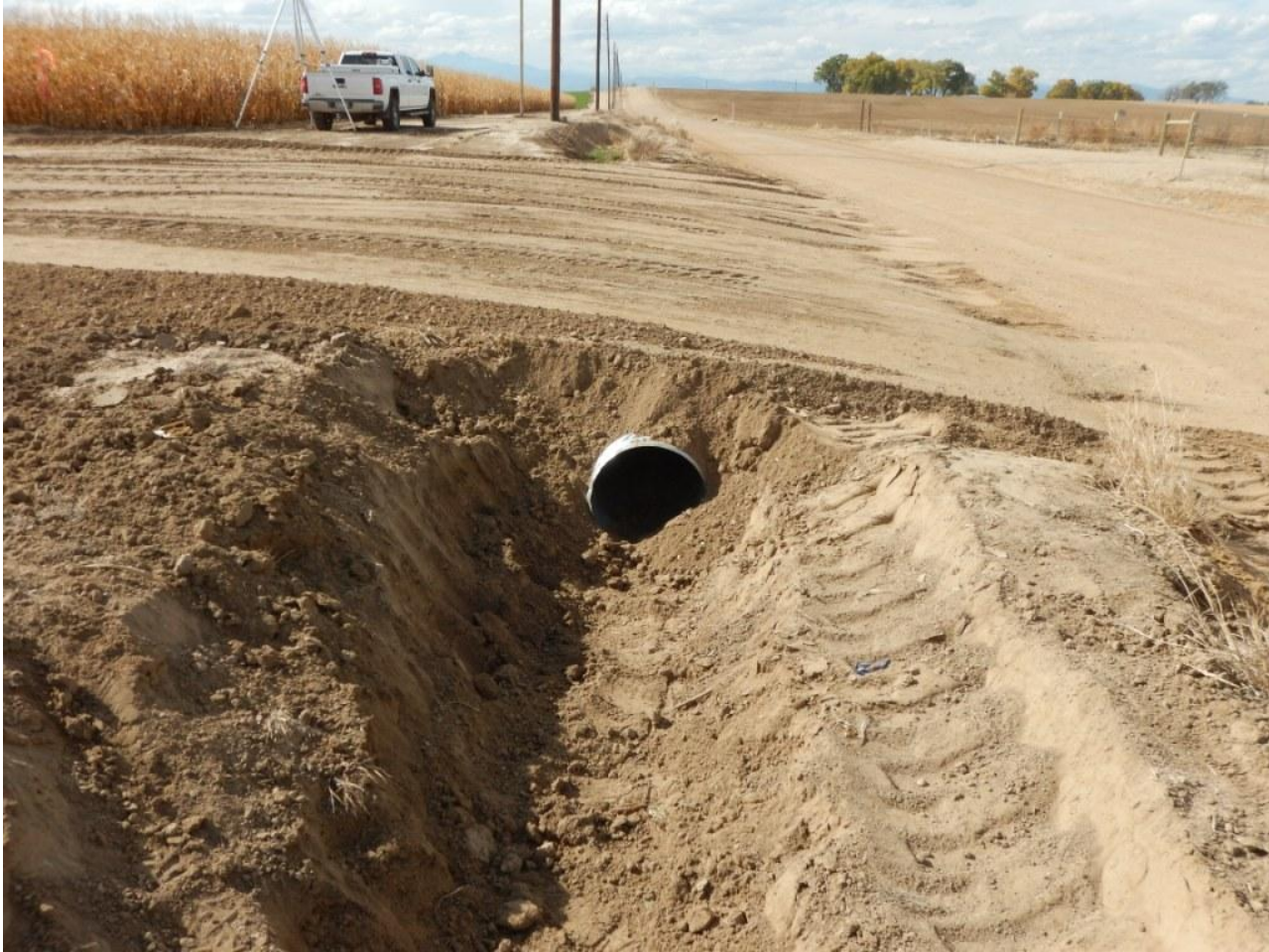
Photo 3. Photo taken of west, northern access road, facing West. Stormwater control ditch with culvert in center of photo.
