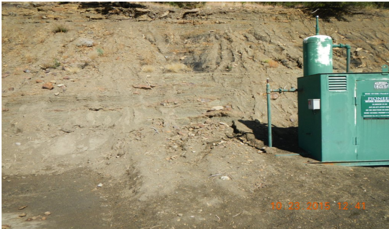
photo 4: Erosion is occurring along the north side of the location.
