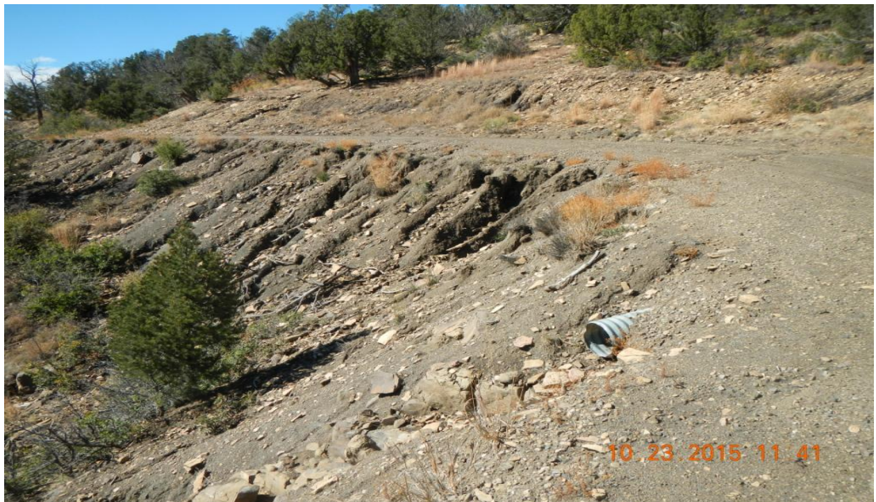
photo 2: Facing west. Erosion occurring along the access road near the location.
