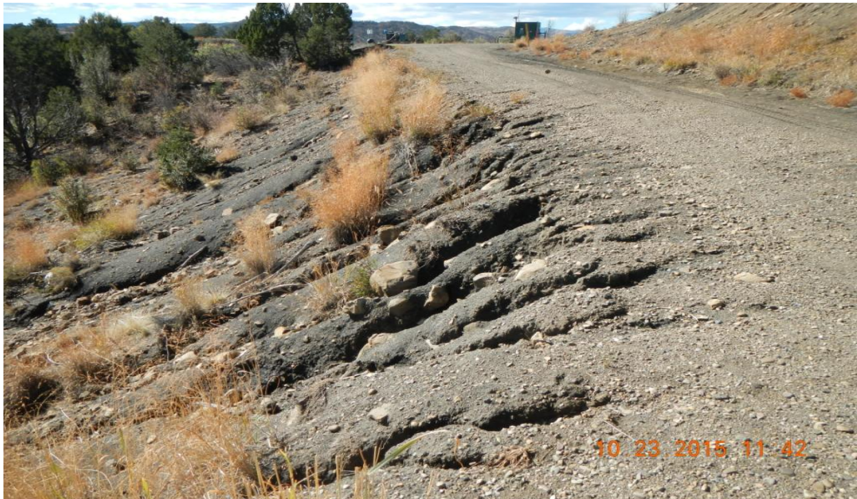
photo 3: Facing southwest. Erosion occurring along the access road near the location.
