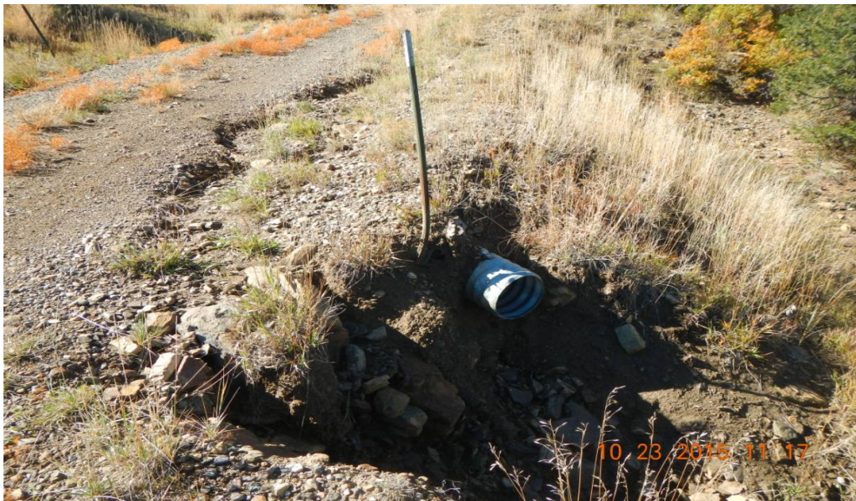
photo 4: Access road is eroding around the culvert.
