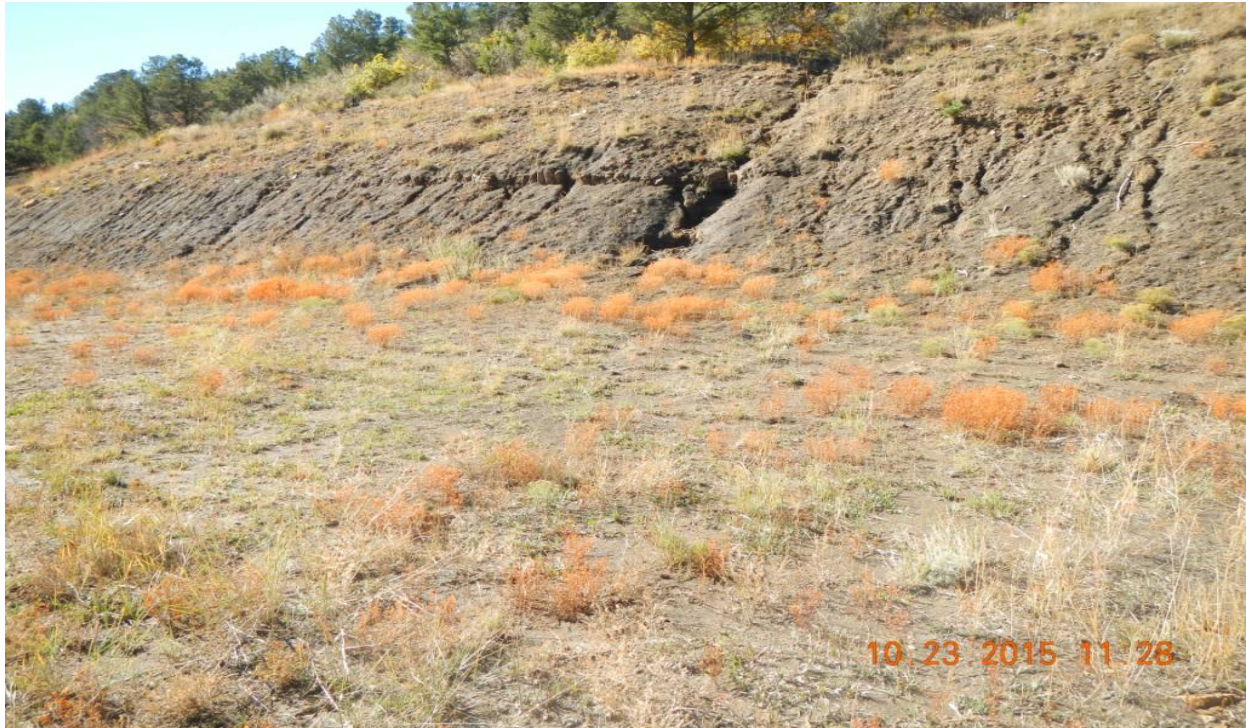
photo 11: Center of the location facing southwest. Erosion occurring along west side of the pad.
