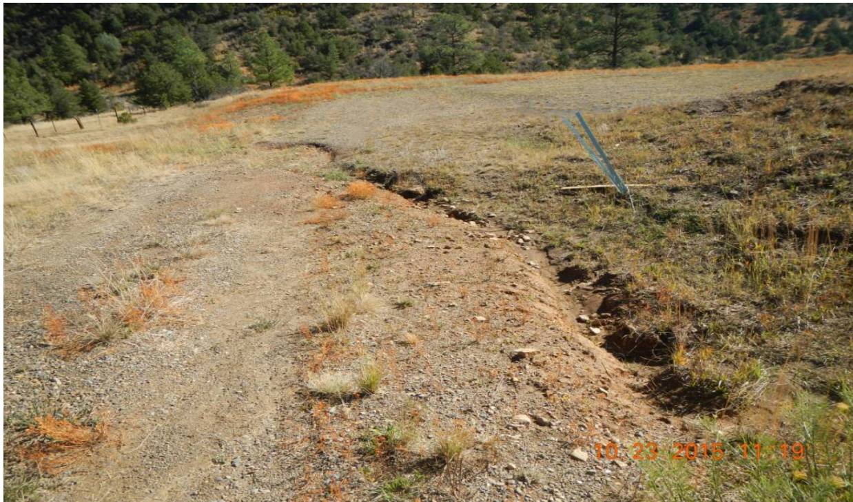
photo 8: Erosion occurring along the access road near the location.
