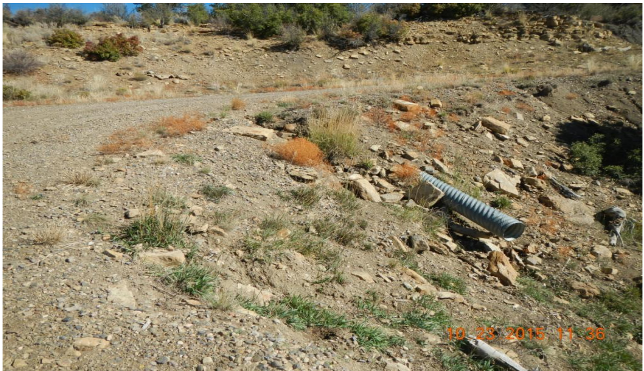
photo 2: Access road towards the location has not been reclaimed and culverts remain in place.
