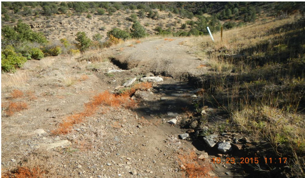
photo 6: Erosion is occurring across the road which is making the road inaccessible.
