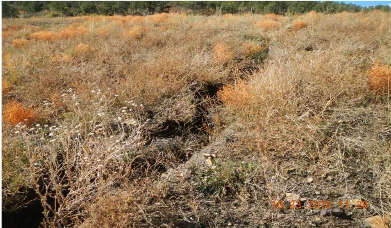
photo 15: East side of the pad. Erosion channel is transporting sediment off the location.
