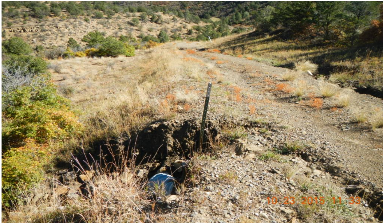
photo 3: Facing east along access road. Access road is eroding around the culvert.
