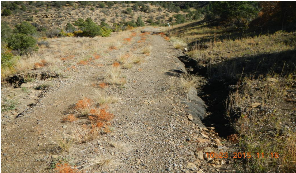
photo 5: Facing east along access road. Erosion is occurring on and along the side of the access road.
