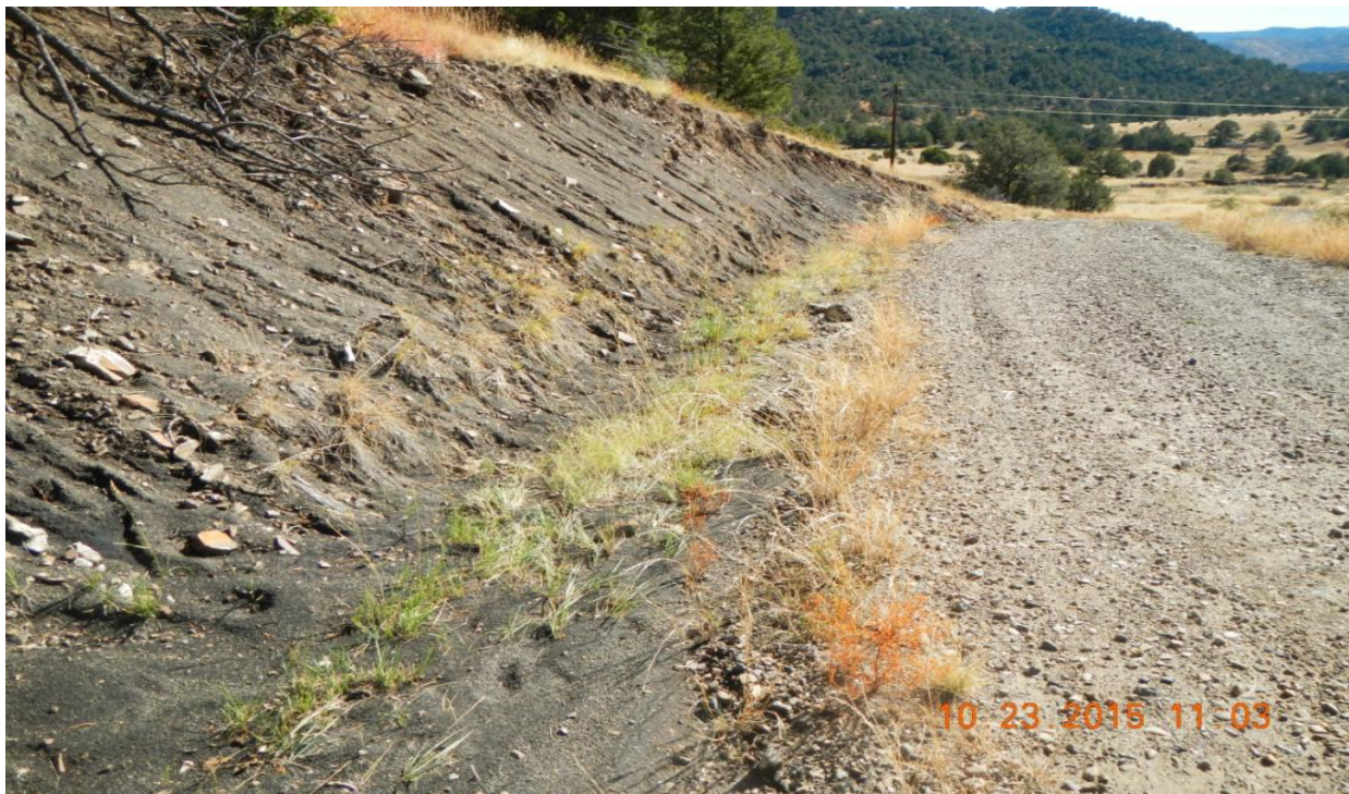
photo 6: Side of the access road is not well stabilized.
